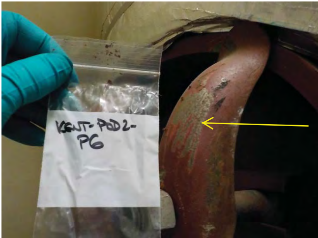
Photograph 13: Non-lead containing red paint (Sample P6) on piping of hot water storage tank in Boiler Room.
