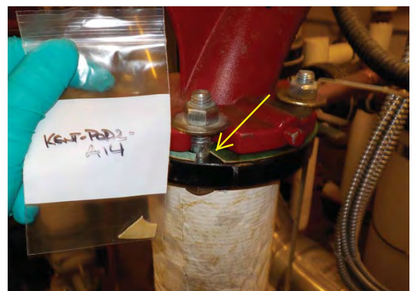
Photograph 12: Typical non-asbestos gasket (Sample A14) located on boiler piping in Boiler Room.
