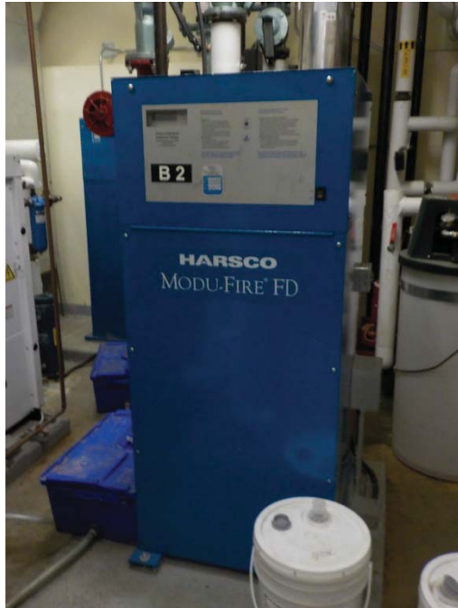
Photograph 9: Boiler number 2 (of 2 boilers) located in the Boiler Room.
