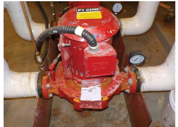
Photograph 14: Non-lead containing red paint (Sample P8) on pump labelled P1CHW in Boiler Room.
