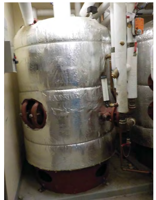
Photograph 8: Hot water storage tank in Boiler Room.
