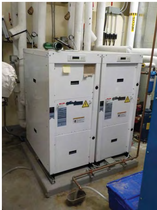
Photograph 3: The two heat exchangers located in the boiler room. The unit on the right is the active unit, containing R410a.
