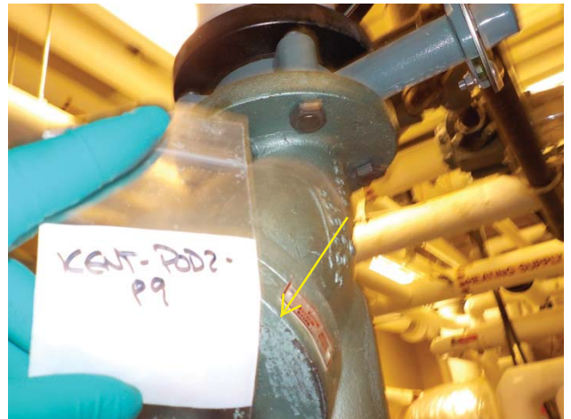
Photograph 2: Lead-containing teal green paint on a valve assembly associated with one of the two boiler units. Both boiler units have a valve assembly with lead-containing teal green paint.
