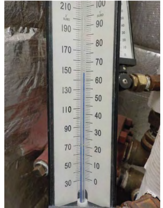
Photograph 10: Typical non-mercury temperature gauge on equipment in Boiler Room.
