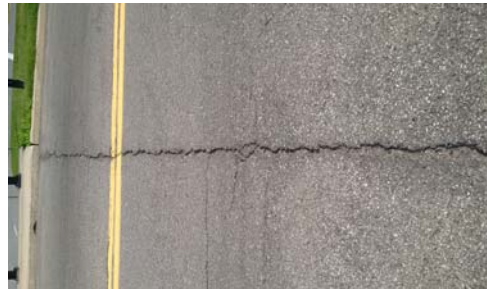
High-Severity longitudinal and transversal cracking to be sealed
