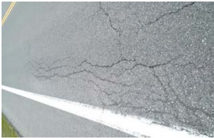
High-Severity Alligator Cracking to be sealed
