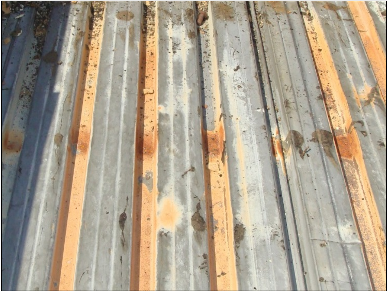
Photo of Level 2: Light to Moderate Corrosion
