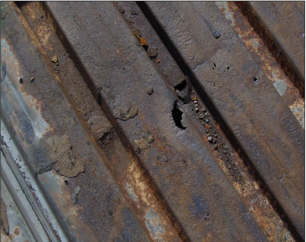
Photo of Level 4: Severe Corrosion With Holes
