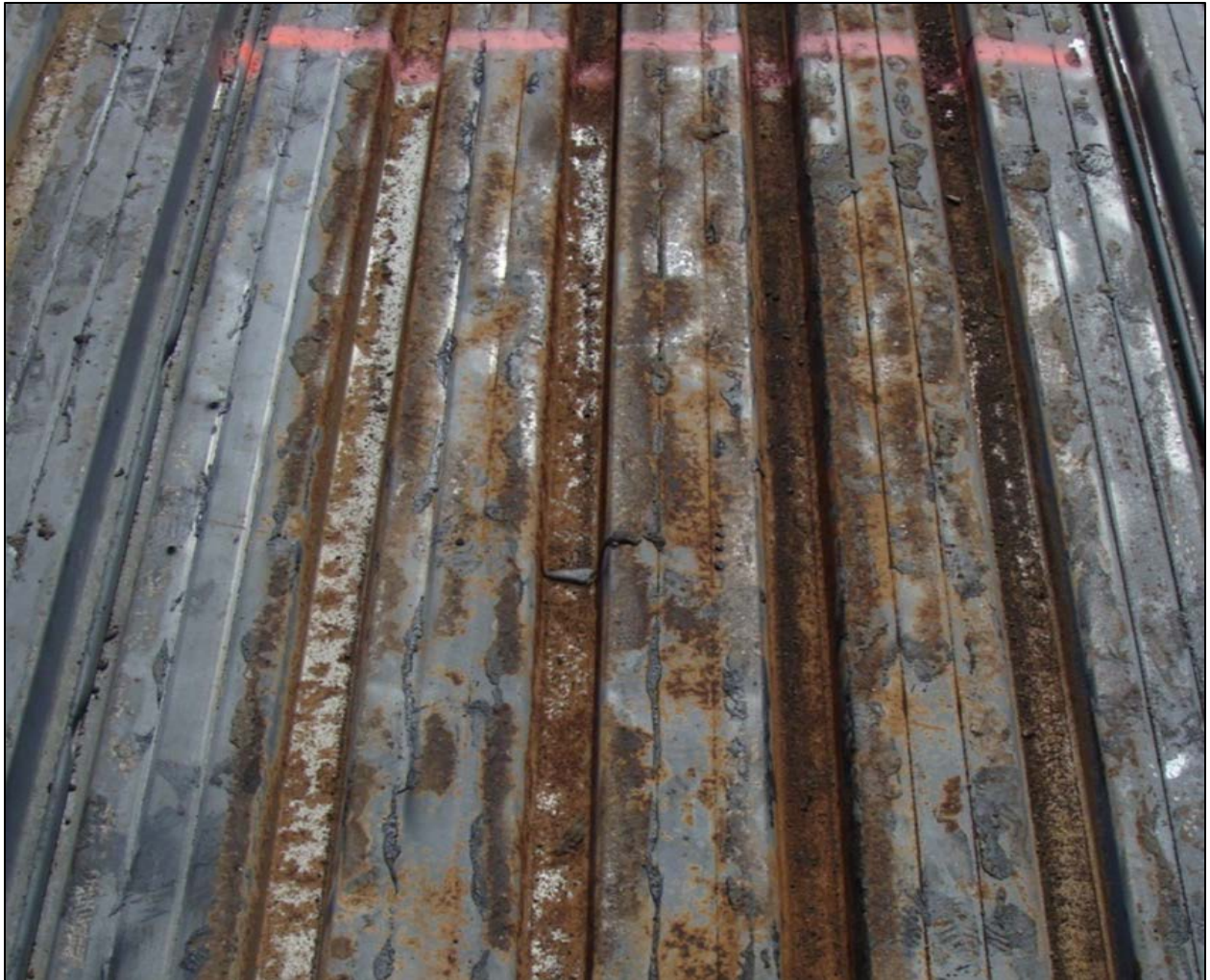
Photo of Level 3: Severe Corrosion, No Holes, or Penetrations
