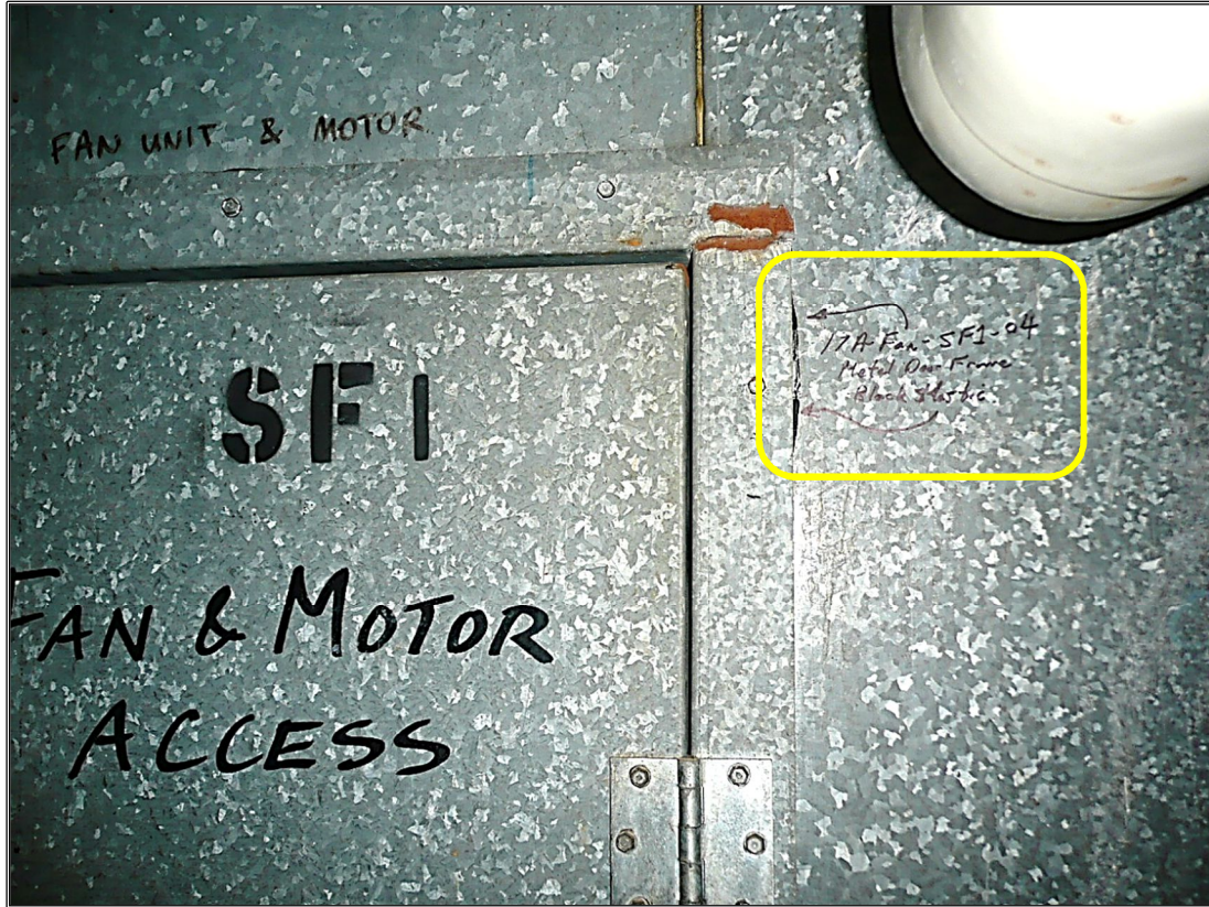
The Black Mastic from under the door edge as sampled and observed on the Exterior Supply Fan SFI Upper Right Door Frame 5th Door to the South was found to be None Detected for asbestos.
