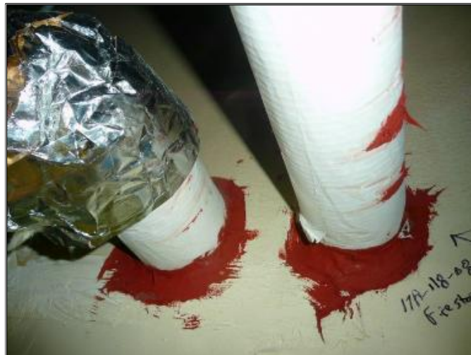
Green Duct Mastic and Red Fire Stop as sampled were found to be None Detect for asbestos.
