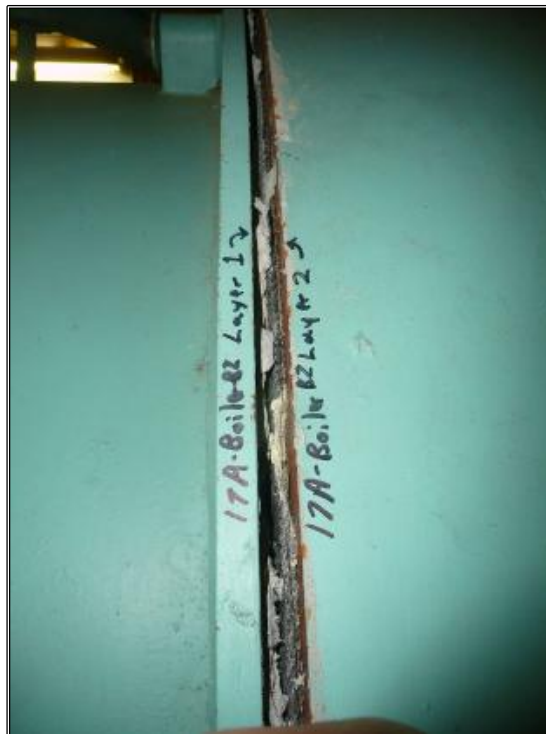
The North End Layered Packing and Gasket associated as observed and sampled on the north end of Boiler B2 in Room 144 Mechanical was found to be None Detected for asbestos.
