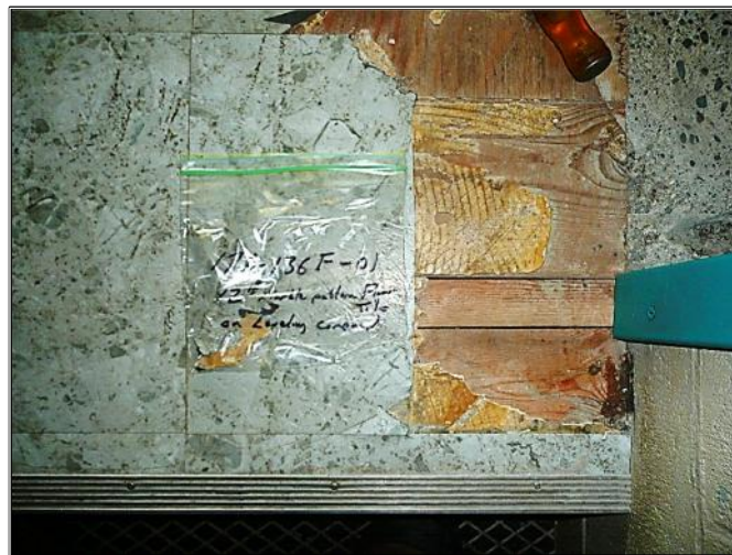
Floor Tile and Vinyl Sheet Flooring as sampled were found to be None Detect for asbestos.
