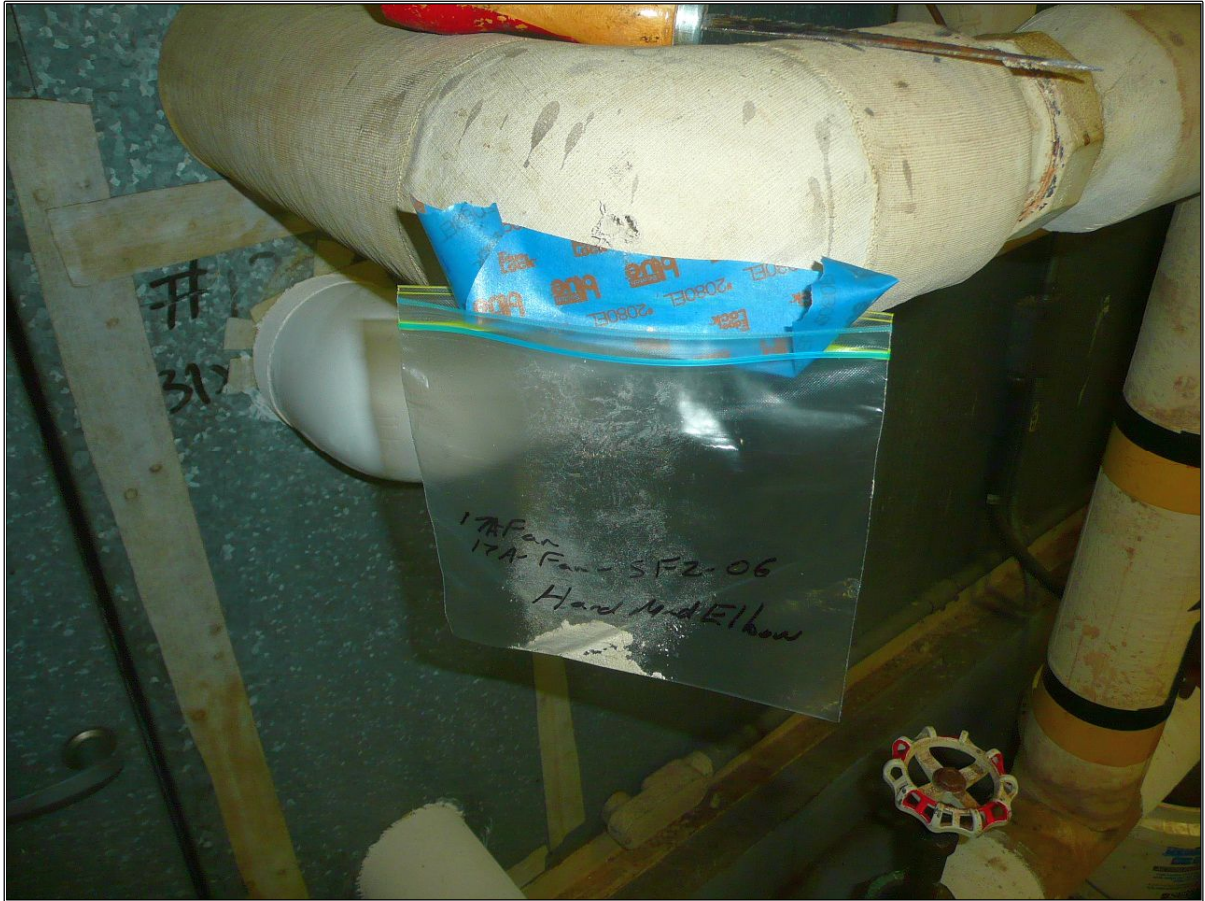
The Thermal Pipe Insulation Hard Mud Elbow as sampled and observed on the North Supply Fan SF2, near 2nd Door to the West was found to be None Detected for asbestos.
