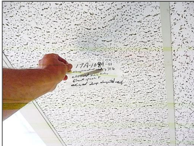
Suspended Ceiling Tiles as sampled were found to be None Detect for asbestos.
