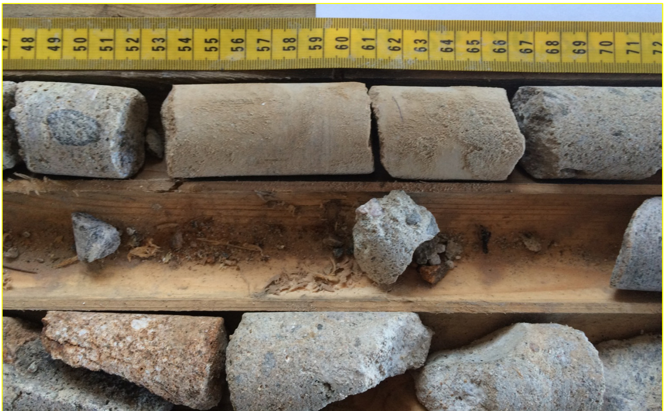
DH15-3 detail showing very friable concrete and poor recovery sections.
