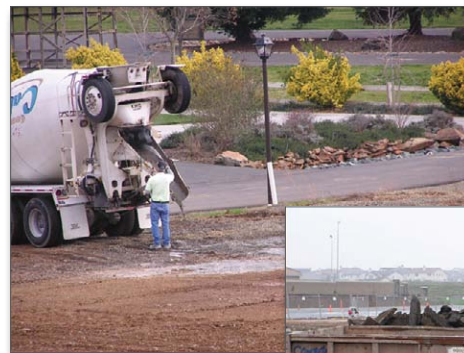
Figure 1. Chute washwater being dumped on the ground
