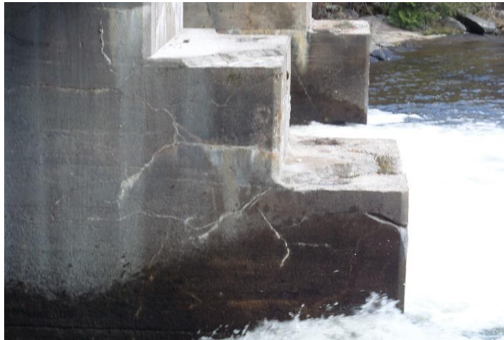
PHOTOGRAPH 3: Cracks on East Pier Stepping
