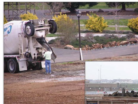
Figure 1. Chute washwater being dumped on the ground
