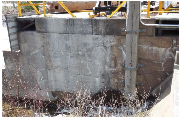
PHOTOGRAPH 2: Cracks on the East Pier
