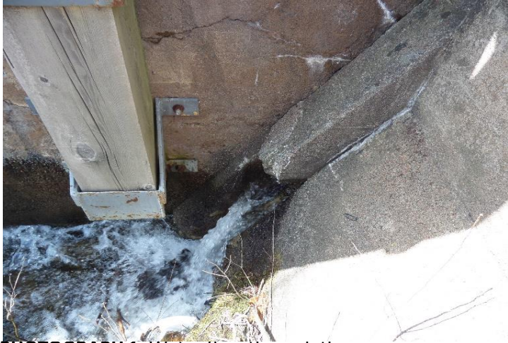
PHOTOGRAPH 1: Water flow through the Concrete Dam at East Pier
