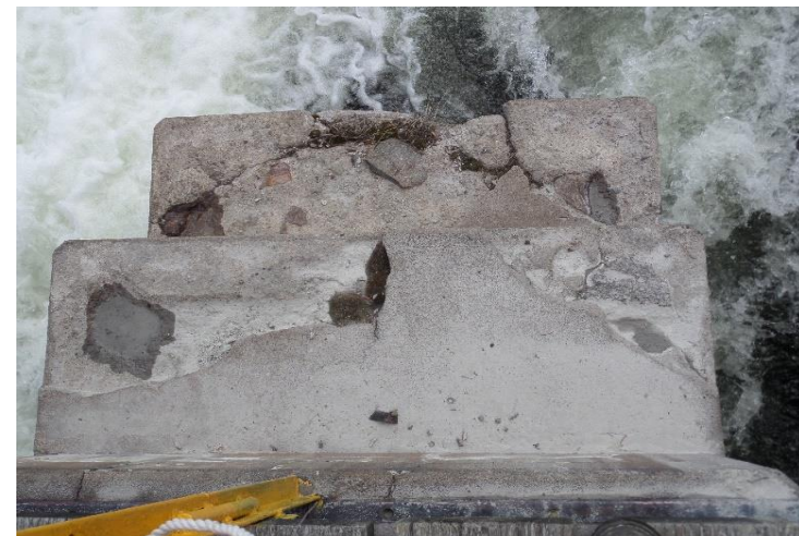
PHOTOGRAPH 4: Cracks on the Middle Pier
