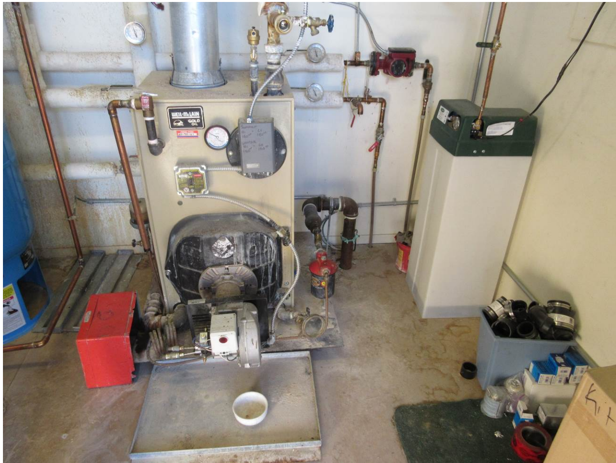
Photo 3 Mechanical Room Piping
