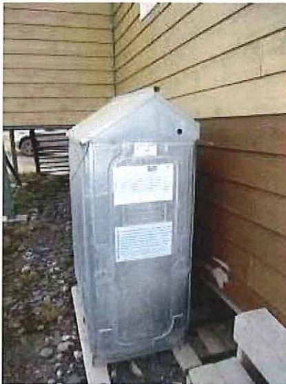
Photo 1: Outdoor above ground fuel tank
