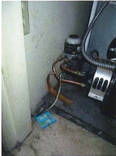
Photo 5: Indoor piping & accessories
