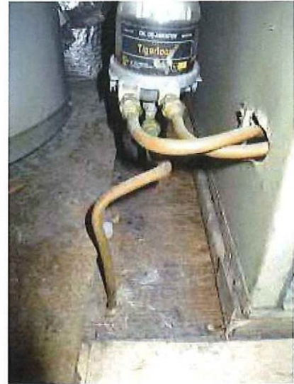
Photo 6: Indoor piping and accessories
