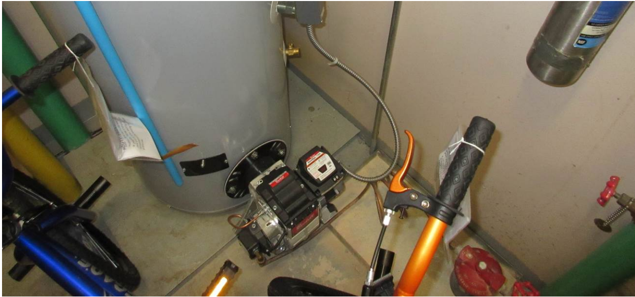
Photo 13 Hot Water Tank Fuel Piping
