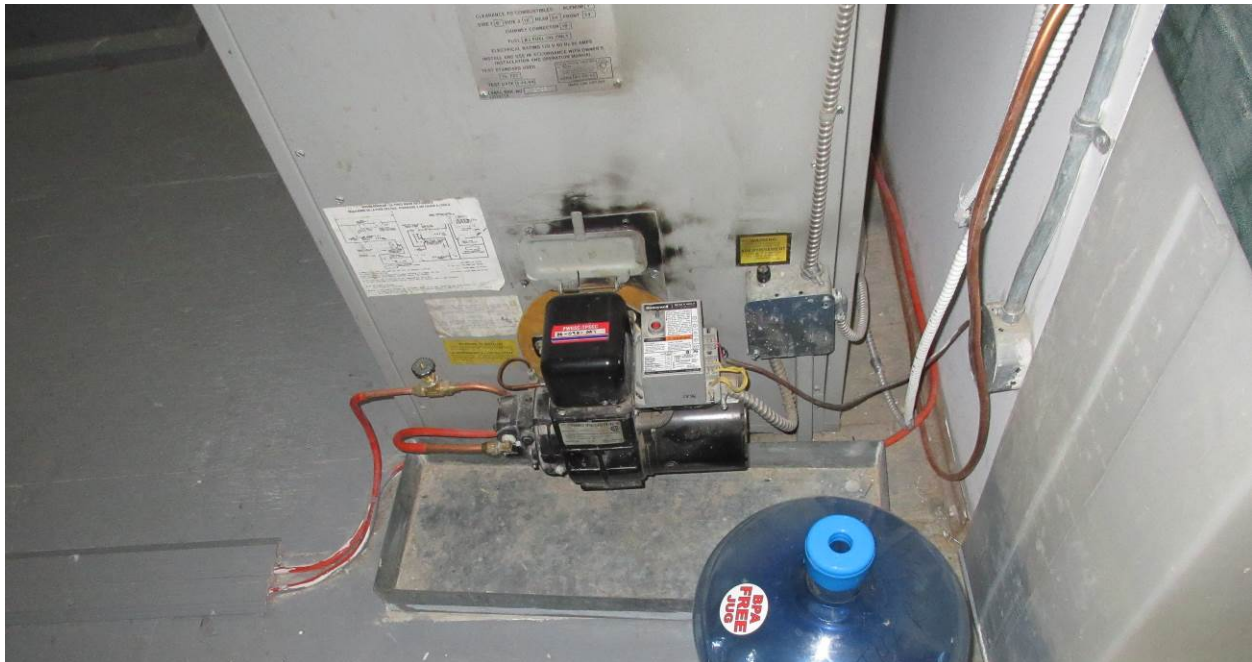
Photo 12 Fuel Lines at Furnace
