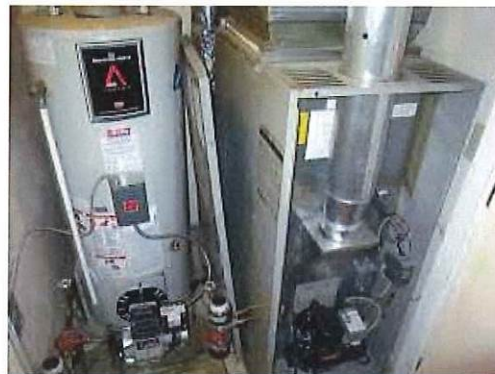
Photo 2: Interior furnace and water heater
