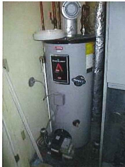
Photo 4: Indoor water heater
