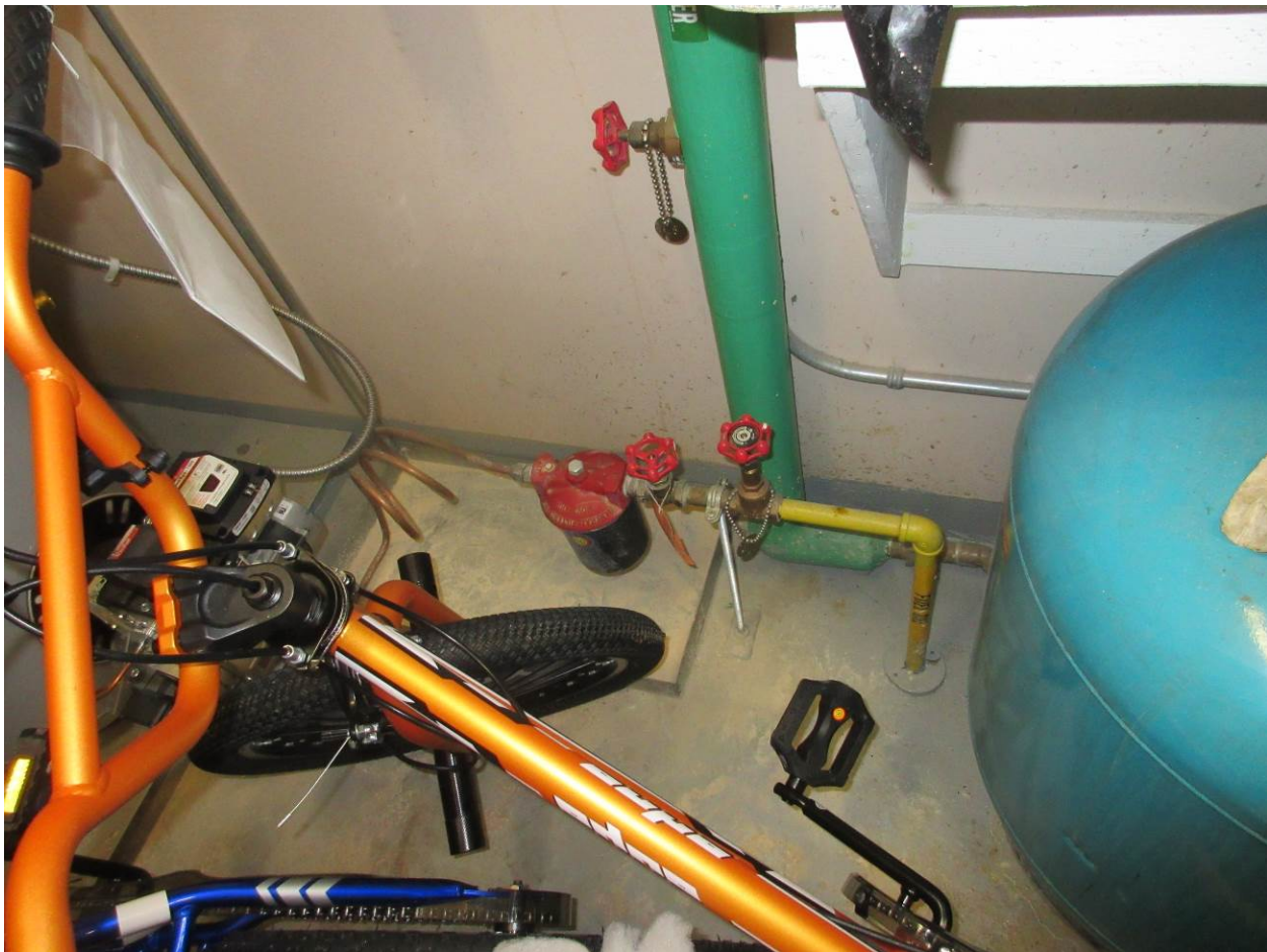
Photo 14 Hot Water Tank Fuel Piping
