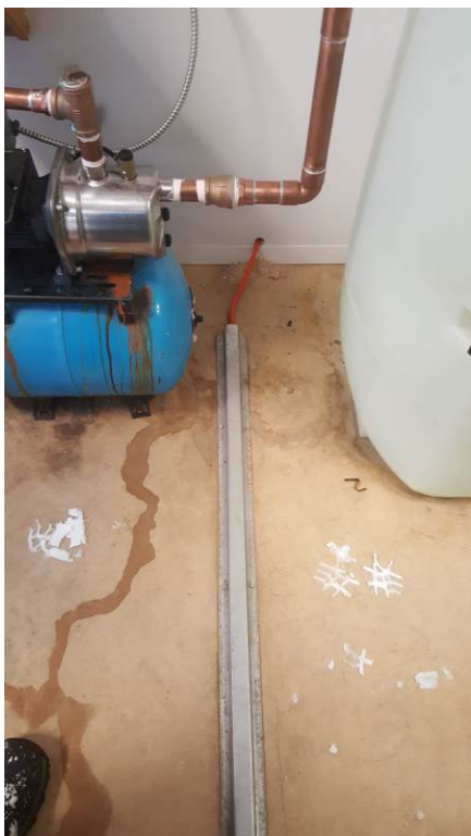
Photo 16 Interior Piping from exterior tank
