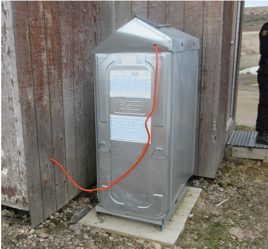
Photo 5 Existing Fuel Tank
