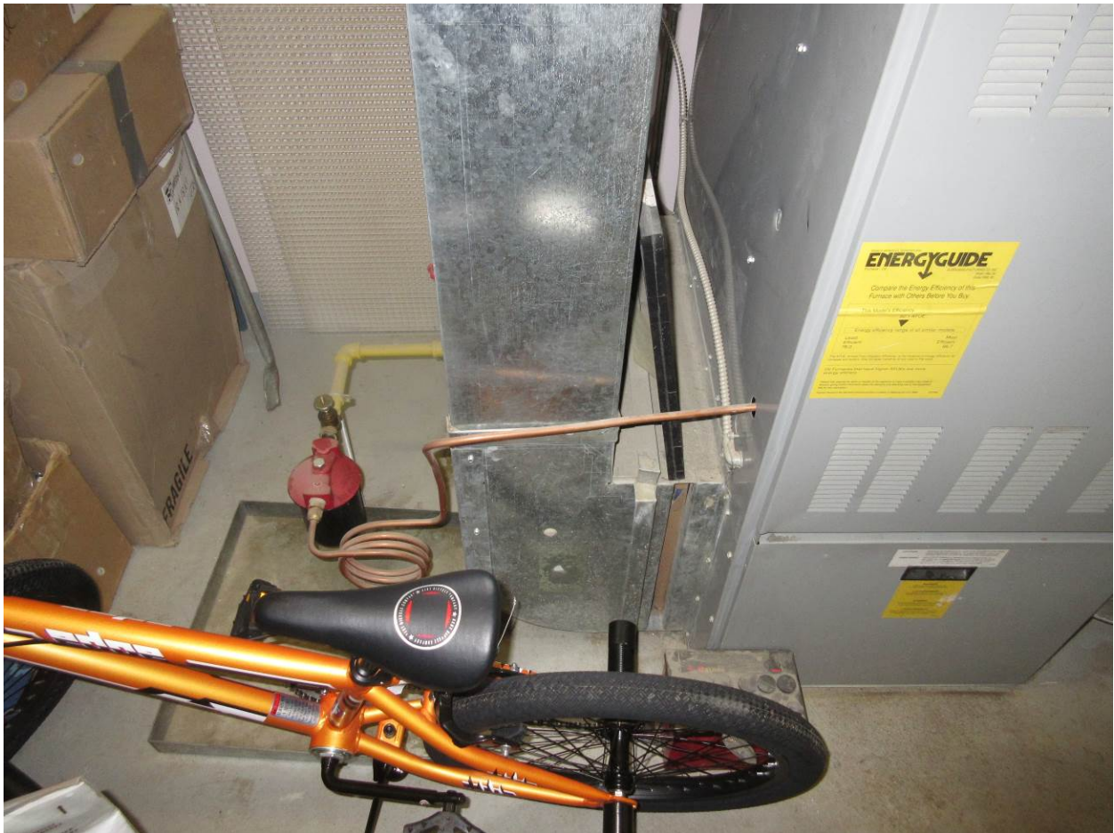
Photo 18 Furnace No.3 Fuel Piping
