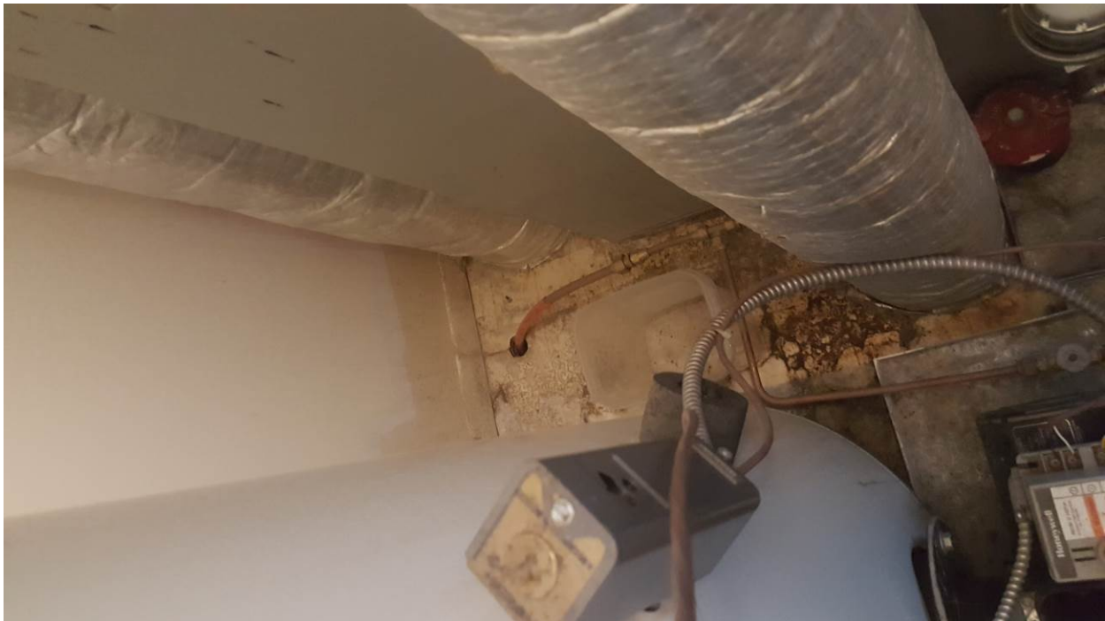
Photo 14 Piping from Crawl Space
