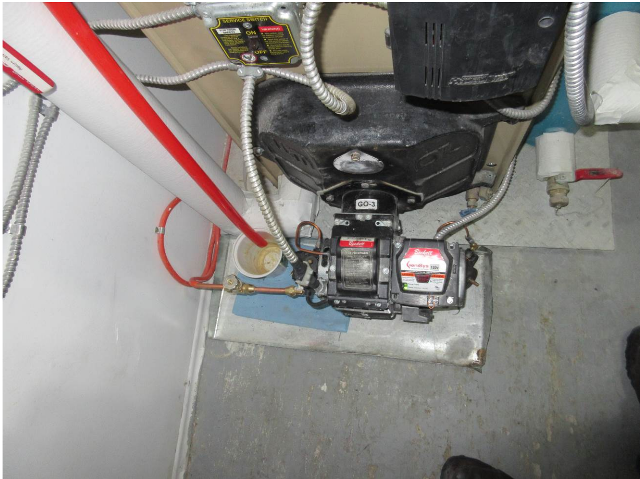
Photo 13 Fuel Line at Boiler
