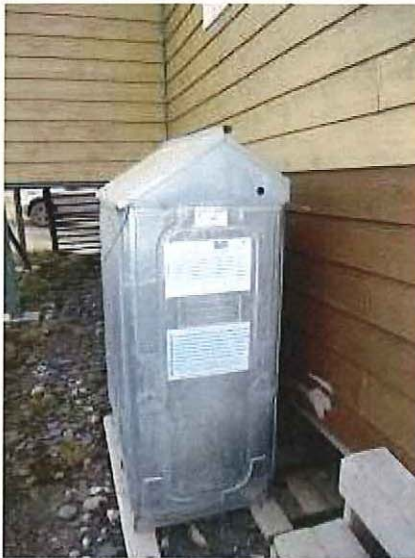
Photo 1: Outdoor above ground fuel tank
