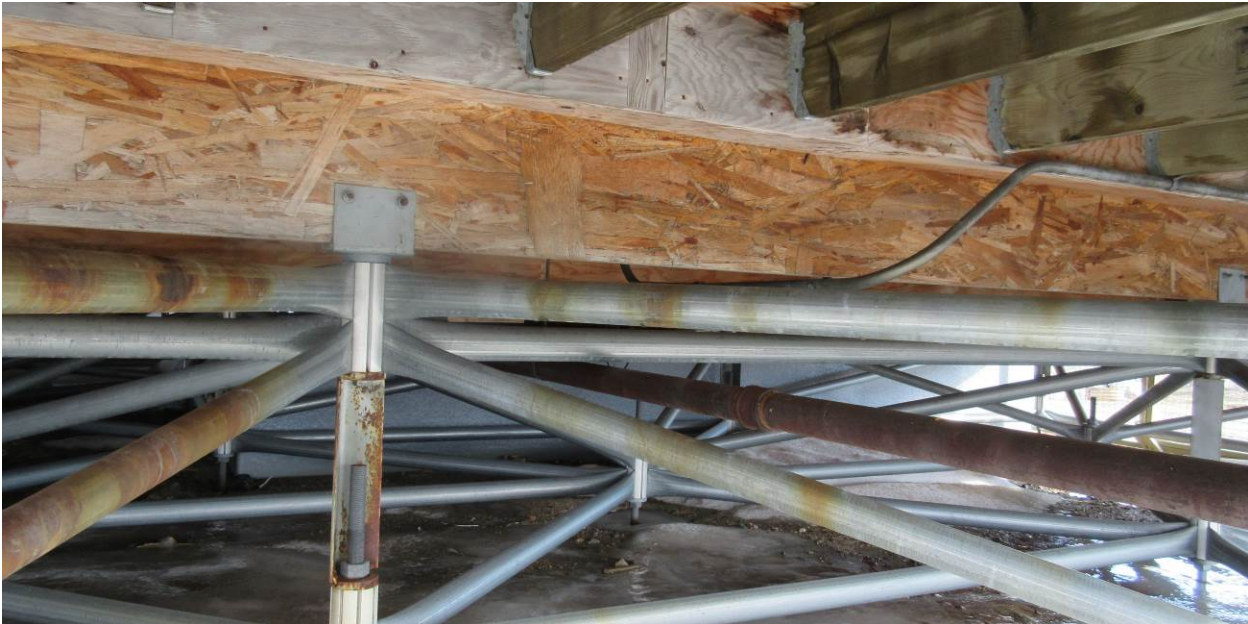
Photo 2 Exterior Piping Under Duplex
