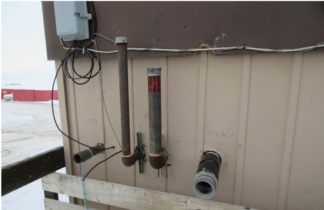
Photo 14 Exterior Fill Lines
