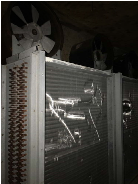
Fans associated with cold storage room
