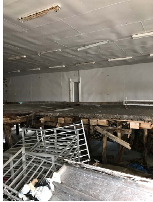
General view – interior of fish plant
