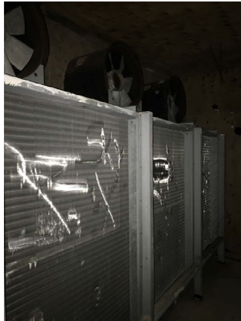
Fans associated with cold storage room
