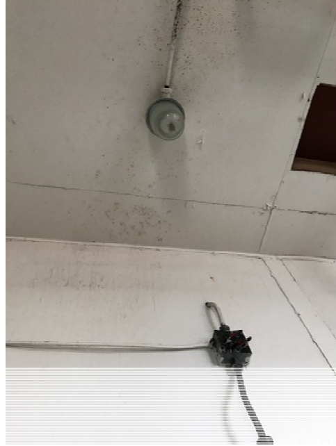
Mould on walls/ceiling - storage building
