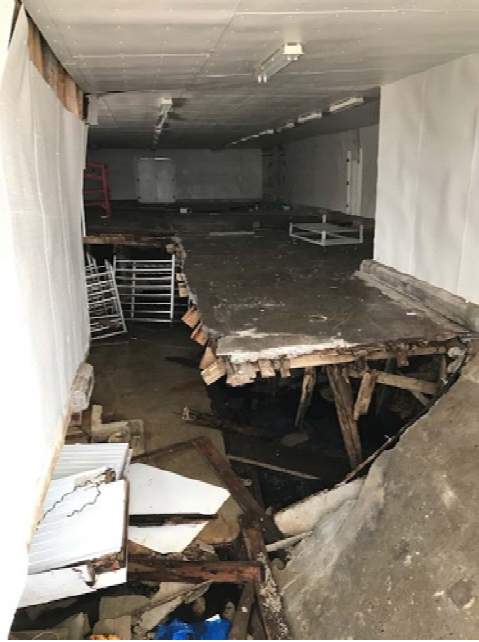
Collapsed floors (fish plant)
