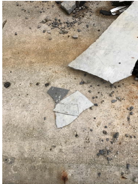
Transite (asbestos) – west side of fish plant
