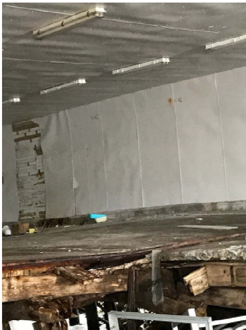
General view – interior of fish plant
