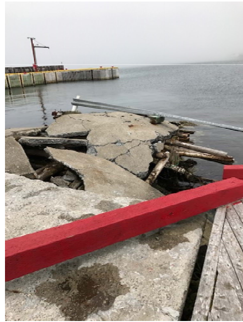
Collapsed wharf (east side of fish plant)
