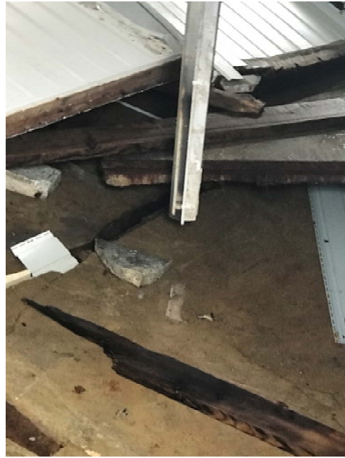
Dilapidated foundation (fish plant)
