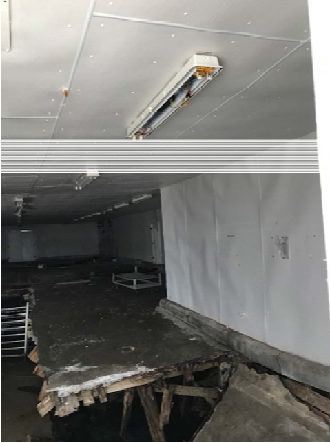
Collapsed floors (fish plant)
