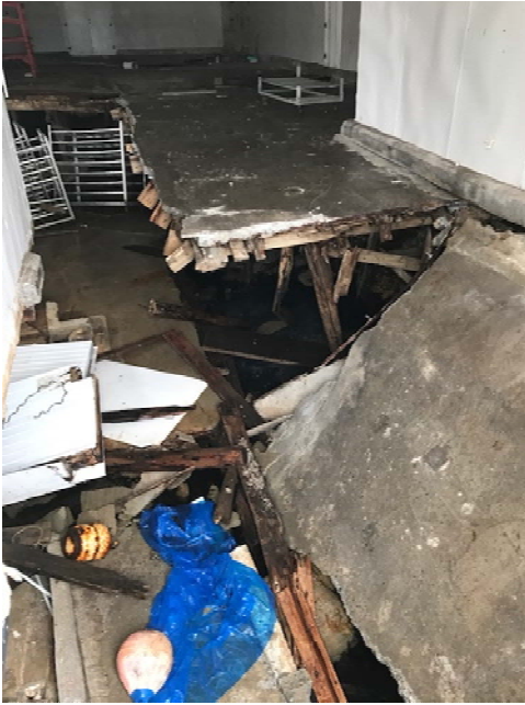
Collapsed floors (fish plant)
