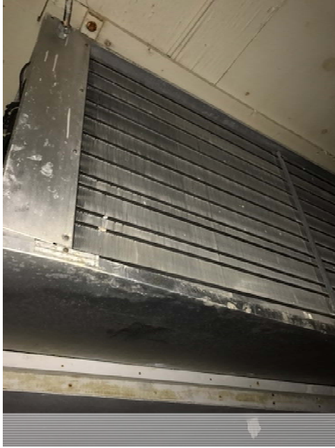
Fans associated with cold storage room
