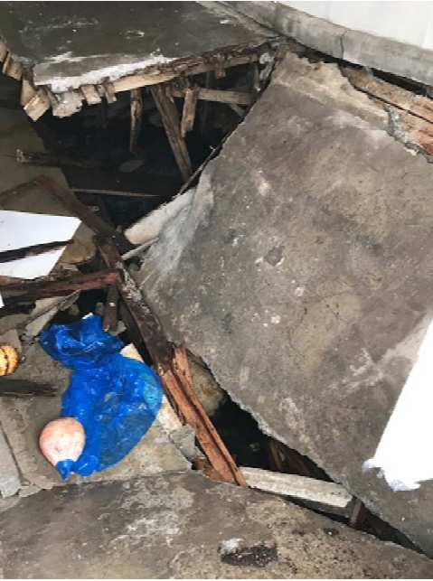
Collapsed floors (fish plant)
