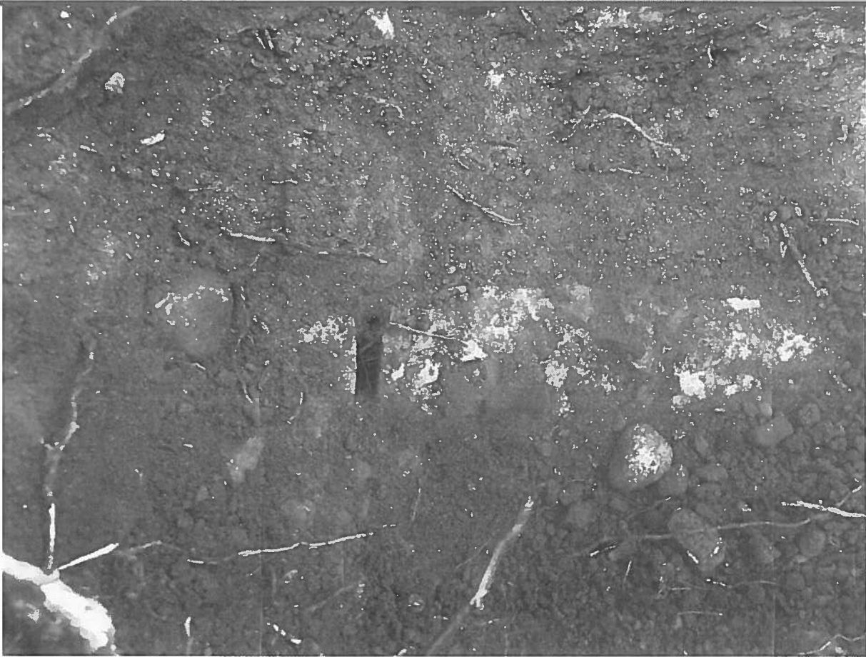
Photo 9: Clay tile pipe with root infiltration.
