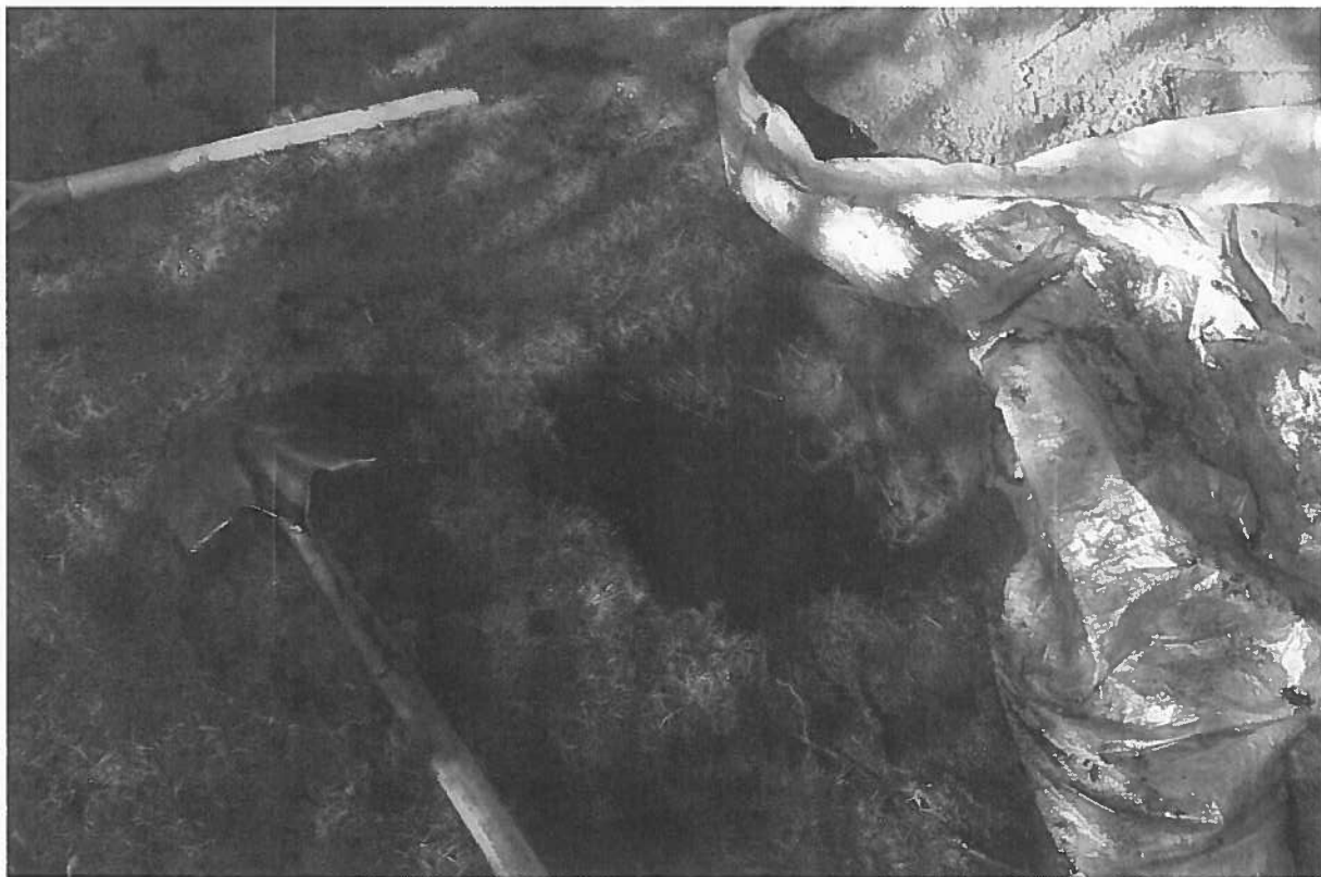
Photo 8: Roots at pipe blockage.
