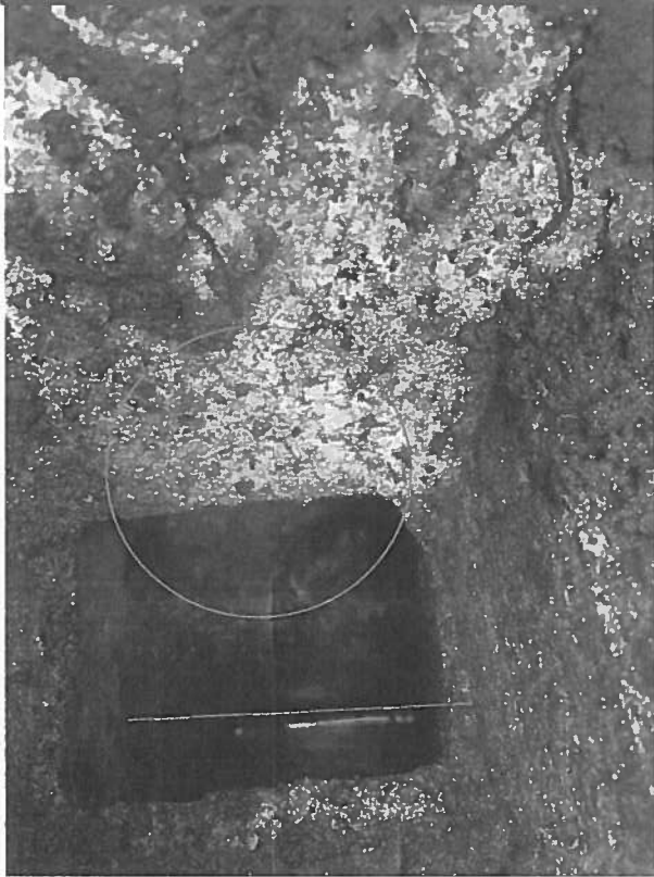
Photo 7: Liquid level approx. 4" below outlet pipe invert.
