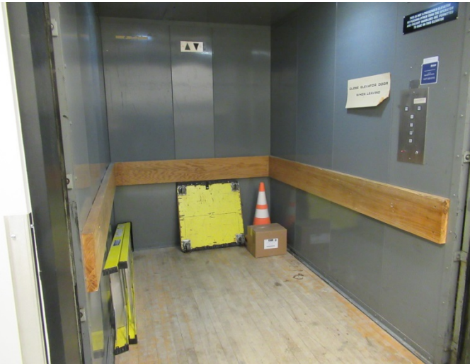
Elevator at 5201 Heather St
