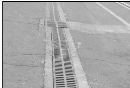
UNAUTHORIZED Sanitary Sewer Discharge point (i.e. trench drains).
