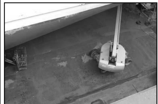
Antifoulant contaminated washwater entering the collection system (trench drains and sump wells) on the drydock floor.
