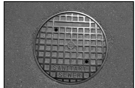
UNAUTHORIZED Sanitary Sewer Discharge point (i.e. sewer manhole).
