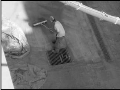
Clean up waste grit to prevent it from being washed into the drainage system by clean water (e.g. cooling water discharge, stormwater, dust suppression unit spray).
