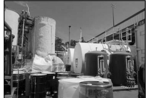
ADEQUATE containment of odorous waste.
