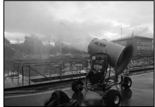
Dust suppression unit in operation.
