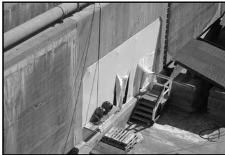
ADEQUATE containment on stabilizer pocket doors.
