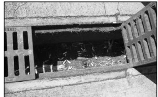
INADEQUATE: Keep trench and storm drains free of debris.
