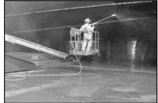
Collect and properly dispose of all contaminated water.
