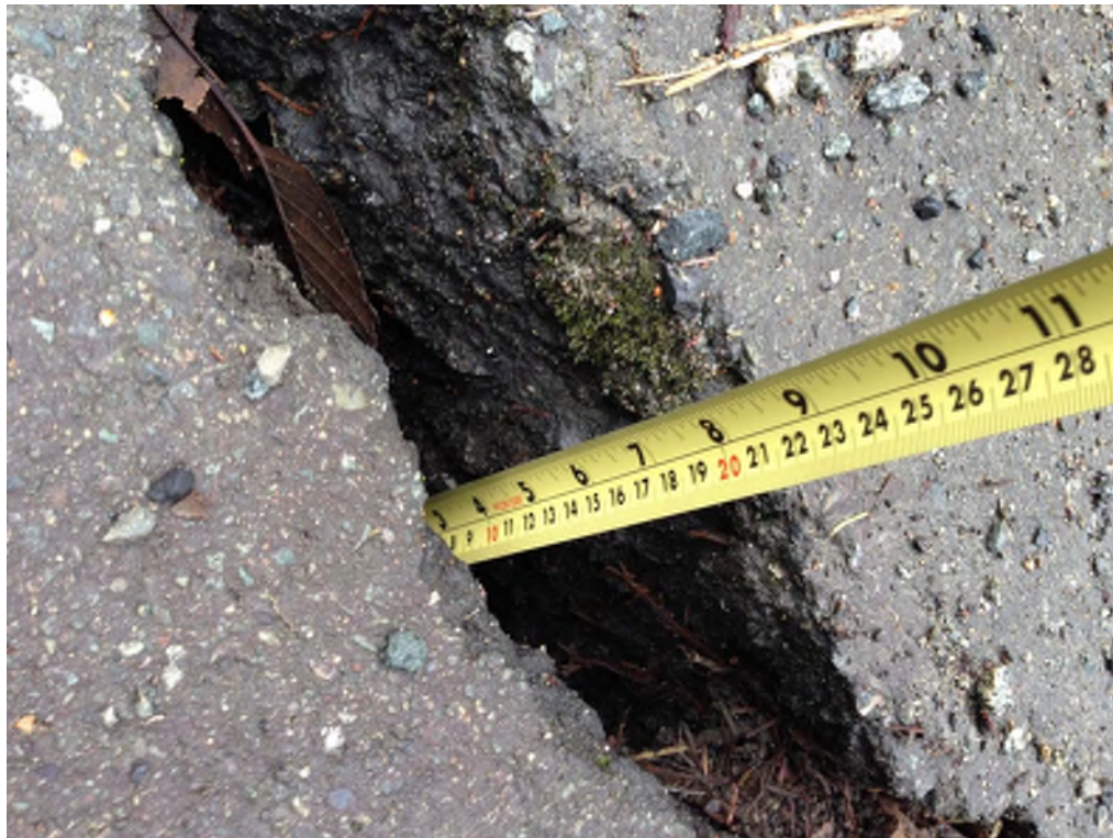
Photo 2: Open crack in south shoulder of road near BH14-01 (11 February 2014)
