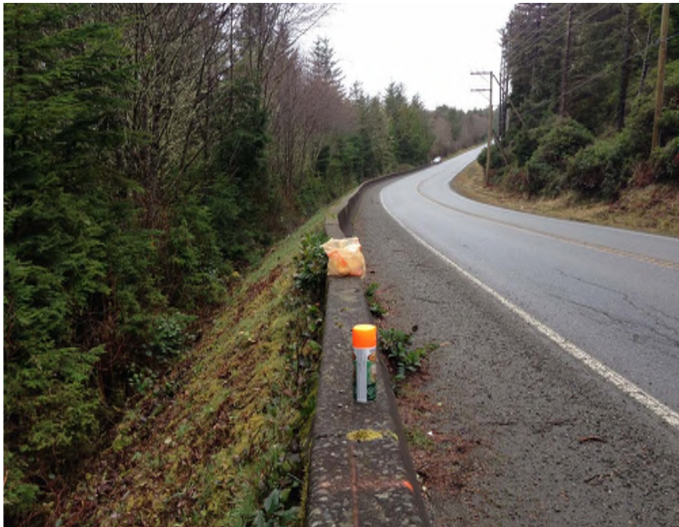
Photo 6: View looking east of open crack in road near BH14-02 and BH14-03 (11 February 2014)
