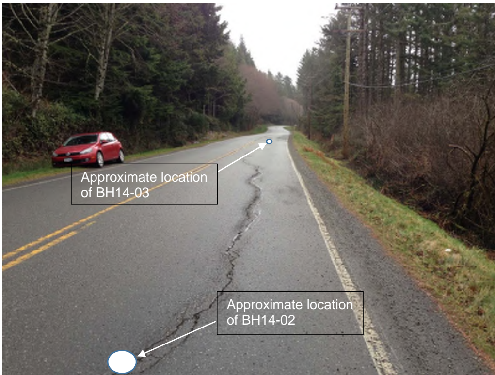
Photo 4: View looking east of open crack in road near BH14-02 and BH14-03 (11 February 2014)
