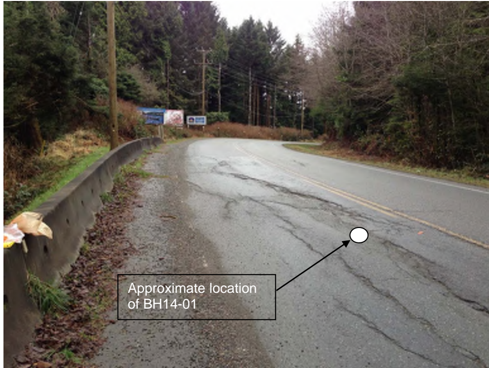
Photo 1: Condition of road on eastbound lane near Esowista IR #3 (11 February 2014)
