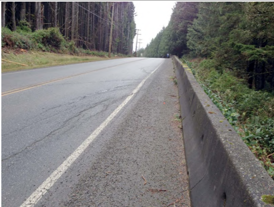
Photo 8: View looking east at road condition near BH14-04 (11 February 2014)
