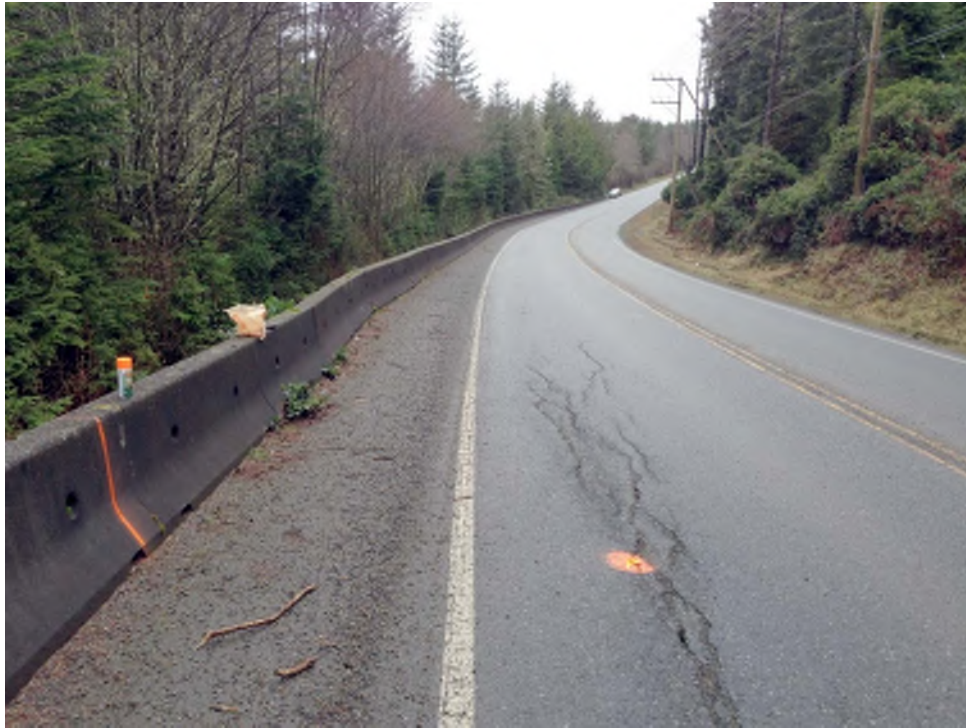
Photo 7: View looking west at road condition near BH14-04 (11 February 2014)
