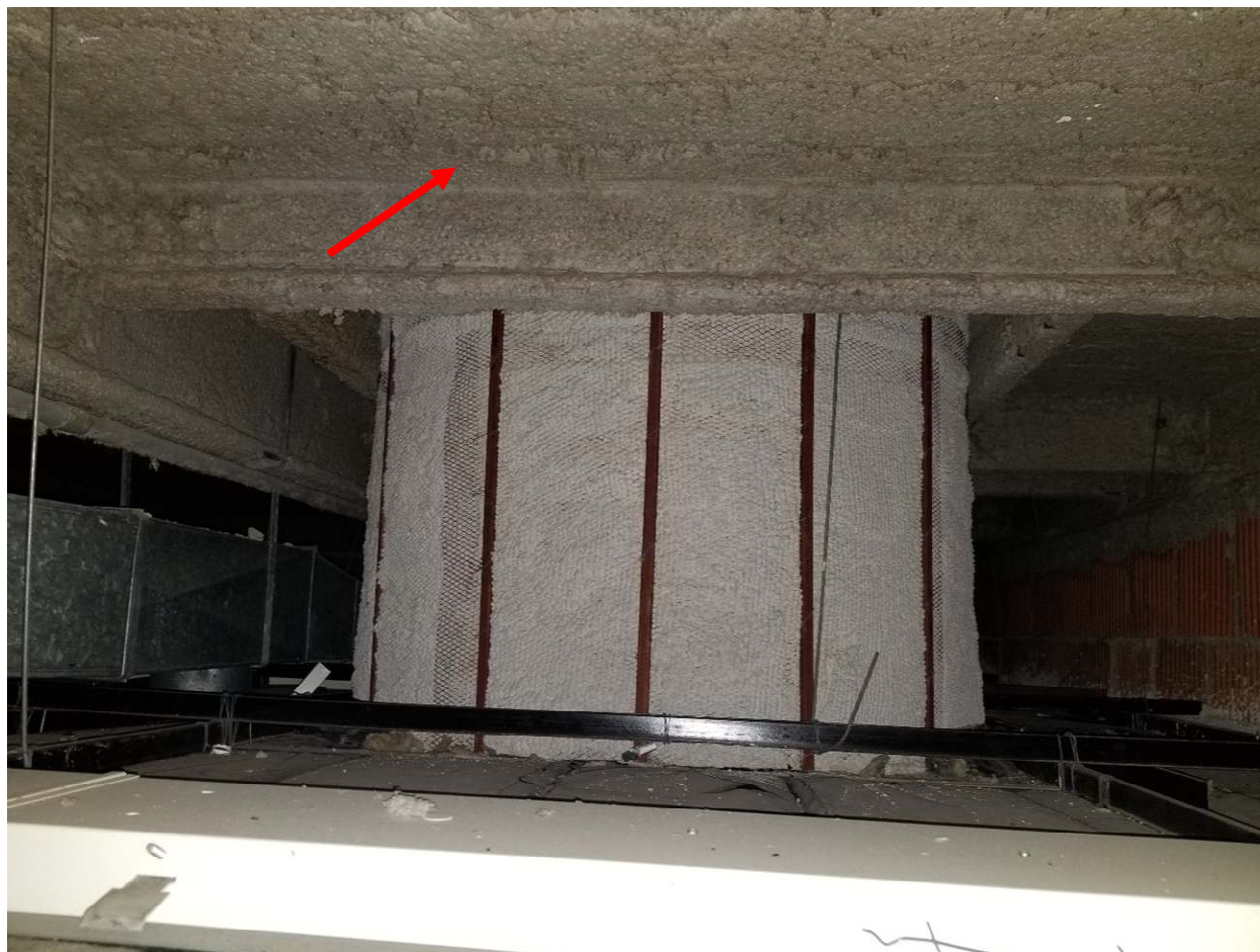
Photo 3: Friable spray on fireproofing, located on the deck above the suspended ceiling of Room E123 was confirmed to contain 65% Amosite asbestos (DST Sample 31268-13A).
