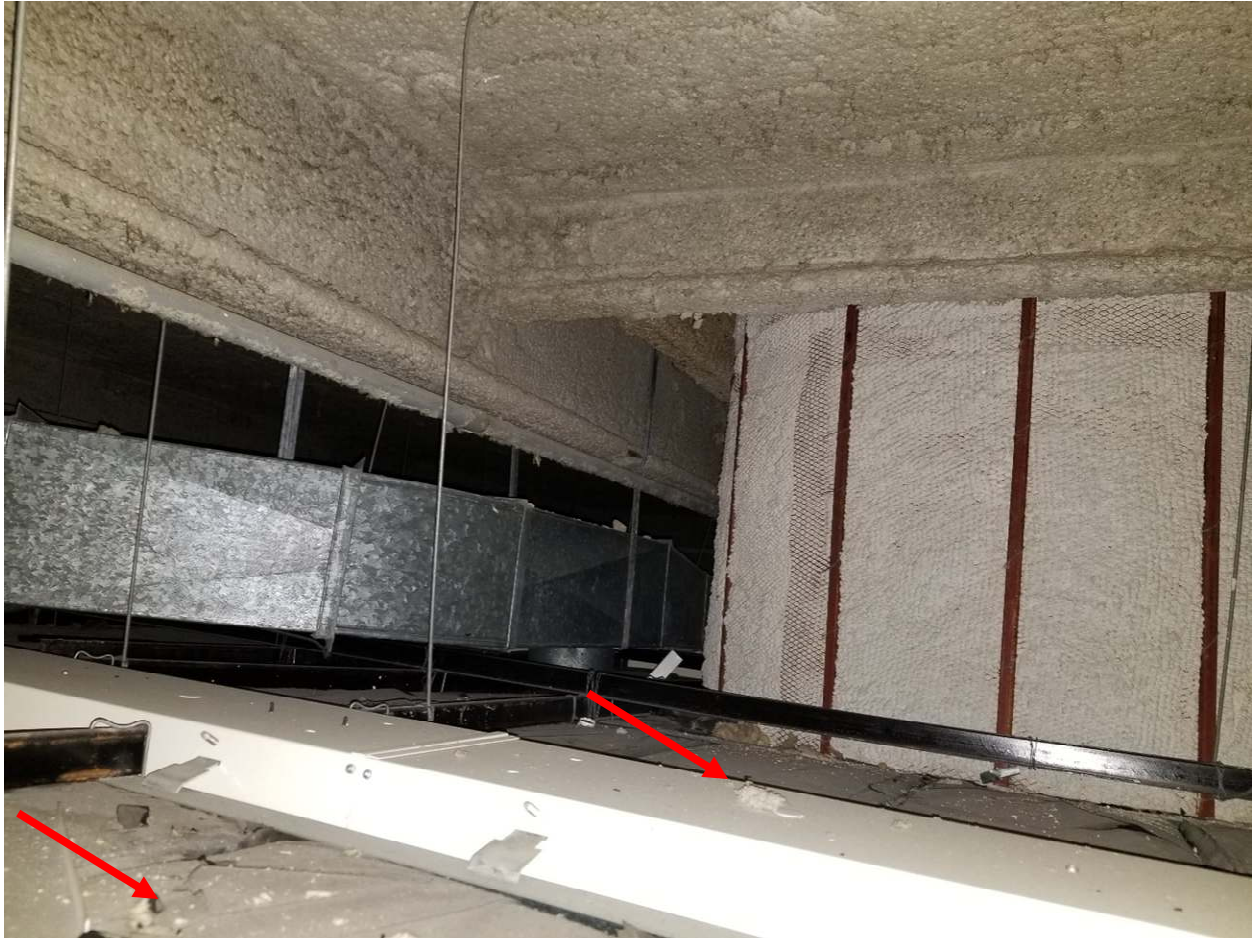
Photo 4: Asbestos-containing fireproof debris was observed on the suspended ceiling throughout Room E123.
