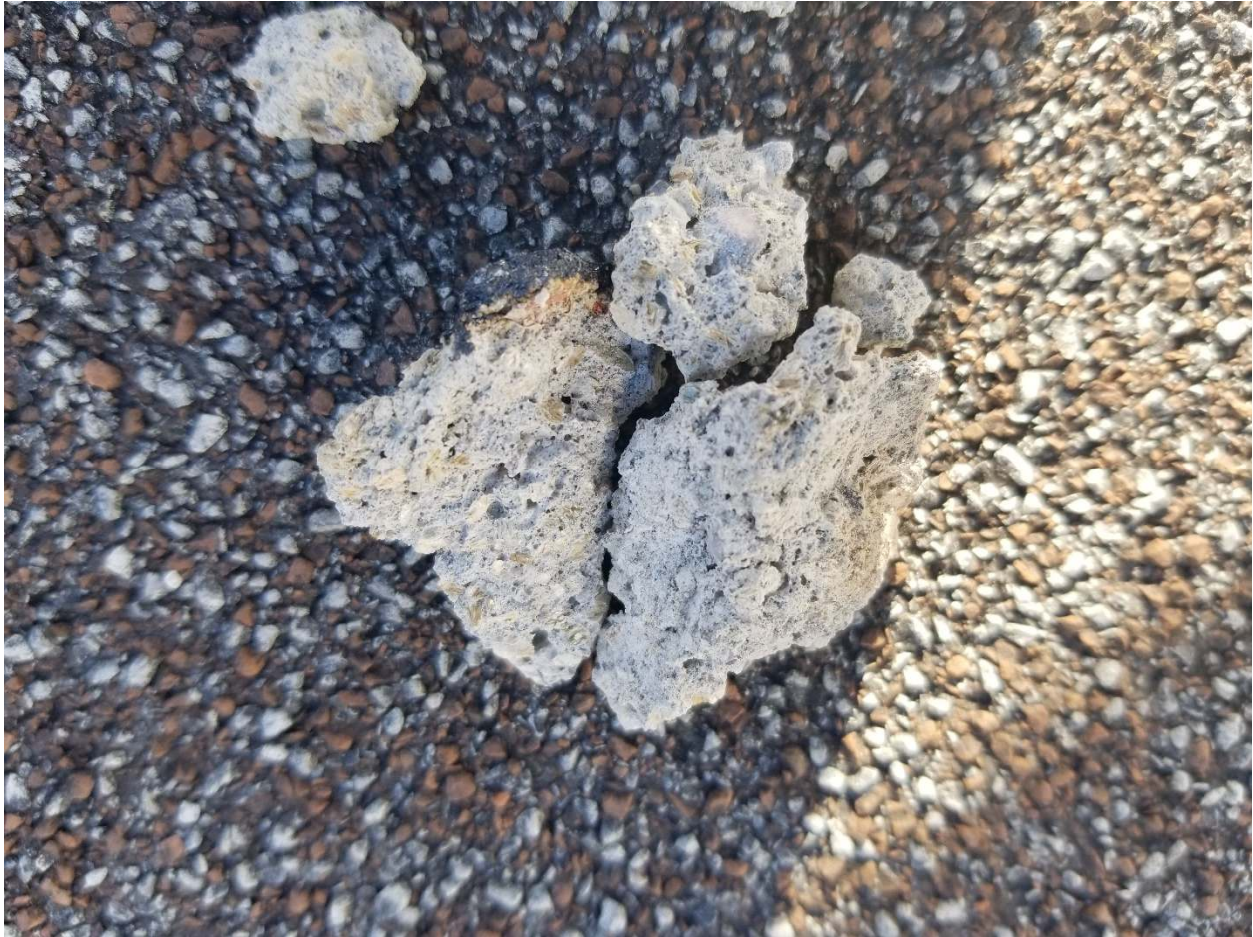
Photo 5: Non-friable cementitious roof leveling compound, located under existing roofing materials from Block 1 was confirmed to contain 1% Tremolite asbestos (DST Sample 31268-15A).
