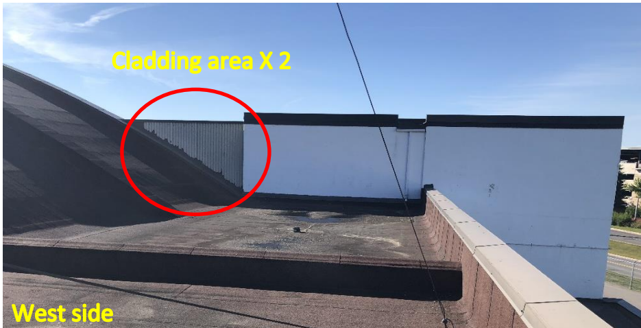
Transit board cladding identified in red and located on each side of the barrel roof.
