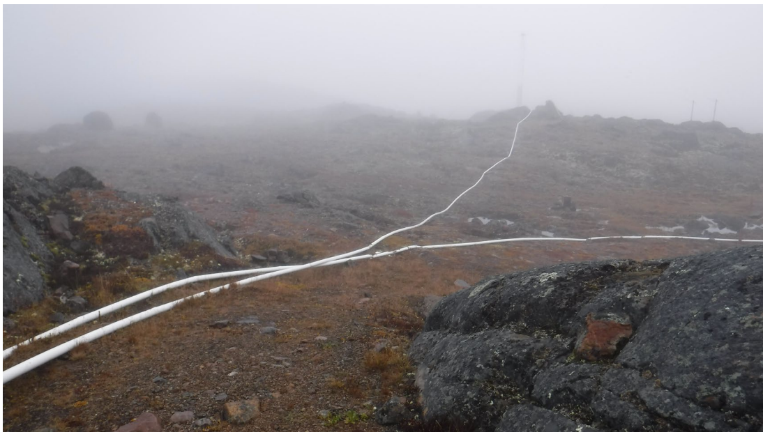
Figure 4: Existing conduit installed on site
