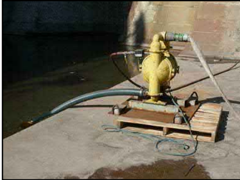
The sill diversion pump removes clean seawater from the pool at the front of Section 1 (moon pool) and discharges into the tunnel drains through a hard pipe on the graving dock wall.
