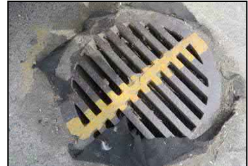
Uplands storm drain with filter cloth. Avoid storing hazardous materials near storm drains, which are directly linked to the marine environment.
