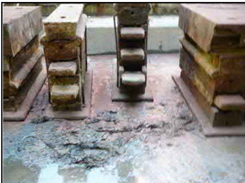
Sediment from the harbour often settles on dock bottom after dewatering. If this becomes contaminated with paint, etc., it must be disposed of.
