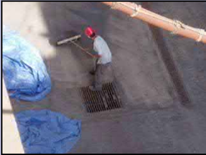
Clean up waste grit to prevent it from being washed into the drainage system by clean water (e.g. cooling water discharge, stormwater, dust suppression unit spray).
