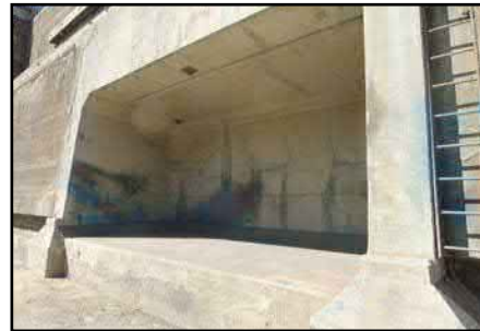
Paint overspray due to INADEQUATE containment stabilizer pocket doors.
