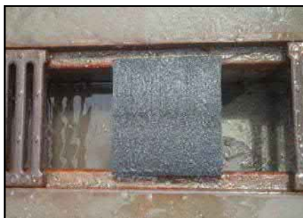
Example of high density styrofoam blocks used as a drain blocker on the NLW.
