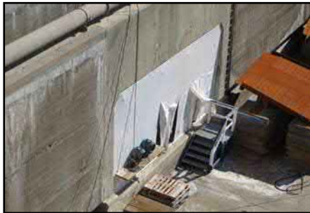
ADEQUATE containment on stabilizer pocket doors.
