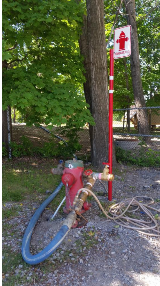
Photo 4: Fire hydrant located nearby
