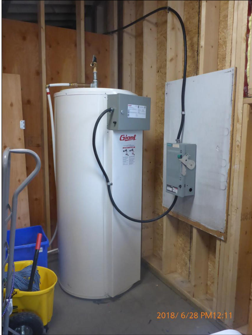
Photo 3: Water heater supplied
