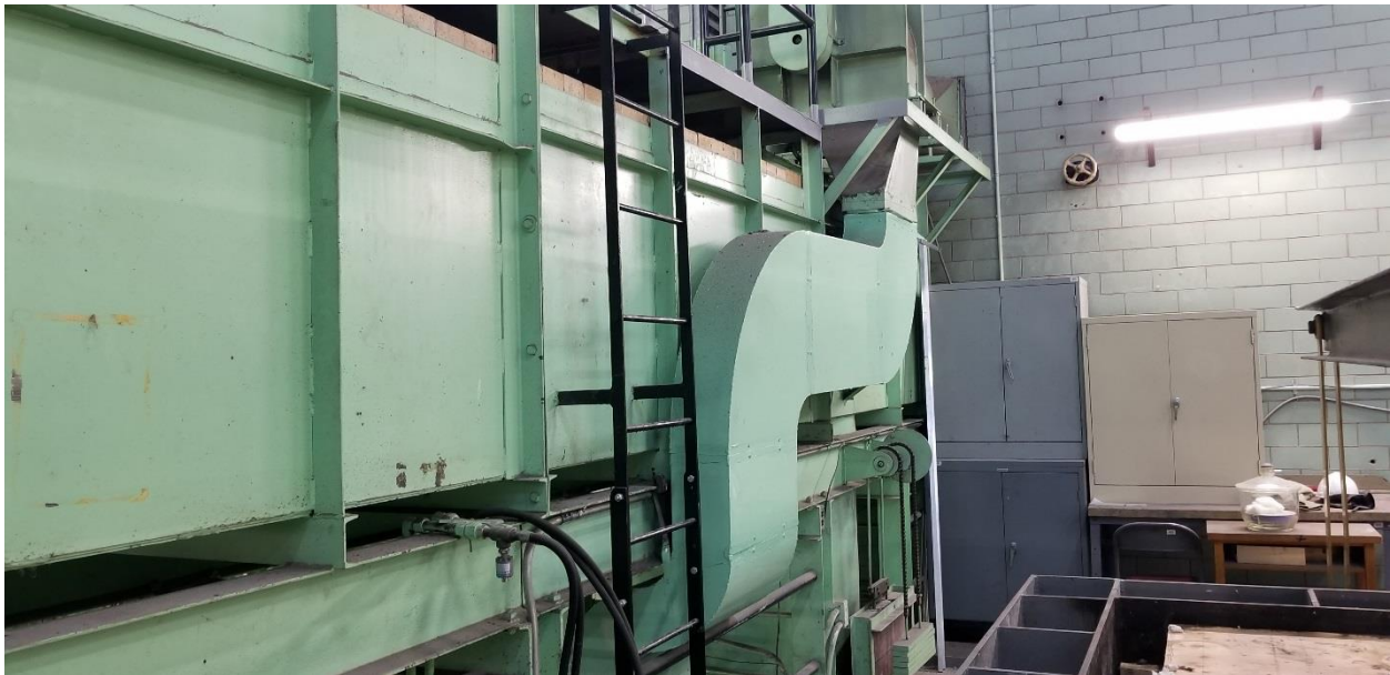
Image 1. Partial details of the air vent duct work
