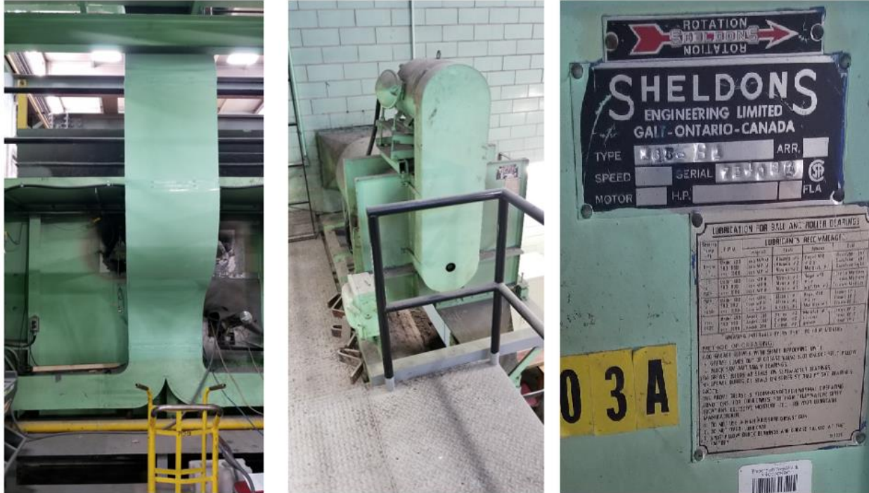
Image 2. Partial details of the air vent duct work (left image). Existing air circulating fan (middle image). Existing air circulating fan nameplate (right image).
