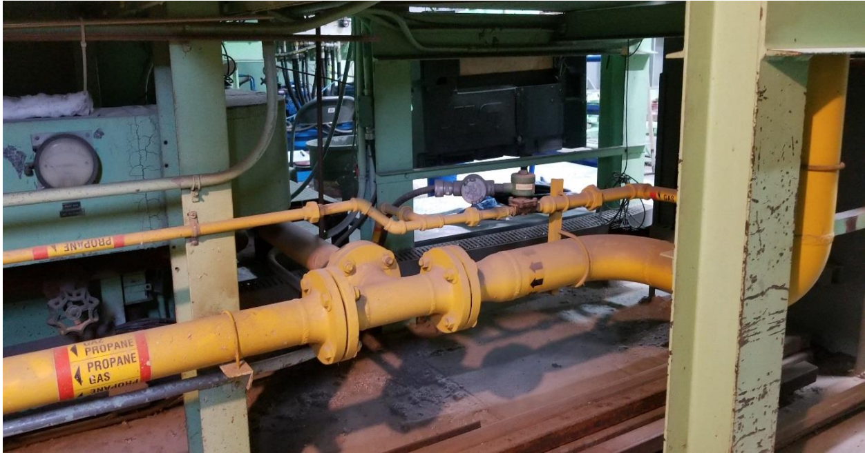
Image 1. Main gas supply to Flooring combustion Testing Furnace.
