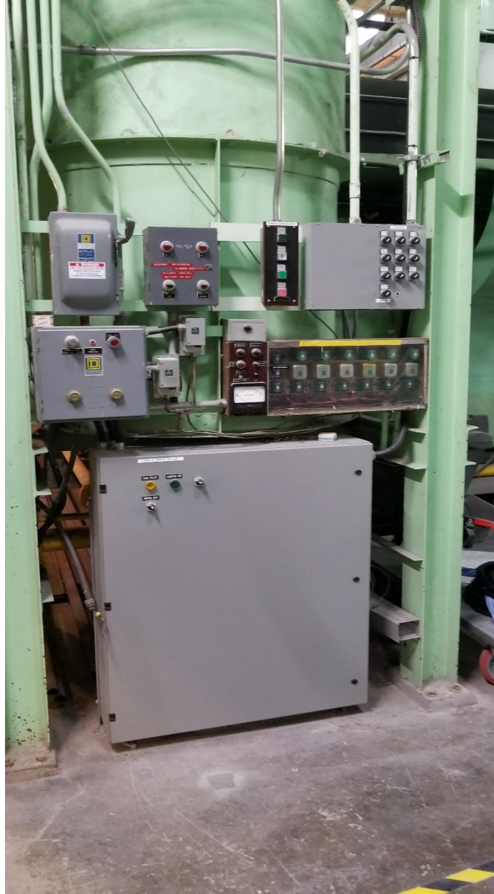
Image 4: All panels to be removed. New panel supplied to substitute the panels above.
