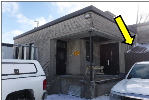
Asbestos-containing tar on flashing above Ramp Shed
