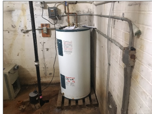
Externally un-insulated hot water tank within the Sump Pump Room (Location 10)
