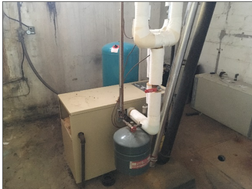
Externally un-insulated furnace within the Sump Pump Room (Location 10)
