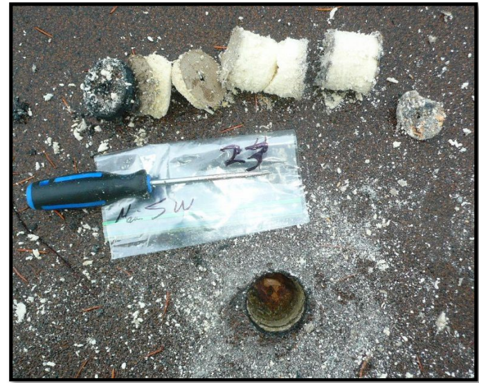
Roofing materials core layer Sample 17A-TSB-23 collected from the southwest portion of the Technical Services Building.
