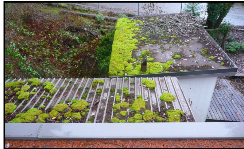
Looking eastward from the roof of the Technical Services Building onto the east attached open ended canopy (foreground) and detached storage shed (upper right).
