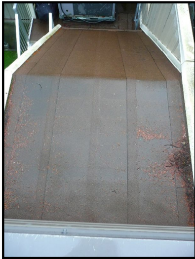
Looking southward from the roof of the Technical Services Building down onto the top of the south staircase canopy.
