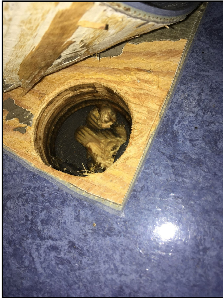
Close-up of exploratory review of modern vinyl sheet flooring and underlying plywood and wood blocking within southwest corner of office area.
