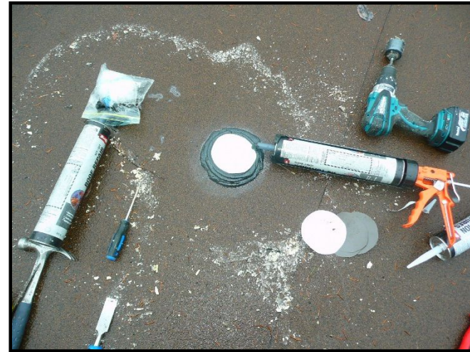
Post-core-sampling temporary fill and patch with flashing cap on the southwest portion of the Technical Services Building ( not warranted ).
