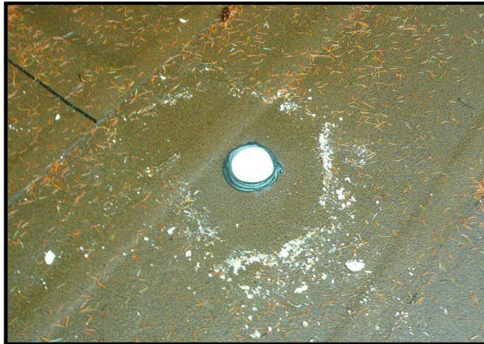
Post-core-sampling temporary fill and patch with flashing cap on the northeast portion of the Technical Services Building ( not warranted ).
