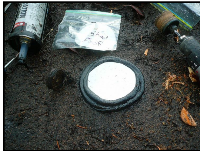
Post-core Sample 17A-TSB-25 temporary fill and patch with flashing cap on the detached storage shed ( not warranted ).
