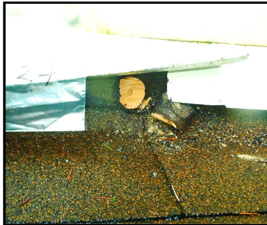
Roofing materials core layer Sample 17A-TSB-24 collected from the east cant strip under the flashing of the south staircase canopy. Subsequently filled and patched with flashing cap ( not warranted ).
