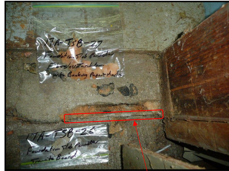
Sample 17A-TSB-26 of sub-grade hard fireproof composite fibre cement board panelling (Transite Panel) (10 % Chrysotile) and Sample 17A-TSB-27 of fibreglass insulation with backing paper and black mastic large (None Detected) as collected from the east elevation at the entrance to the Carpenter Shop Room #7.
