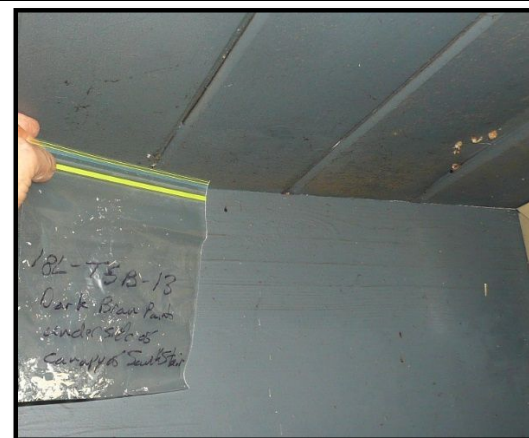
Dark Brown Paint Sample 18L-TSB-13 representative of the underside of the canopy over south staircase as collected from the east side of the Furnace Breaker Building.
