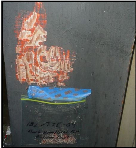
Brown-Grey Paint on Orange Paint and White Paint Sample 18L-TSB-04 and Painted Base Substrate TCLP Sample 18TCLP-TSB-04 from the exterior door of the Paint Shop # 6.
