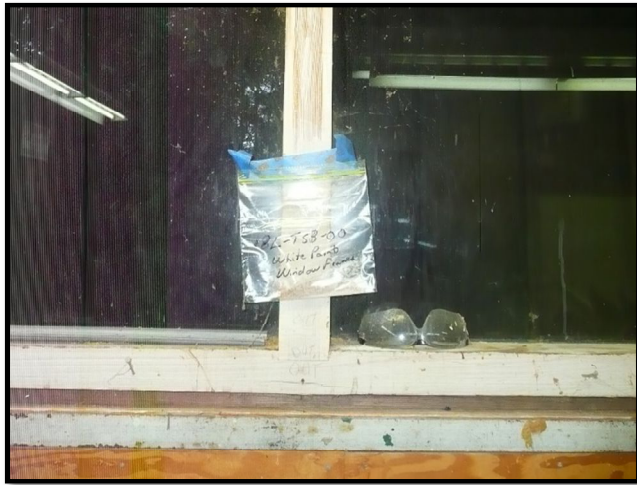
White Paint Sample 18L-TSB-00 from the interior side of wooden window frame in the Carpenters Shop Room # 7.
