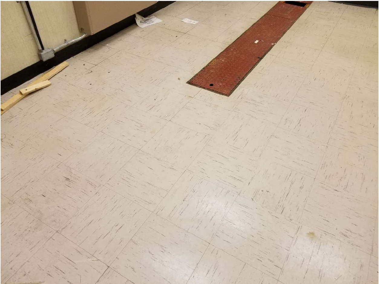
Photograph 3: 12"X12" vinyl floor tiles, off white with brown streaks, pictured in Room 064, was confirmed to contain 2% Chrysotile asbestos (DST Sample ID 31268-M23A-01A-C).
