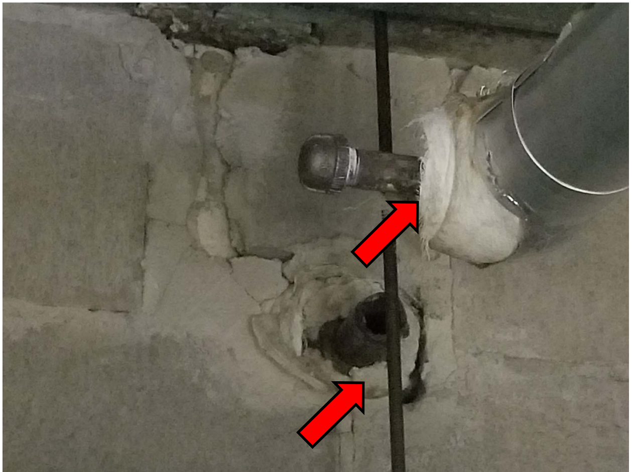
Photograph 2: Friable grey cement compound pipe fitting insulation (poor condition), pictured in Room 064. Historic laboratory analysis has confirmed this material contains 50 to >75% Chrysotile asbestos (Historic Oakhill Sample IDs M23A-02A and M23A-08A).
