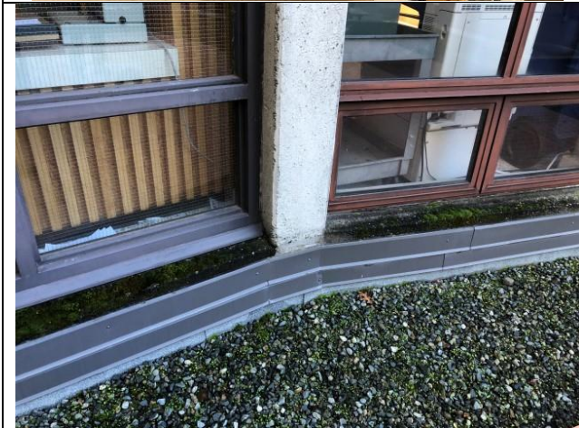
Photo 4 – Sample of Base of Wall Conditions
