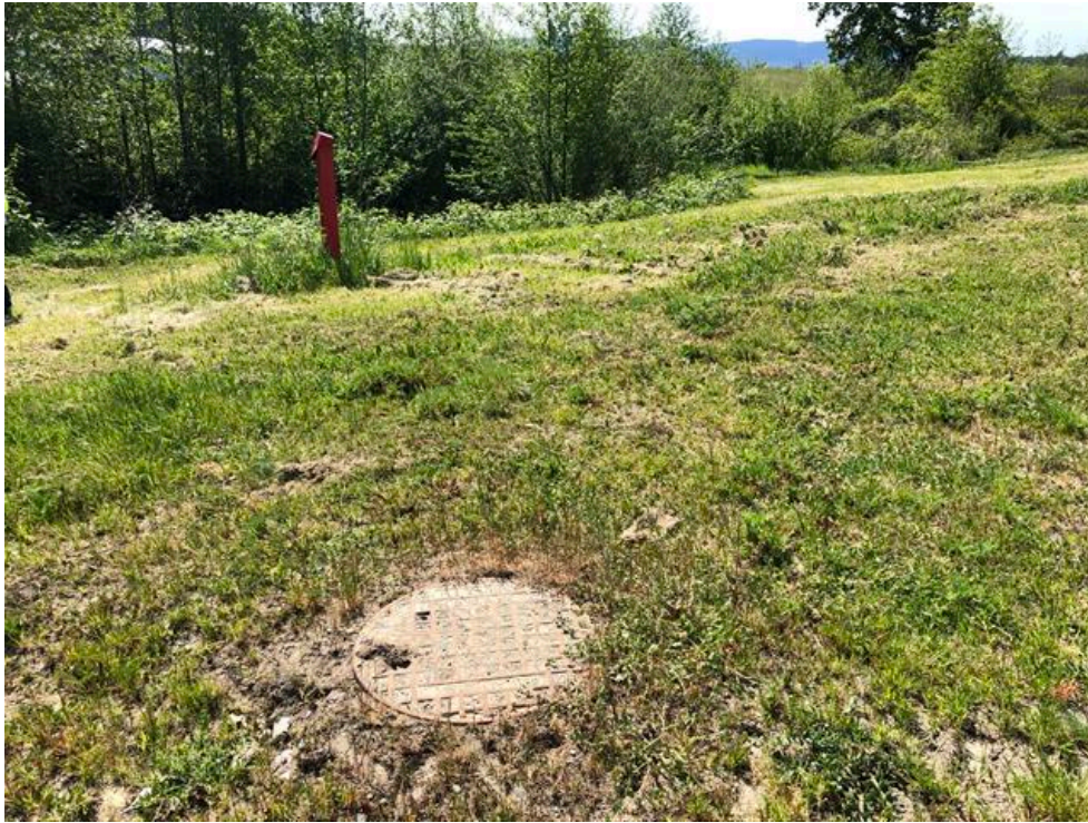
Photo 15: Storm lines adjacent to Reach 1C and Reach 1A to be protected, looking south.
