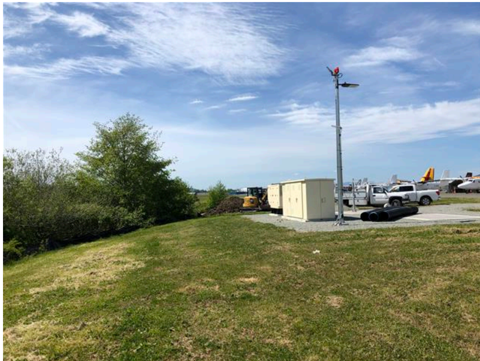
Photo 16: Utility infrastructure along north side of Reach 1A at upstream end, looking west.
