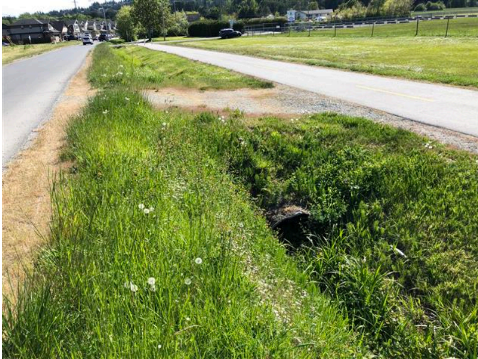
Photo 9: Alternate road-side ditch crossing to potential alternate stockpile or laydown area, looking south. Cycling / Pedestrian path visible in right of photograph. Crossing to be maintained and protected.
