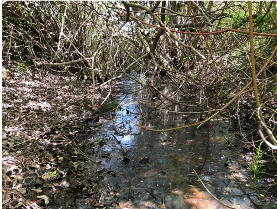
Photo 19: Newly installed storm outlet pipe from pumphouse to upstream end of Reach 1A and old abandoned PVC storm pipe to be protected, looking north.
