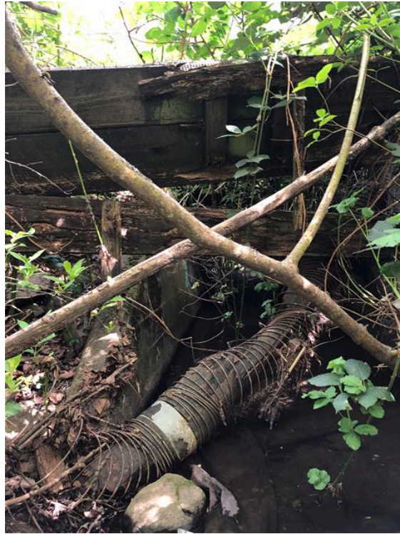
Photo 43: Old metal-coiled wood stave water pipe at downstream end of Reach 4 near Canora Road culvert, looking south. Pipe has collapsed into Reay Creek.
