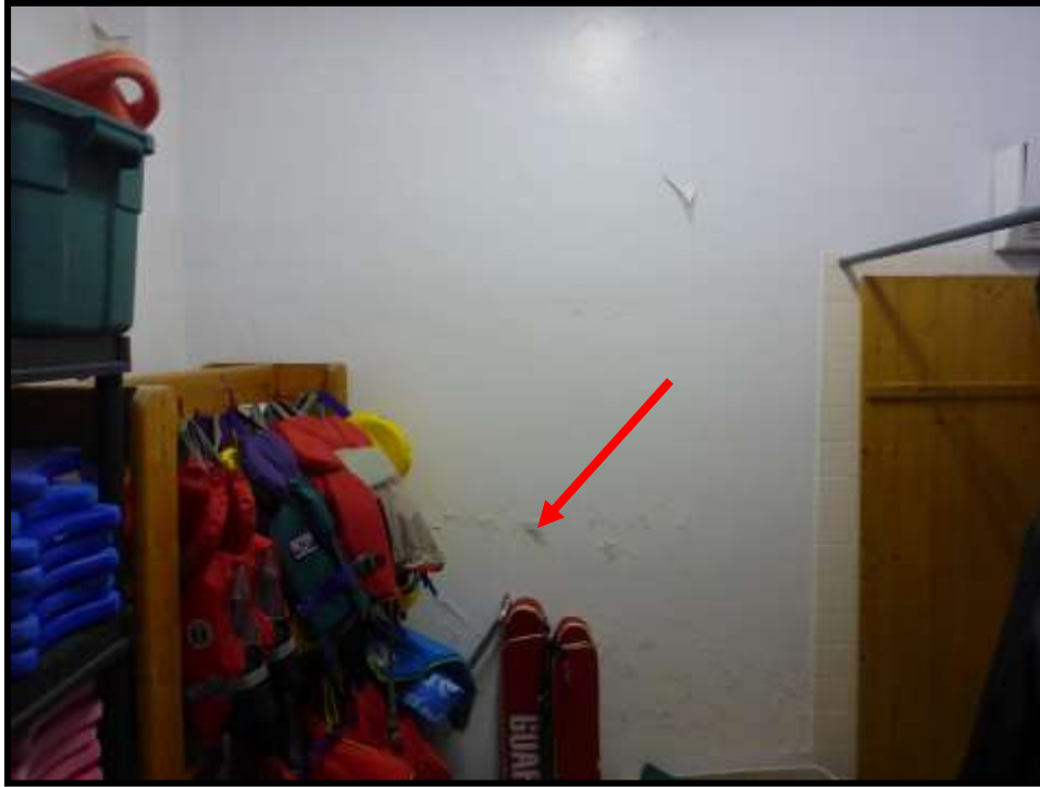
Photograph #7 – Example of Lead-Based Green Paint Under Other Layers – Room 115
