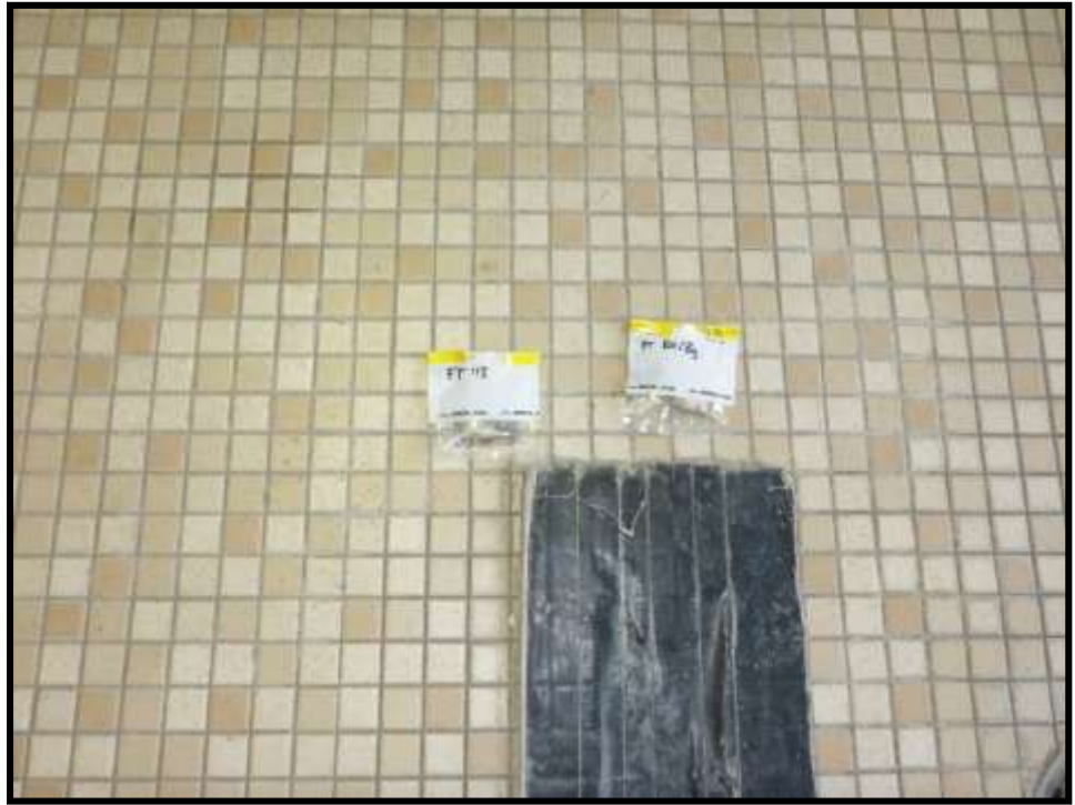
Photograph #1 – Asbestos-Containing Tile Thin Set Mortar under Brown & Beige Tiles – Room 113 (Sample A8b)
