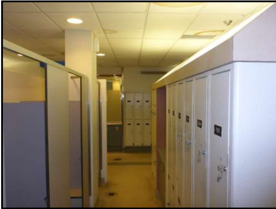
Photograph #5 – Asbestos-Containing Plaster Base Coat – Column Room 104 105 (Sample A24b).
