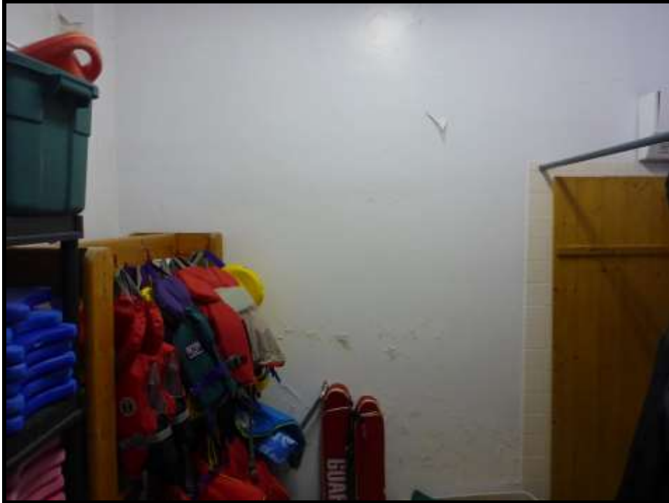
Photograph #4 – Asbestos-Containing Plaster Skim Coat – Room 115 (Sample A13a).
