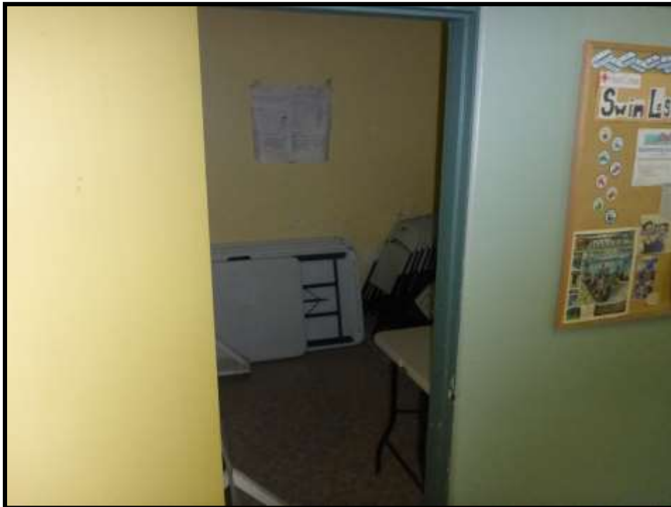
Photograph #6 – Lead-Based Green Paint on Plaster Wall (Sample Pb17).
