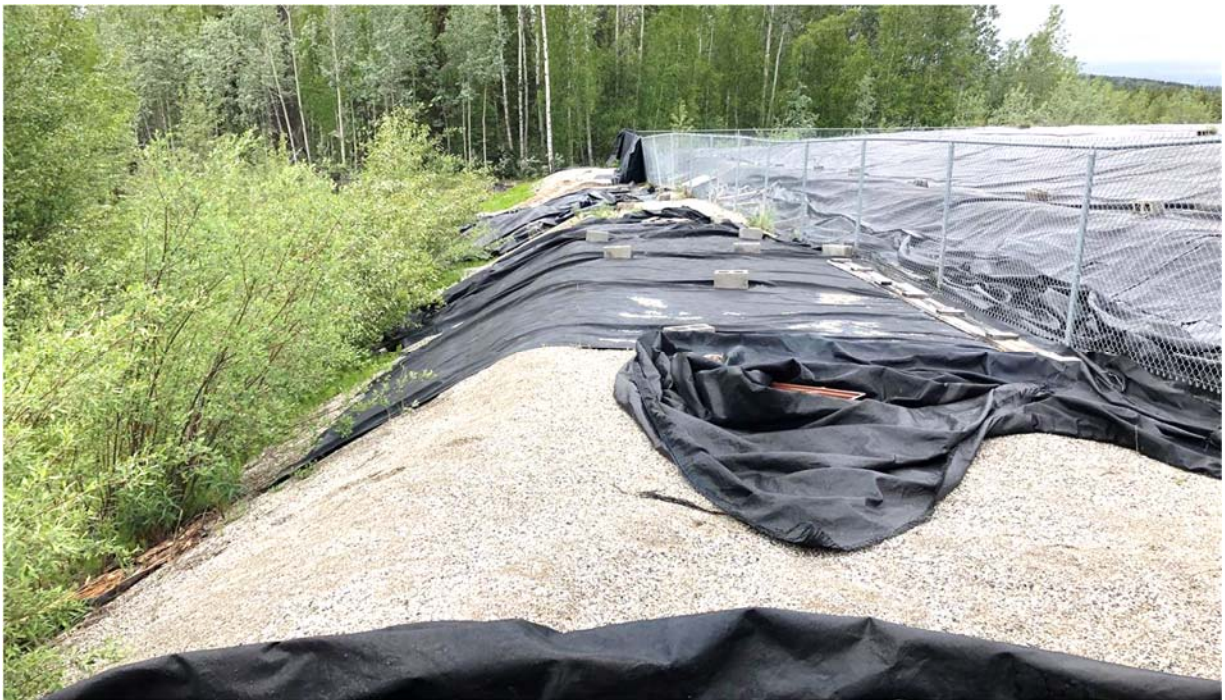
Photo 2: View of Iron Creek southern berm showing disturbed berm cover (foreground) and berm repair area (background), facing west.
