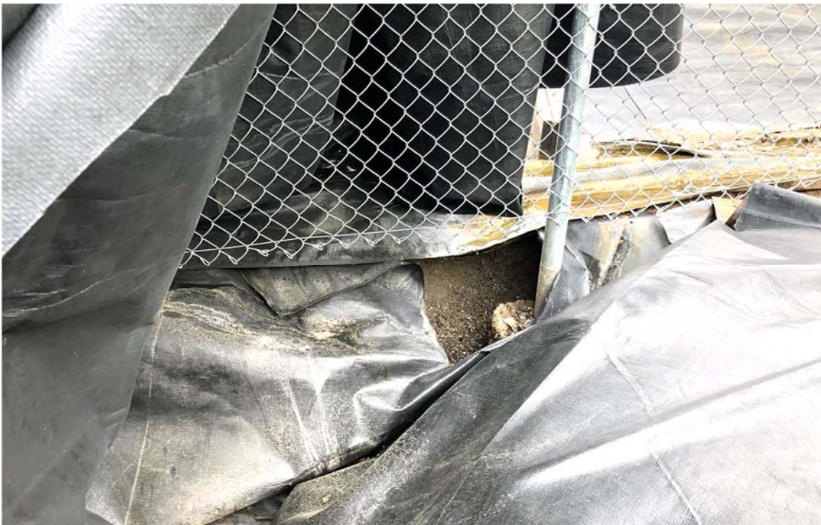
Photo 4: View of Iron Creek southern berm fence post to be secured and realigned.
