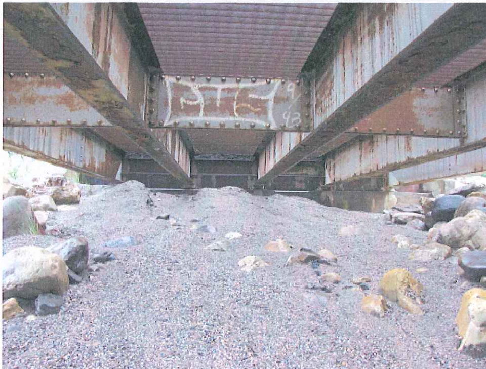
Photo 6 – Corroded Steel I Girder – Approach Span
