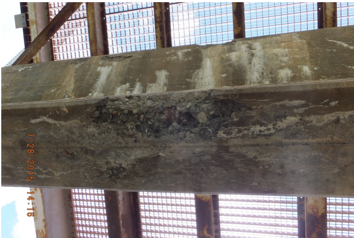
Photo 1 – MacDonald Bridge, Underside of south pier cap, spall with exposed stirrups.
