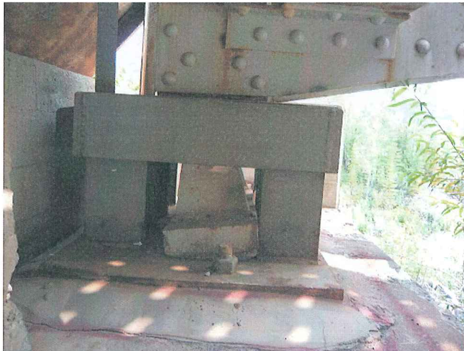
Photo 10 – Bearing Touching Limiter
