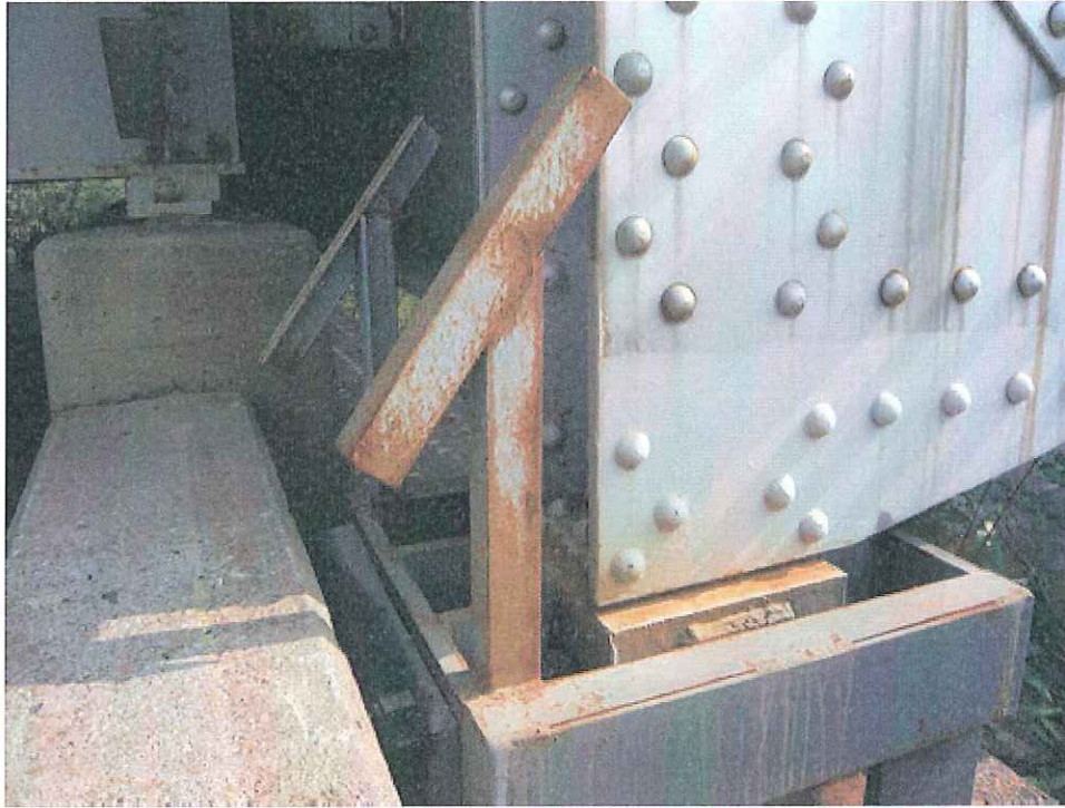
Photo 13 – Limiter and Debris Prevention Plate (missing)
