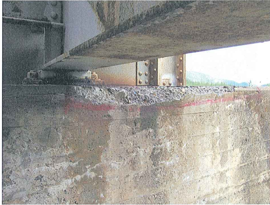
Photo 7 – Concrete Spalling at Pier
