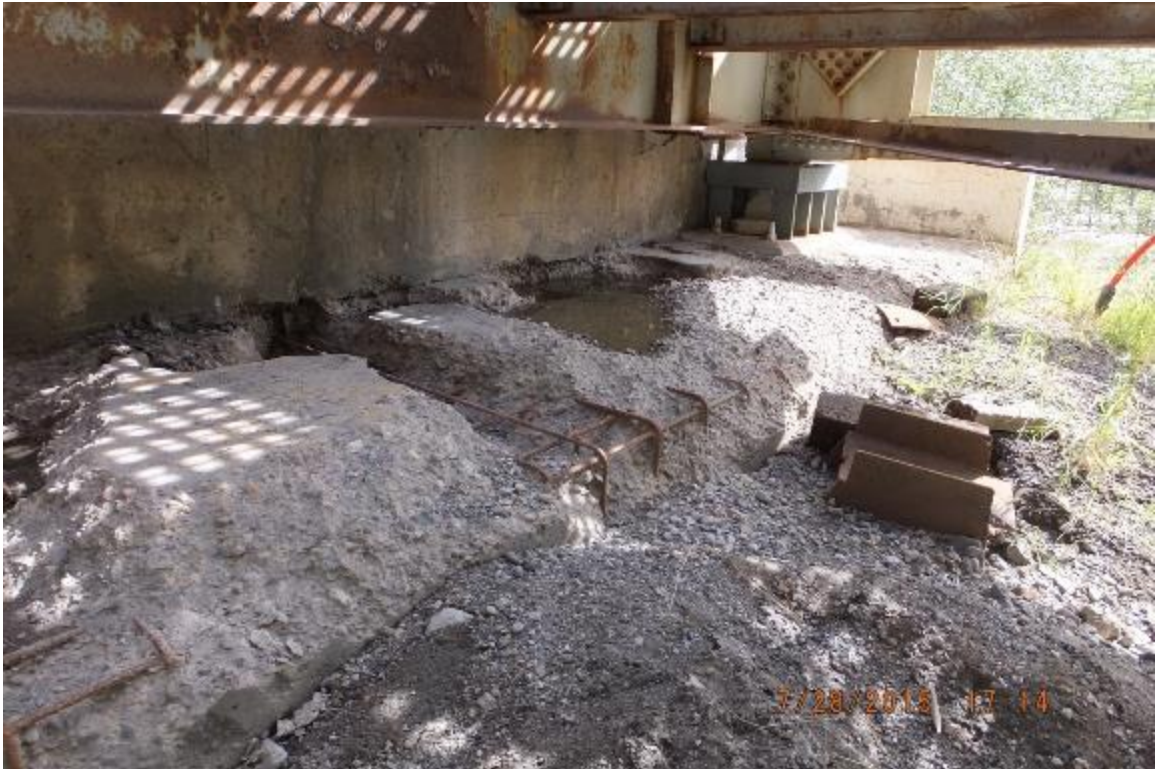
Photo 4 – South abutment bearing seat of the Racing River structure. Severe scaling with exposed rebar
