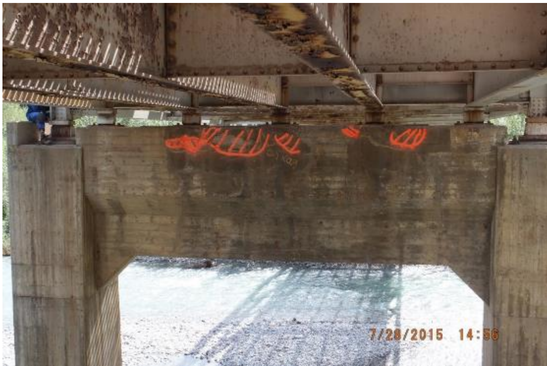
Photo 5 – Delaminated concrete patch repairs in the pier cap of the MacDonald bridge. exposed rebar.
