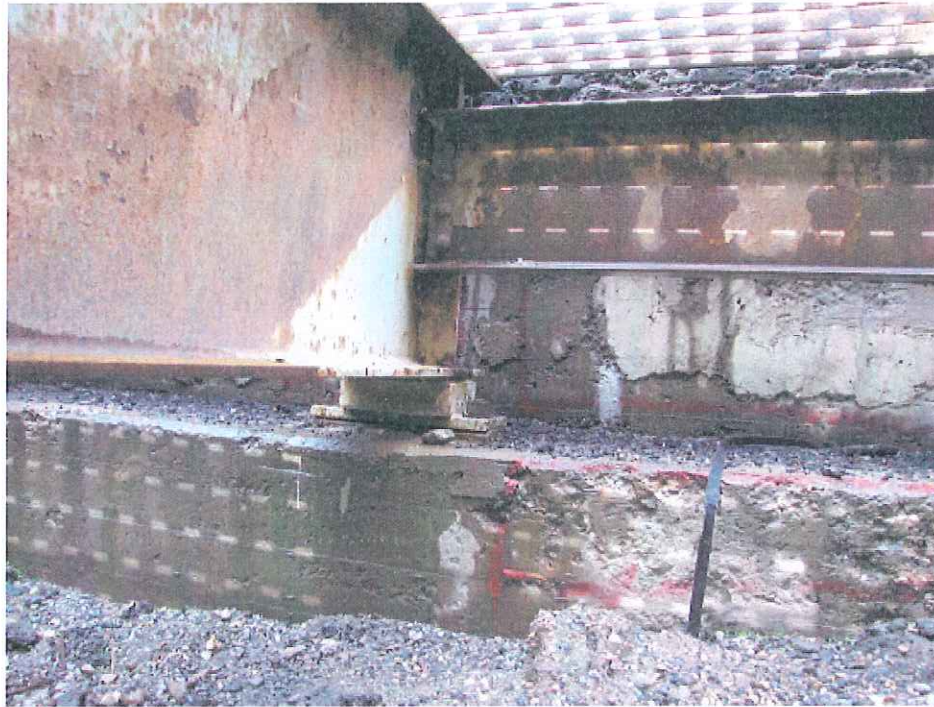
Photo 13 – Spalling at South Abutment
