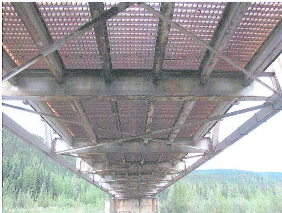
Photo 10 – Condition of Floor Beams, Stringers and Bracing
