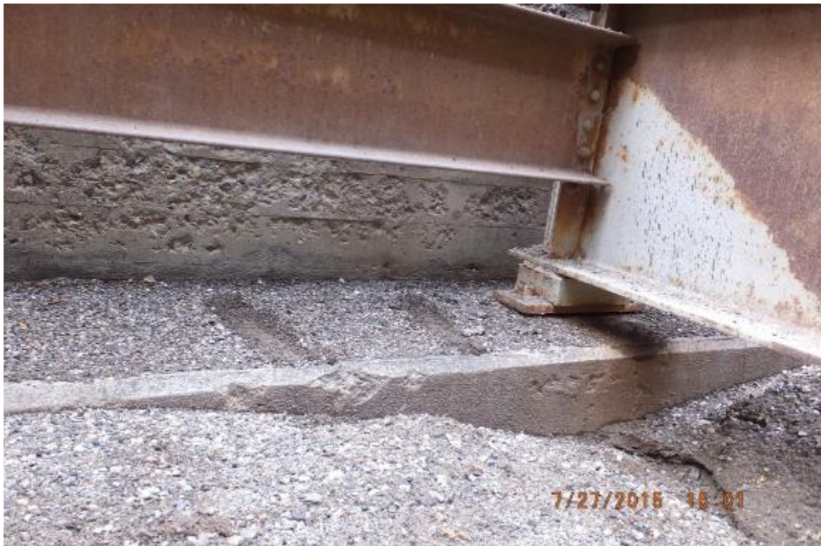
Photo 7 – North abutment of Tetsa structure with scaling in the backwall.
