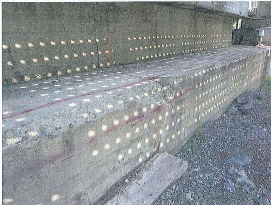
Photo 8 – Spalls on North Abutment
