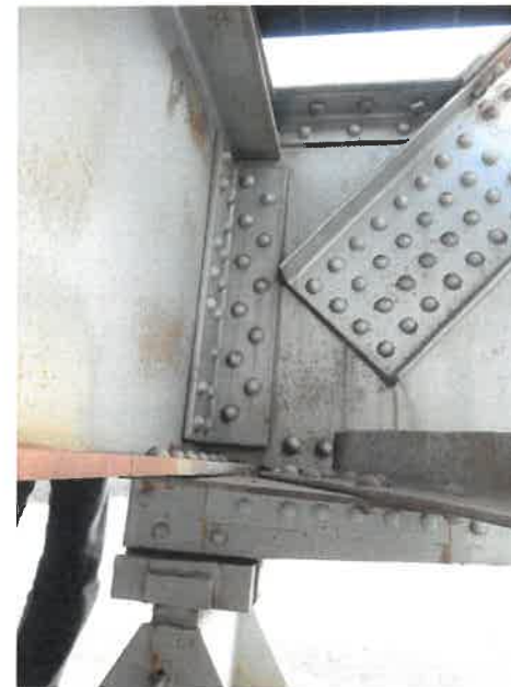
TYPICAL TRUSS END CONNECTION AT BEARING - 225 ft SPAN (200 ft SPAN FLOOR BEAM CONNECTION RIVET PATTERN DIFERENT)
