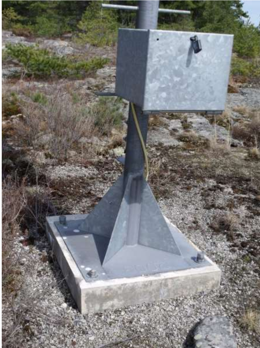
Figure 10: LL1028.5 Whitcher Island Rear Range – Existing foundation to be removed after new tower commissioned directly behind existing
