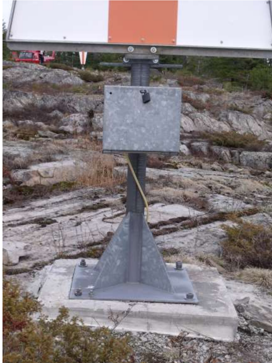
Figure 9: LL1028 Whitcher Island Front Range - Existing foundation to be removed after new tower commissioned directly behind existing
