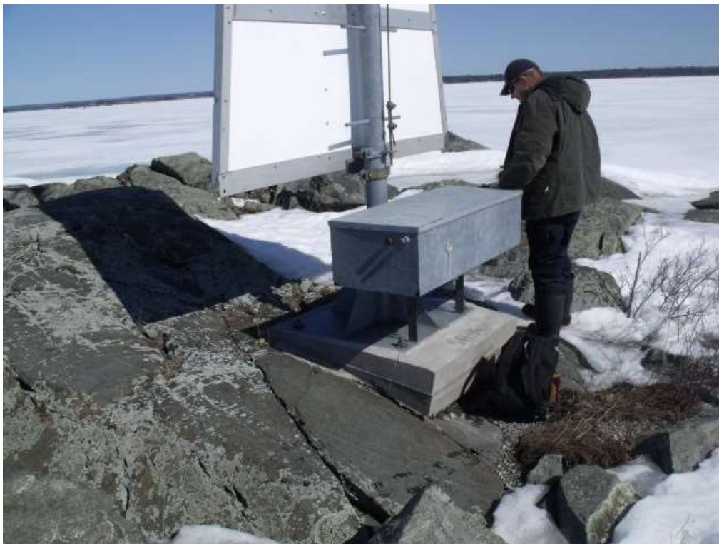
Figure 13: LL1029 Decelles Island Front Range – Tower to be placed in front of existing tower (where shadow is shown in photo) and old foundation removed after commissioning of new tower
