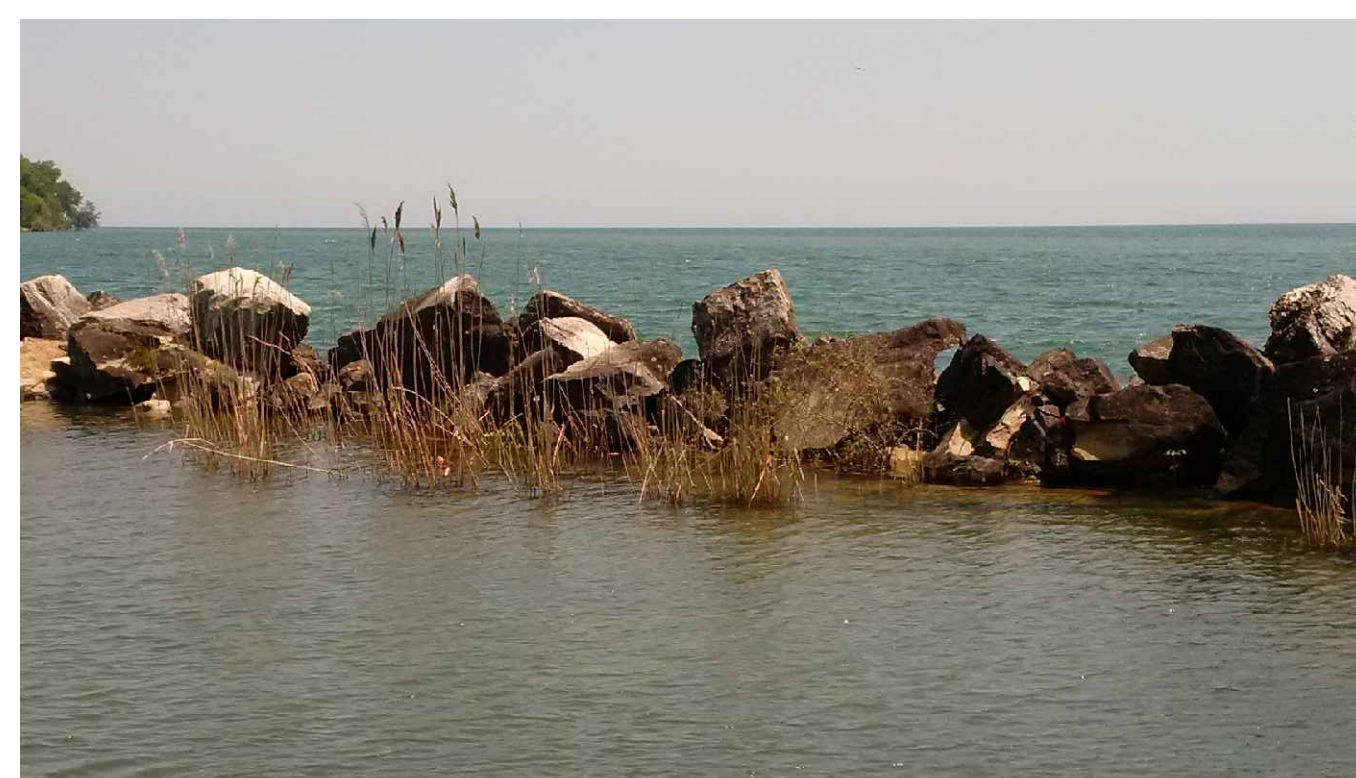
MAIN WEST BREAKWATER FAILURE - STA S 0+080 SCALE: NTS
