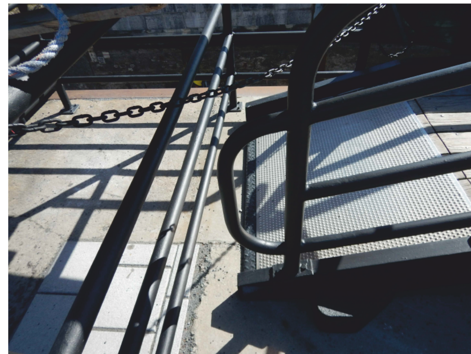
PHOTO 28-7704 PASSERELLE HORS SERVICE PICTURE 28-7704 OUT OF SERVICE FOOTBRIDGE
