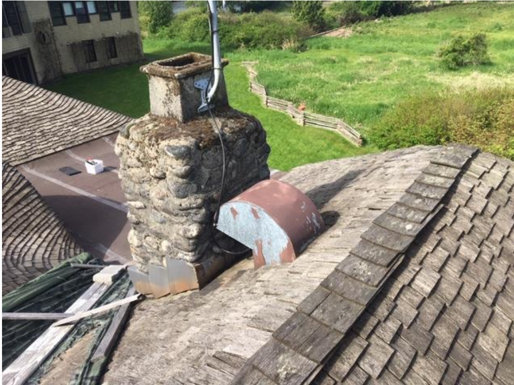
Lodge Building - Brown lead containing paint on roof vent.
