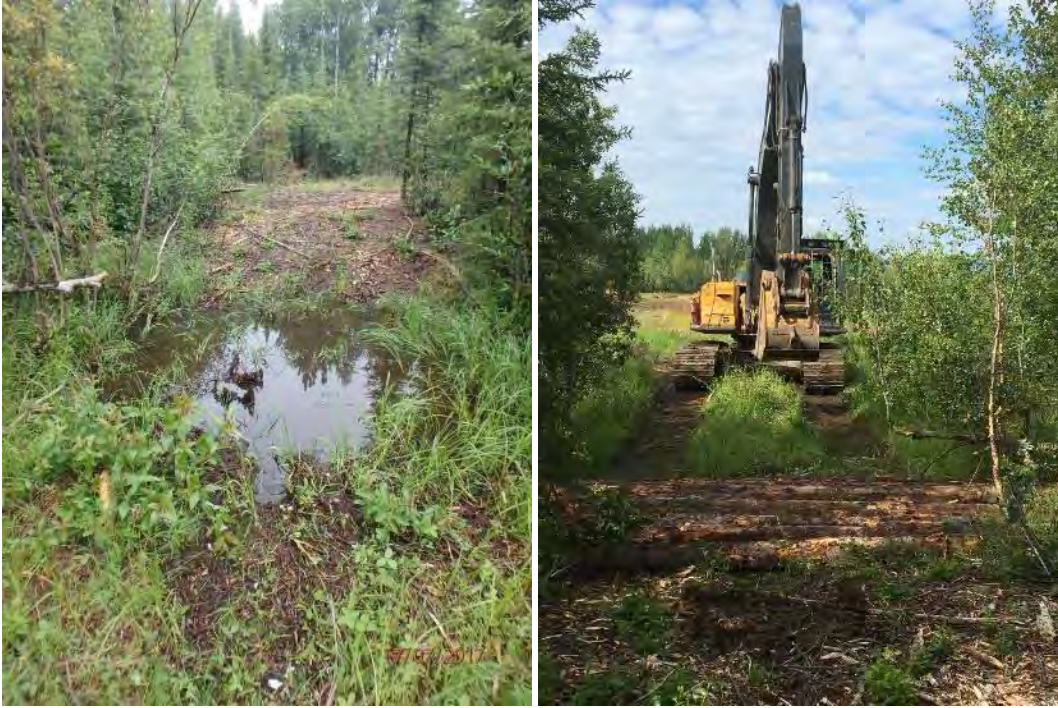
Photo 5: The swale at APEC 27, which collected water during rainfall before the crossing and during construction of the temporary crossing on 19 July.
