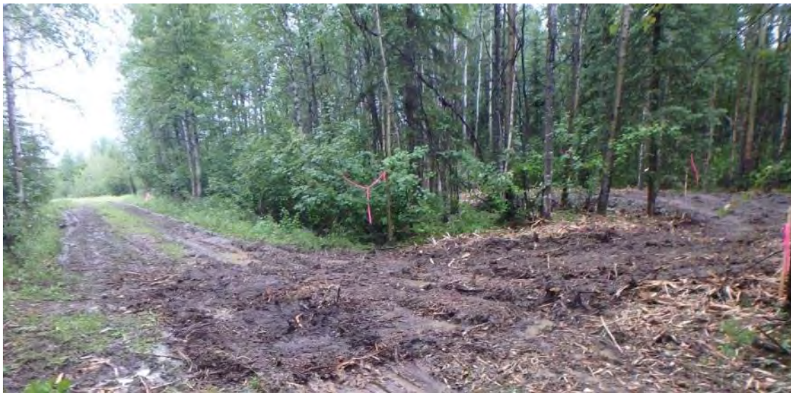
Photo 7: Above shows the rutting that occurs when the excavator turns when leaving a site. Below is after the excavator has smoothed the surface and added mulch.
