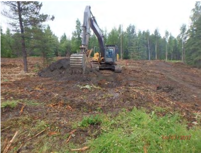
Photo 6: Excavator replacing soil into a completed test pit in the reverse order it was taken so that topsoil remains at the surface.
