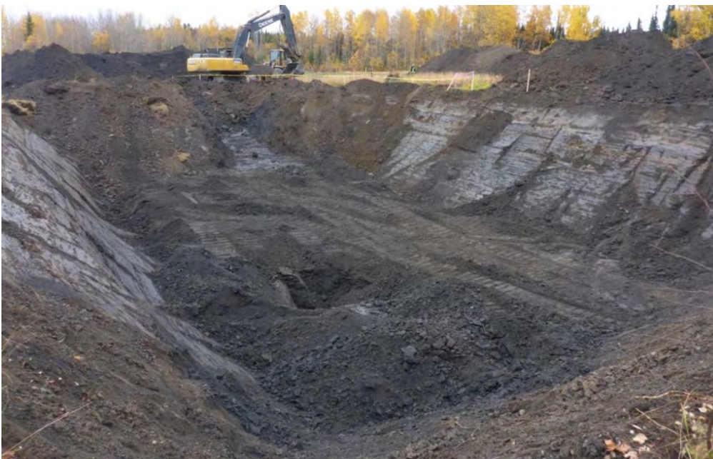
Photo 4: Excavation to 4 metres below ground surface (m bgs) of inferred impacted material from southwestern corner of AEC 1B looking towards the north-east.
