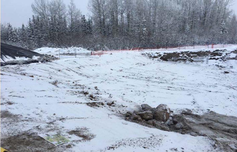
Photograph 1: AEC 1C Cells F8, G8 to G11 polyed with sloped backfilled material looking east
