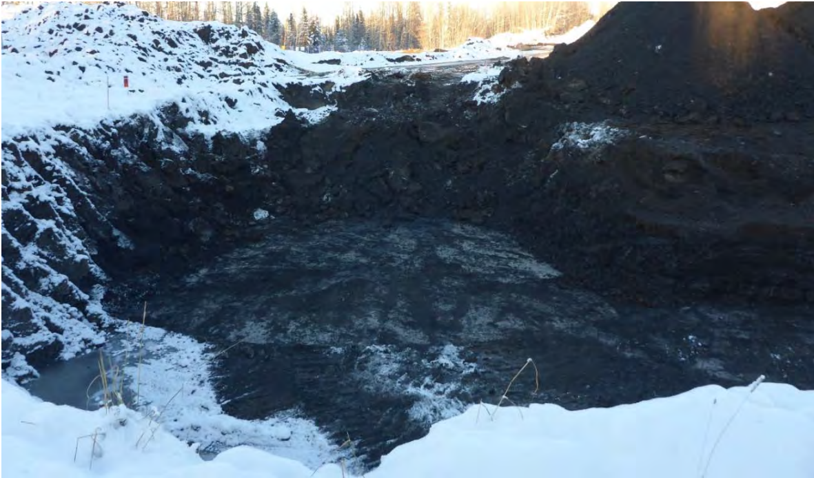
Photo 35: Continued excavation of inferred impacted material along western edge of AEC 1C looking towards the north.
