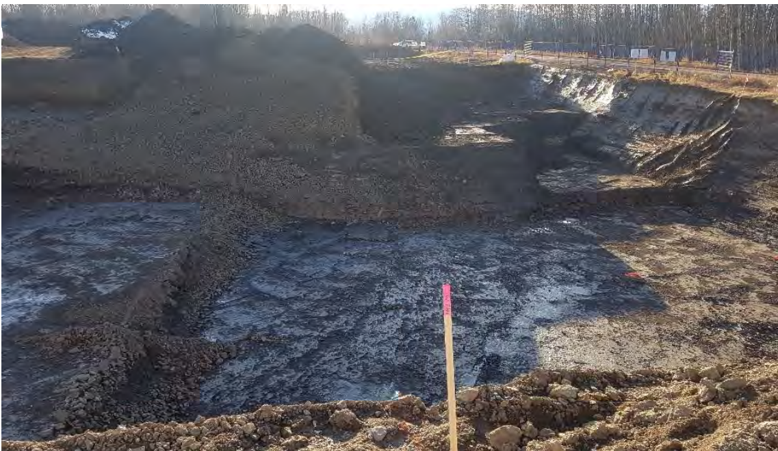
Photo 16: Excavation of inferred impacted material from western edge of AEC 1B looking towards the south-west.
