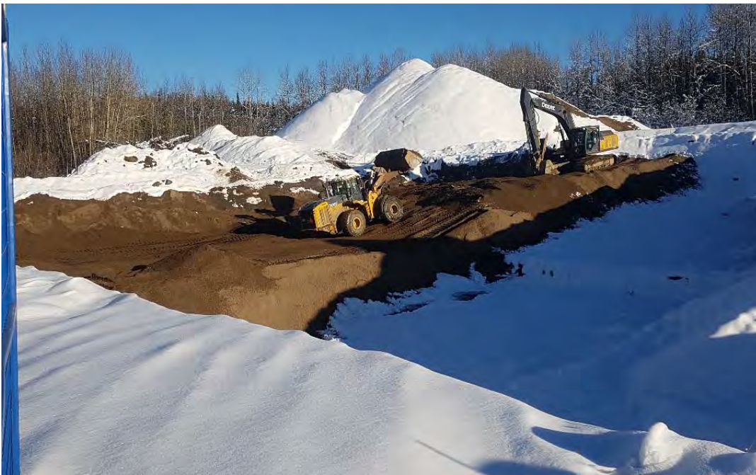
Photo 24: Continued backfilling of northern portion of AEC 1B looking towards the north-east.
