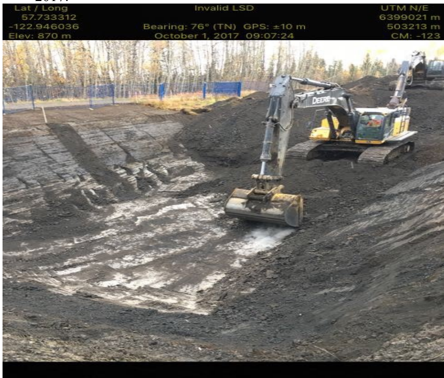
Photograph No. 2 – Photograph 2 Showing nice clean sloping and wide open excavation. No signs of sloughing, groundwater or tension cracking. Fencing in place along roadway. October 1 st , 2017.
