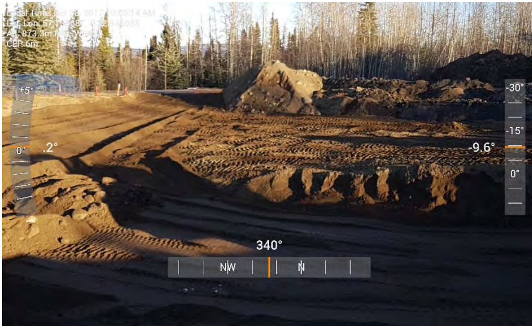
Photo 27: Continued backfilling of northern portion of AEC 1B looking towards the north.
