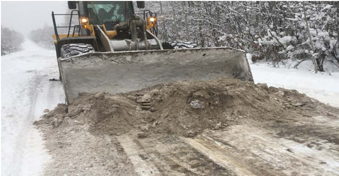
Photograph 2: Removed material from coolant spill. Material was placed with stockpile to be hauled off-site.
