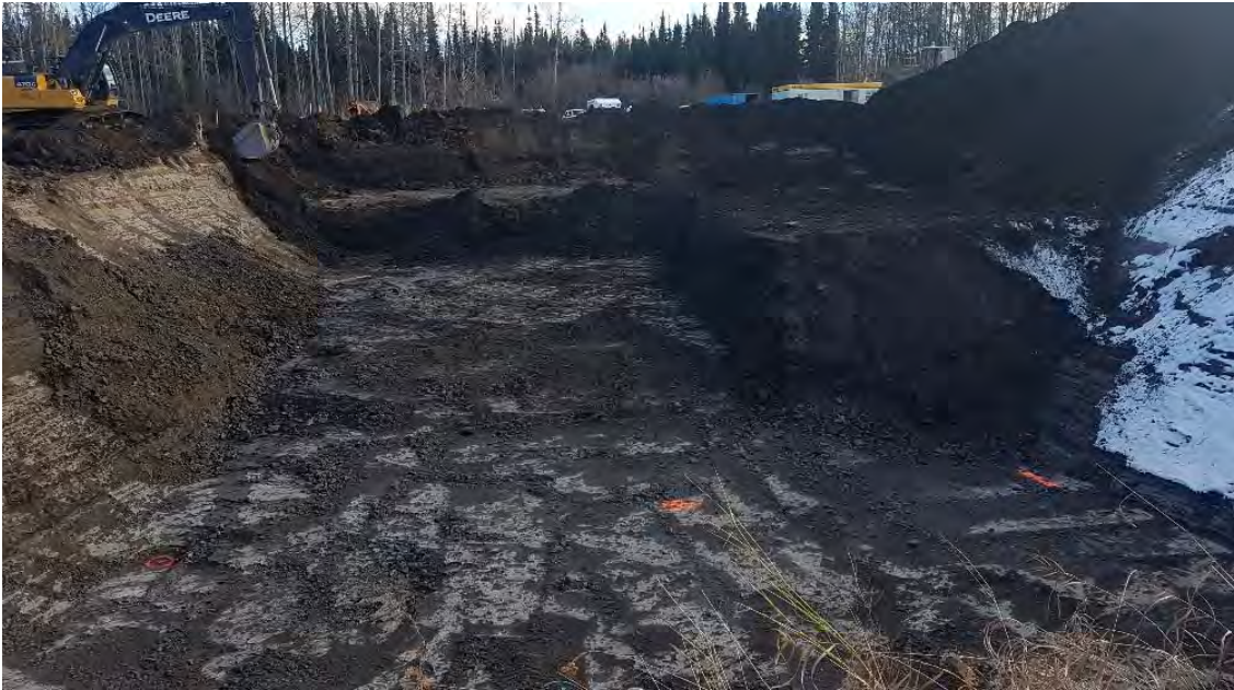
Photo 13: Continued excavation of inferred impacted material in eastern portion of AEC 1B looking towards the east.
