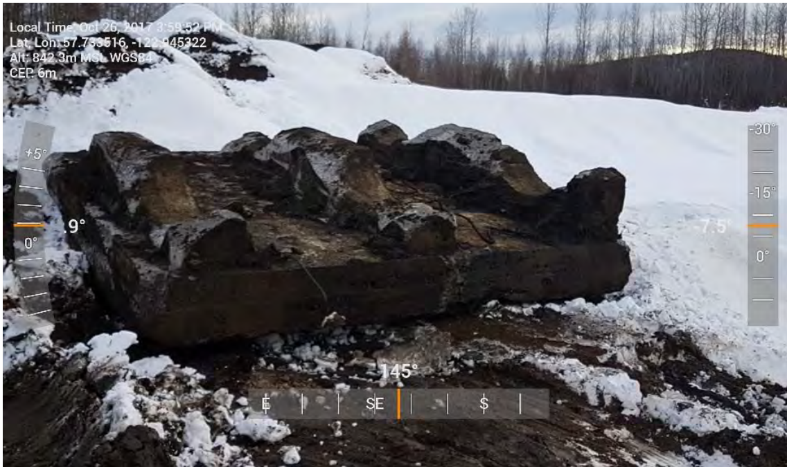
Photo 25: Concrete removed near the western edge of AEC 1B looking towards the south-east.
