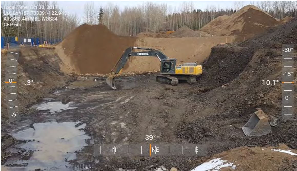
Photo 29: Continued excavation of central portion of AEC 1B looking towards the north-east.
