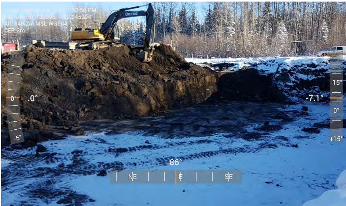
Photo 38: Continued excavation of central portion of AEC 1C looking towards the east.
