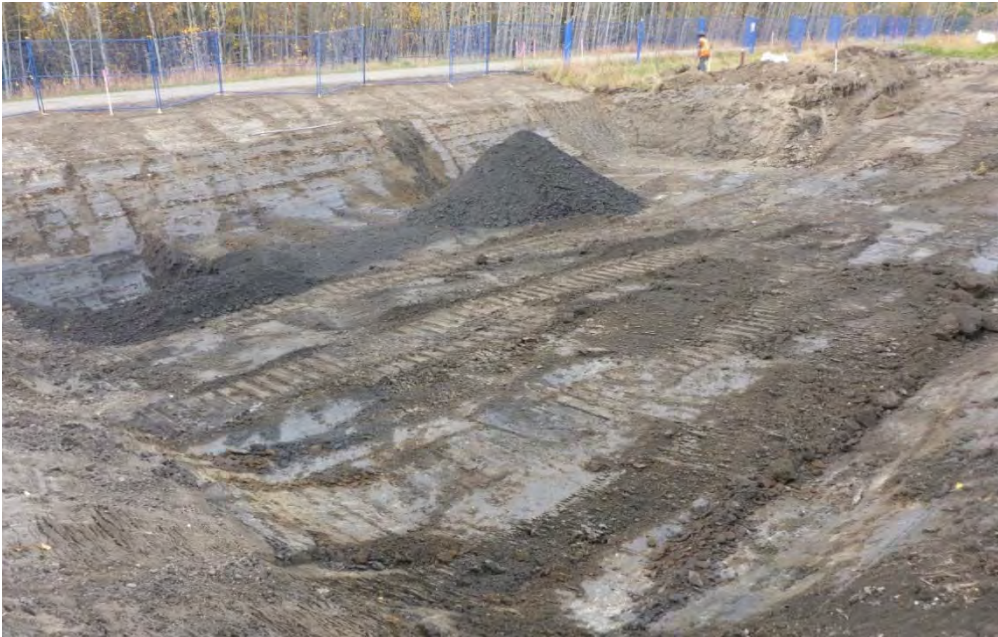
Photo 3: Excavation of inferred impacted material in western portion of AEC 1B looking north-west towards old Alaska Highway alignment.
