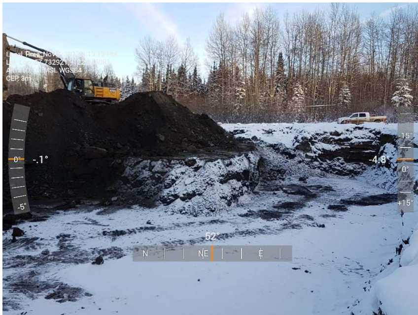
Photograph 2: Excavation in AEC 1c including cells, B7 to B8, C7 to C10 and D7 to D10, looking northeast
