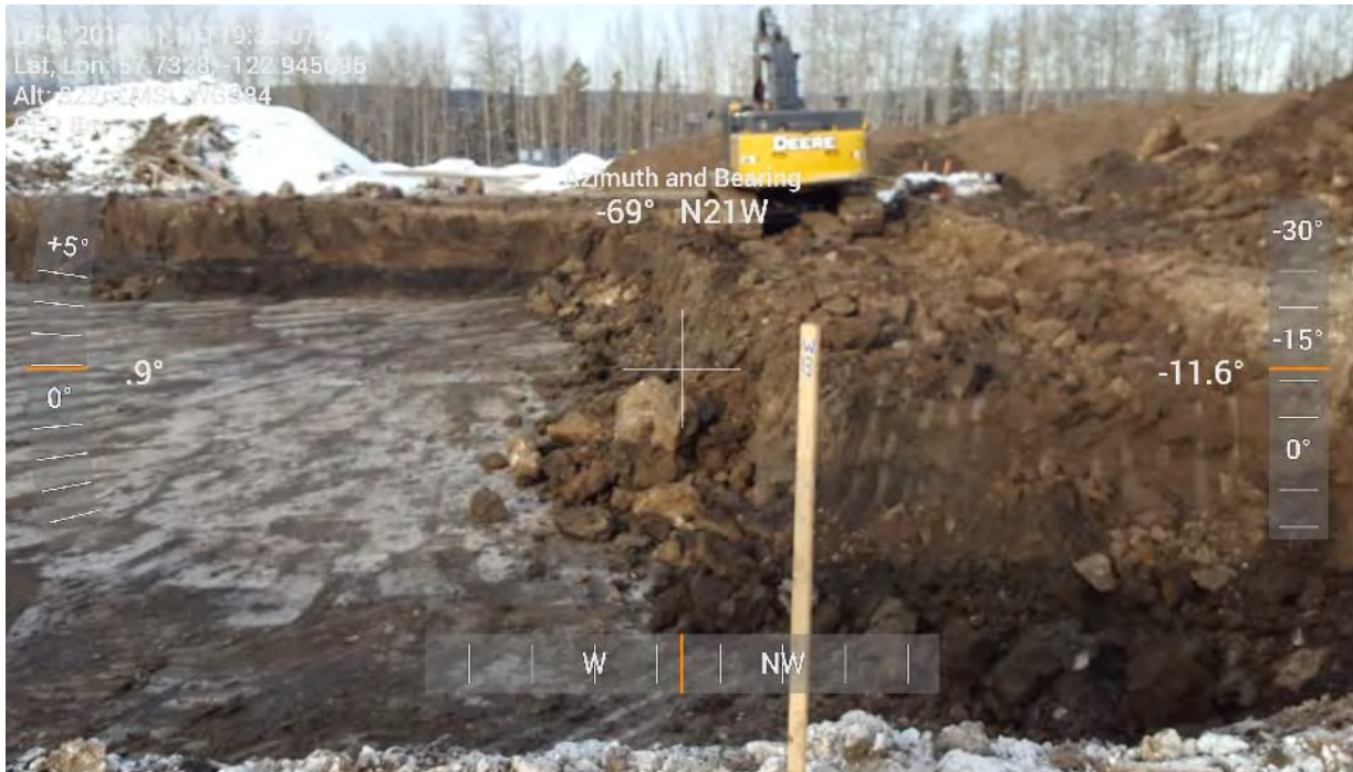
Photo 41: Excavation of inferred impacted material from eastern portion of AEC 1C looking towards the west.
