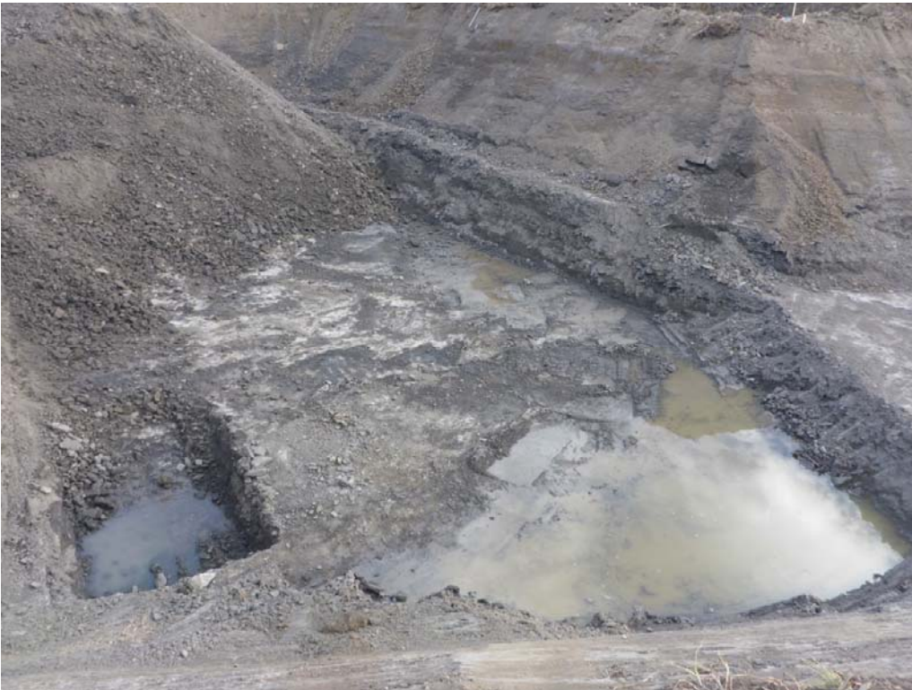
Photograph 4: Water seepage in AEC 1b in cells G2, H2, I2.
