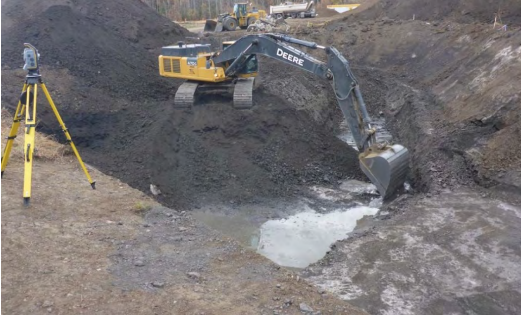
Photo 7: Excavation to 6 m bgs of inferred impacted material from central portion of AEC 1B looking towards the north-east.
