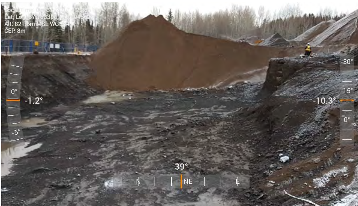
Photo 30: Continued excavation of central portion of AEC 1B looking towards the north-east.
