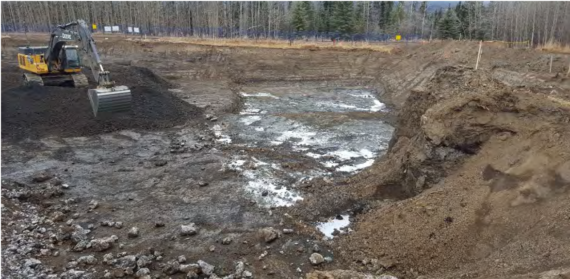
Photo 19: Continued excavation of inferred impacted material from eastern portion of AEC 1B looking towards the west.
