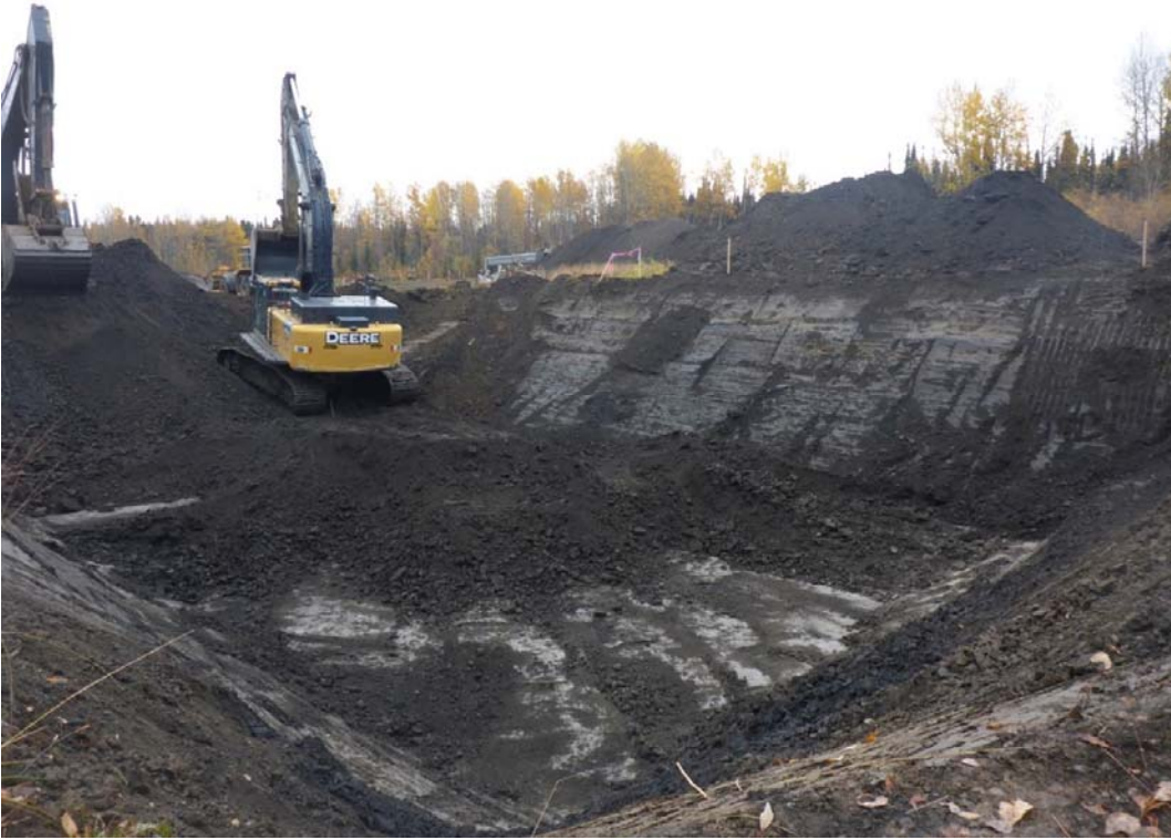
Photograph 1: Excavation in AEC 1b to approximately 5mbgs in cells E2, E3, F2, F3, G2, G3, looking east.
