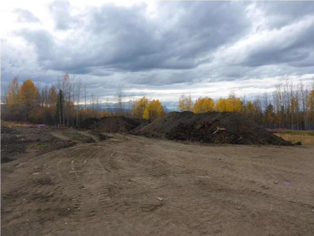
Stockpiles generated from overburden removed from cells E2, E3, F2, F3, G2, G3
