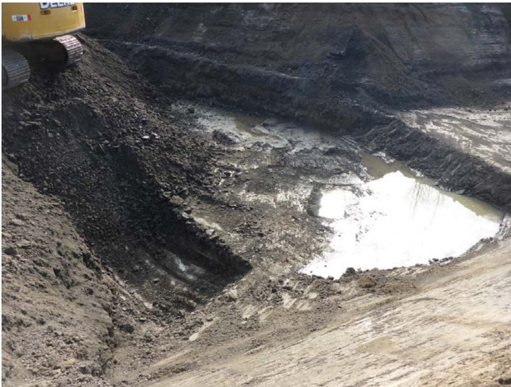
Photograph 2: Test pit in cell H2 to determine feasibility of excavating to approximately 6 mbgs.
