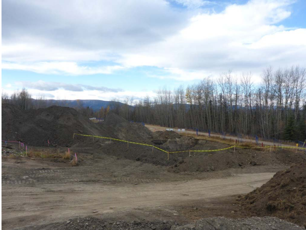
Photograph 1: AEC 1b including the excavation in cells N2, N3, O2, O3, P2, P3, looking west.
