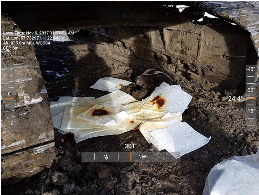
Photograph 1: Spill pads deployed to capture hydraulic fluid leaking from John Deere 470G LC excavator, looking northwest.
