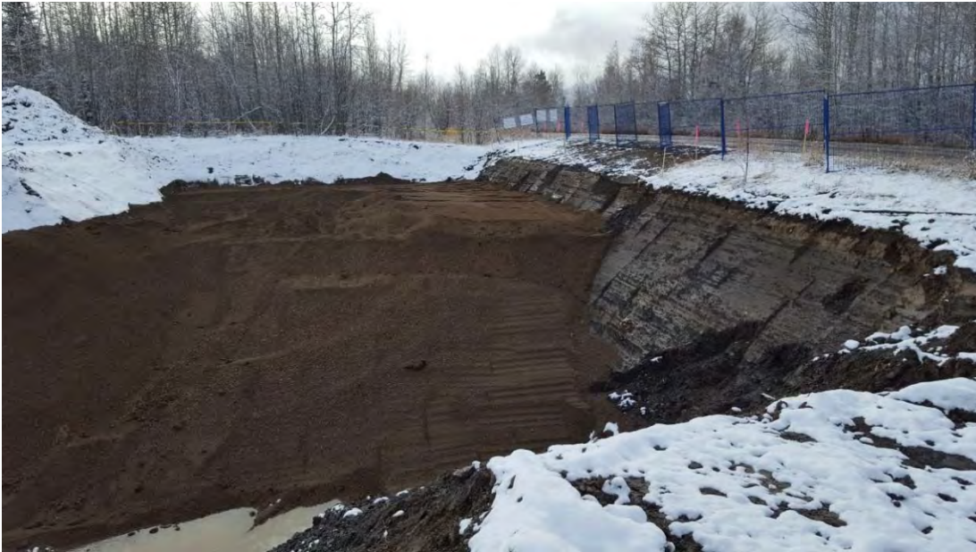
Photo 11: Continued backfilling of southern portion of AEC 1b looking towards the south.
