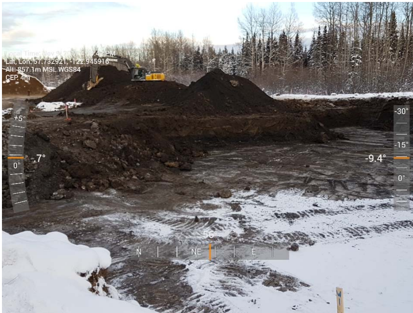
Photograph 1: Excavation in AEC 1c including cells C8 to C10, D7 to D10, E9 to E11 and F9 to F11, looking northeast.
