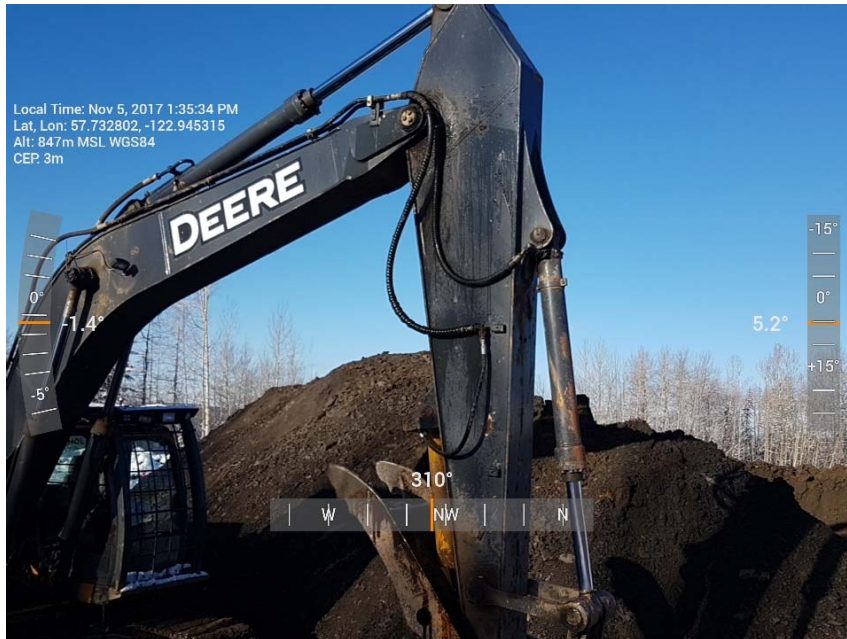
Photograph 2: Hydraulic line leak on John Deere 350G LC excavator, looking northwest
