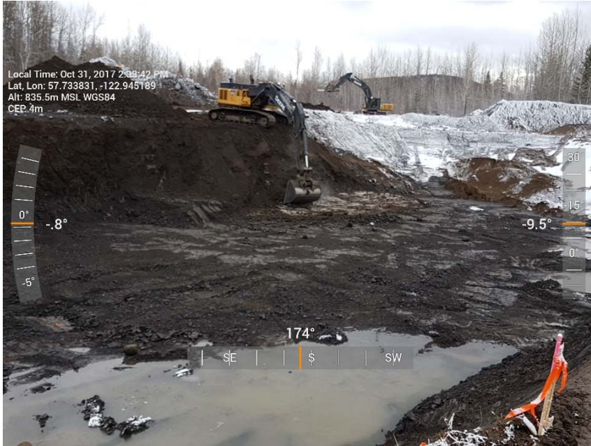
Photograph 1: Excavation in AEC 1b including cells H3 to H5, I3 to I5, J3 to J5 and K3 to K5, looking south
