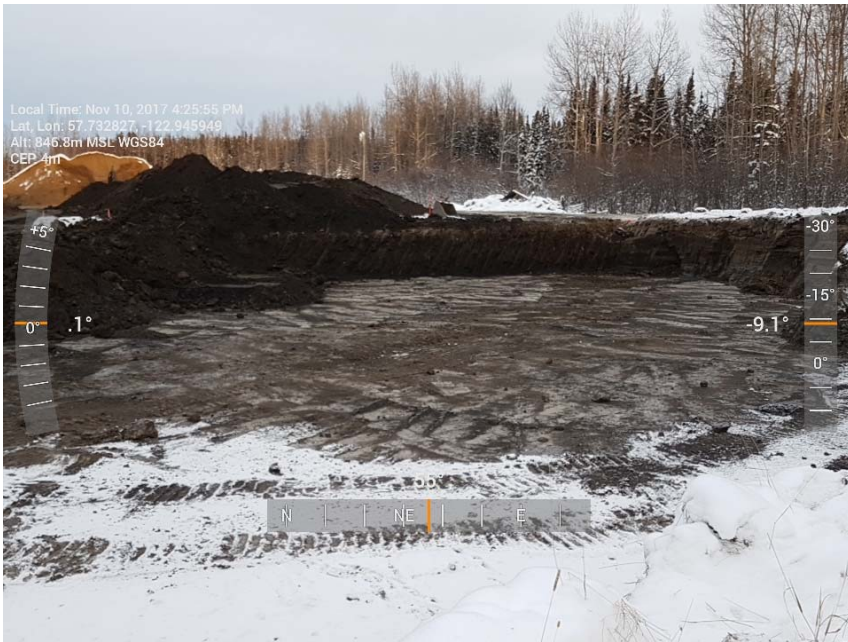
Photograph 1: Excavation in AEC 1c including cells C8 to C10, D7 to D10, E9 to E11 and F8 to F11, looking northeast.
