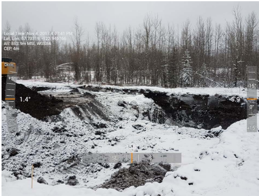
Photograph 1: Excavation AEC 1c including cells B7 to B9, C7 to C10 and D7 to D10, looking southeast.
