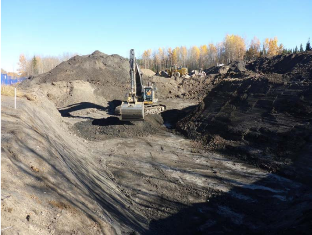
Photograph 1: Excavation in AEC 1b in cells E2, E3, F2, F3, G2, G3, H2, H3, H4 and I4 looking east.
