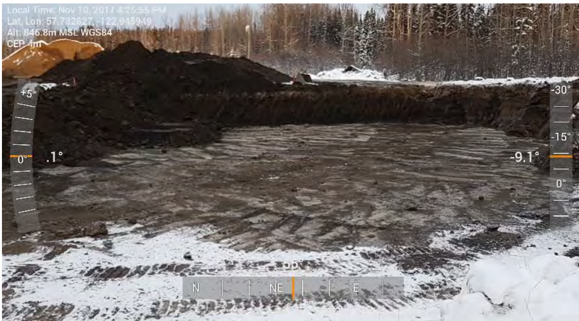
Photo 40: Excavation of inferred impacted material from eastern edge of AEC 1C looking towards the north-east.
