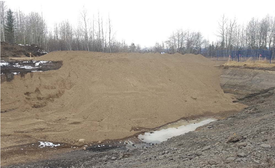
Photograph 2: completed haul road in AEC 1b, cells being backfilled E2, E3, F2, F3, G2, G3, H2, H3, H4, I2, I3 and I4 looking southwest
