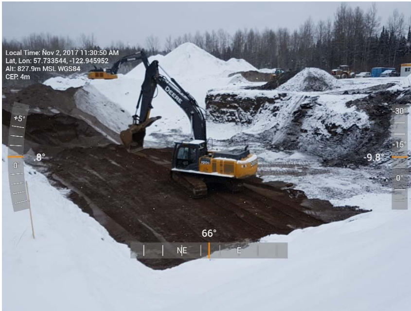
Photograph 1: Backfilling in AEC 1b including cells H2 To L2, H3 to L3, H4 to L4 and H5 to L5, looking east
