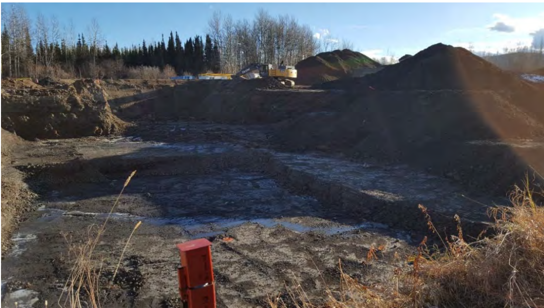
Photo 18: Continued excavation of inferred impacted material from eastern portion of AEC 1B looking towards the south-east.
