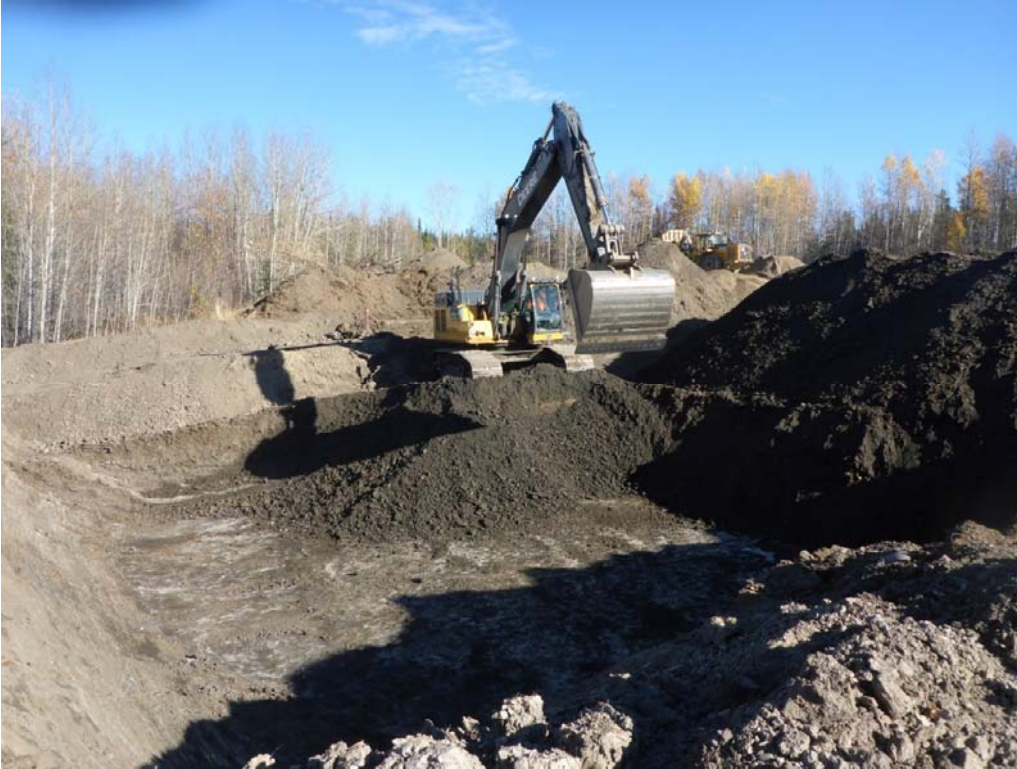
Photograph 3: Excavation in AEC 1b to approximately 4 mbgs in cells N2, N3, O2, O3, P2, P3, looking east.
