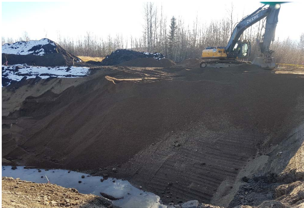
Photograph 2: new haul road in AEC 1b, cells being backfilled E2, E3, F2, F3, G2, G3, H2, H3, H4, I2, I3 and I4 looking southeast
