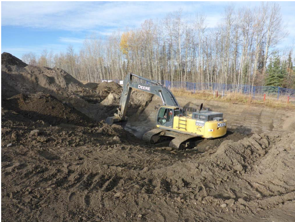
Photograph 2: Excavation in AEC 1b in cells O3 and P3 to 4 mbgs, looking west.
