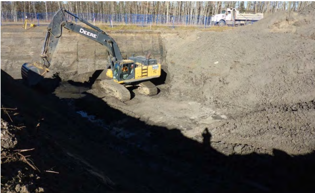
Photo 8: Continued excavation to 6 m bgs of inferred impacted material from central portion of AEC 1B looking towards the west.
