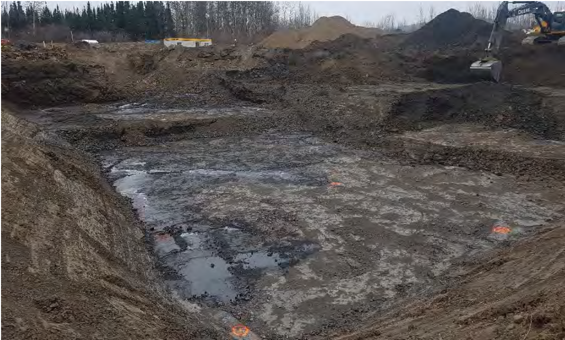
Photo 17: Continued excavation of inferred impacted material from eastern portion of AEC 1B looking towards the south-east.
