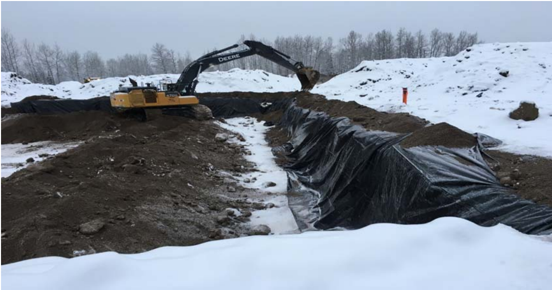
Photograph 1: AEC 1C Cells F8, G8 to G11 polyed with sloped backfilled material looking northwest
