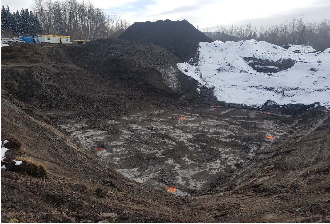
Photograph 1: AEC 1b including cells N2 to N5, O2 to O5 and P2 to P5 looking south
