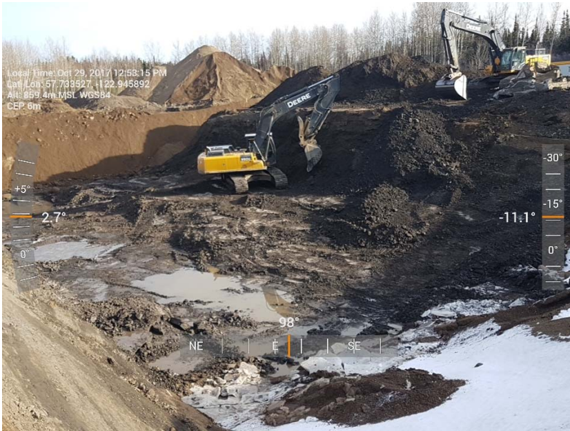
Photograph 1: Excavation AEC 1b including cells H2 to H5, I2 to I5, J2 to J5, K2 to K5 and L2 to L5, looking east.
