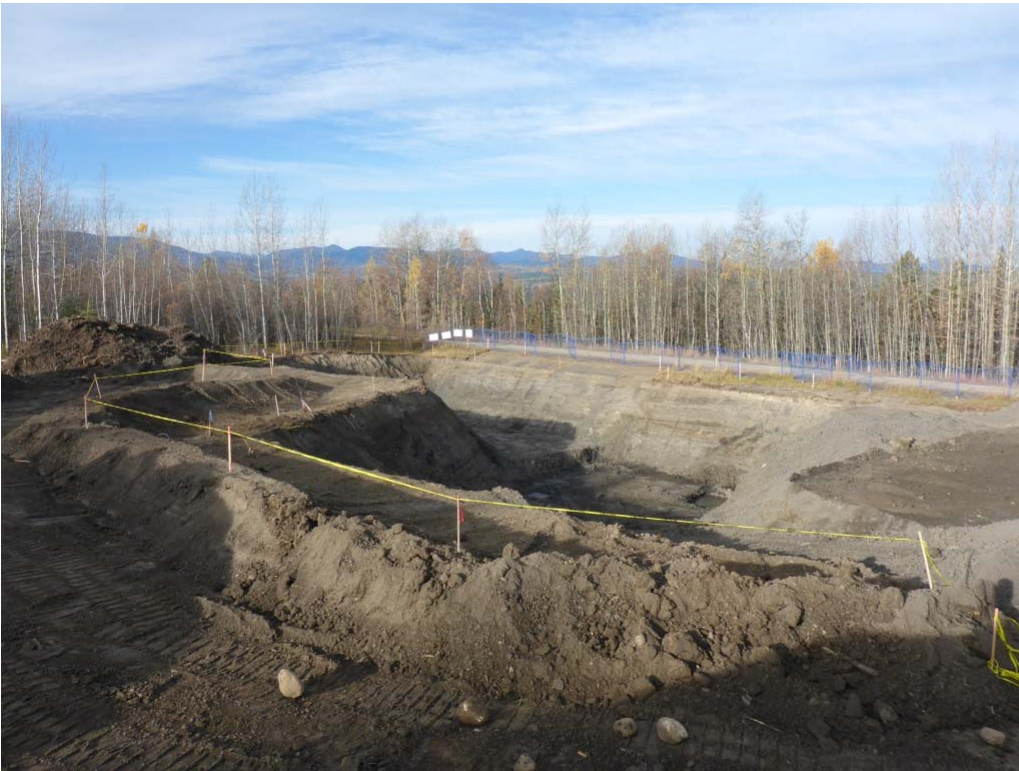
Photograph 1: AEC 1b including the excavation in cells F2, F3, G2, G3, H2, H3, H4, I2, I3, I4, looking west.
