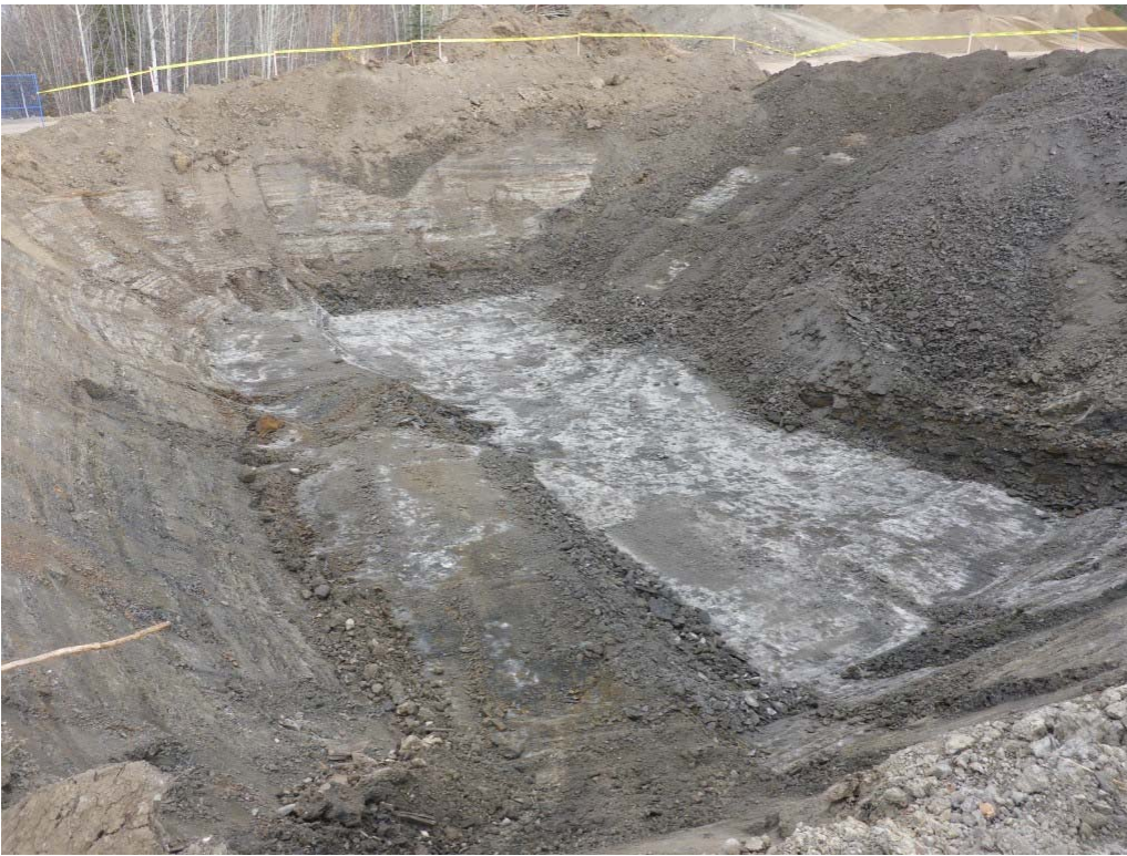
Photograph 3: Excavation in AEC 1b including cells N2, N3, O2, O3, P2, P3, looking east.
