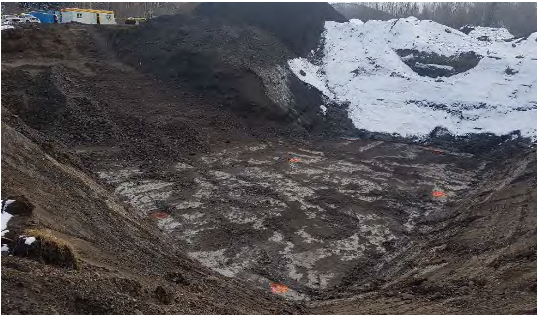
Photo 12: Excavation of inferred impacted material to depth of 5 m bgs in northern portion of AEC 1B looking towards the south-east.
