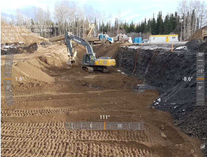
Photograph 1: Backfilling AEC 1b including cells O2 to O7 and P2 to P7, looking east.
