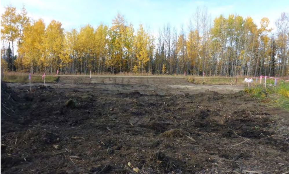
Photo 1: Preliminary excavation of surface material (mulched wood, shrubs, grasses) in AEC 1B looking west towards the former Alaska Highway alignment.
