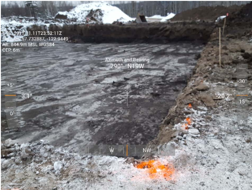
Photograph 1: Excavation AEC 1c including cells E11 to E8, F11 to F8, and G11 to G8, looking west.
