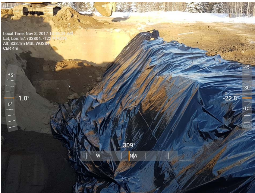
Photograph 2: Liner placed in cells P4 to P6 in AEC 1b, looking northwest
