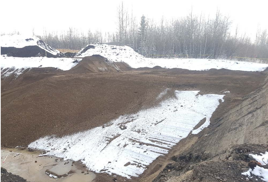
Photograph 2: AEC 1b including cells being backfilled E2, E3, F2, F3, G2, G3, H2, H3, H4, I2, I3 and I4 looking south
