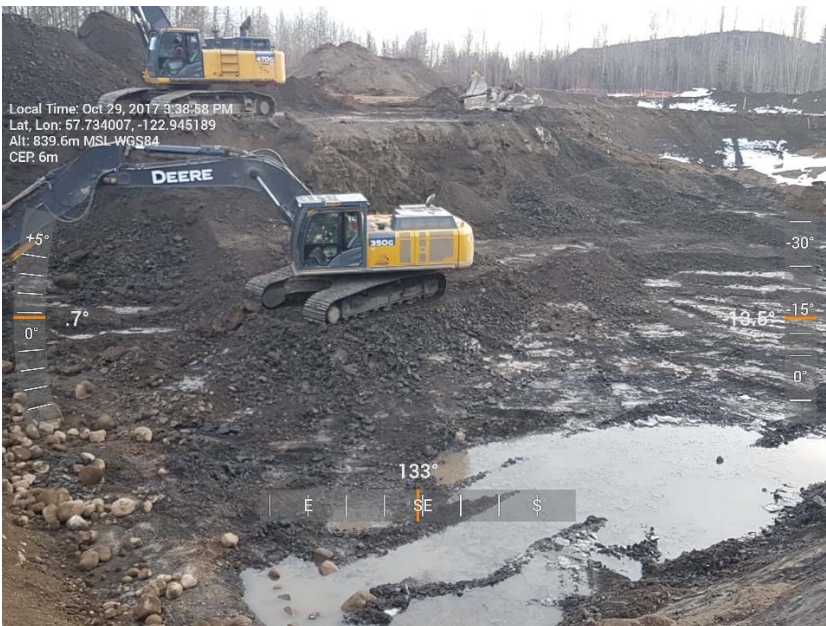
Photograph 1: Excavation AEC 1b including cells L2 to L5, K2 to K5, J3 to J5 and I4 to I5, looking southeast.
