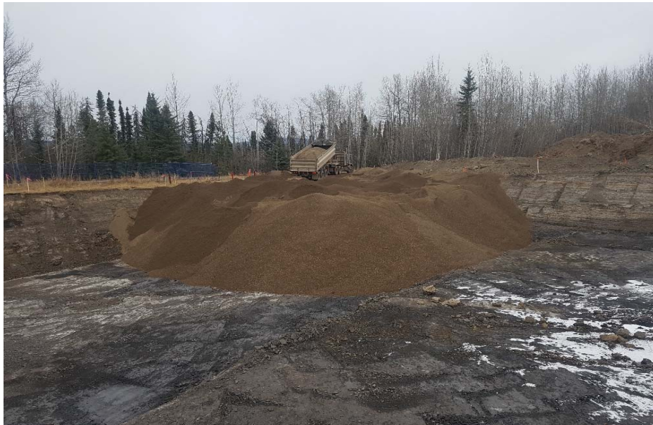
Photograph 2: Backfilling AEC 1b cell P2, P3 P4, O2, O3, O4, N2, N3 and N4 looking northeast
