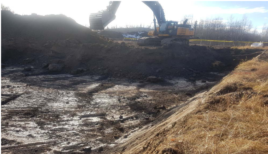
Photograph 2: AEC 1b including cells M2, M3, L2, L3 and K2 looking southeas
