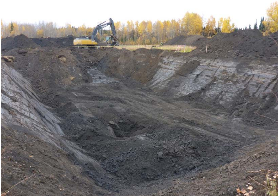
Photograph 2: Excavation in AEC 1b to approximately 4 mbgs in cells E2, E3, F2, F3, G2, G3, looking east.
