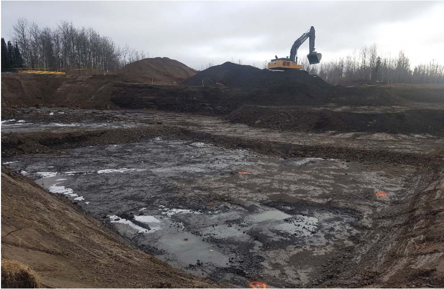
Photograph 1: AEC 1b including cells M2 to M7, N2 to N7, O2 to O7, P2 to P7, L2, L3 and K2 looking south
