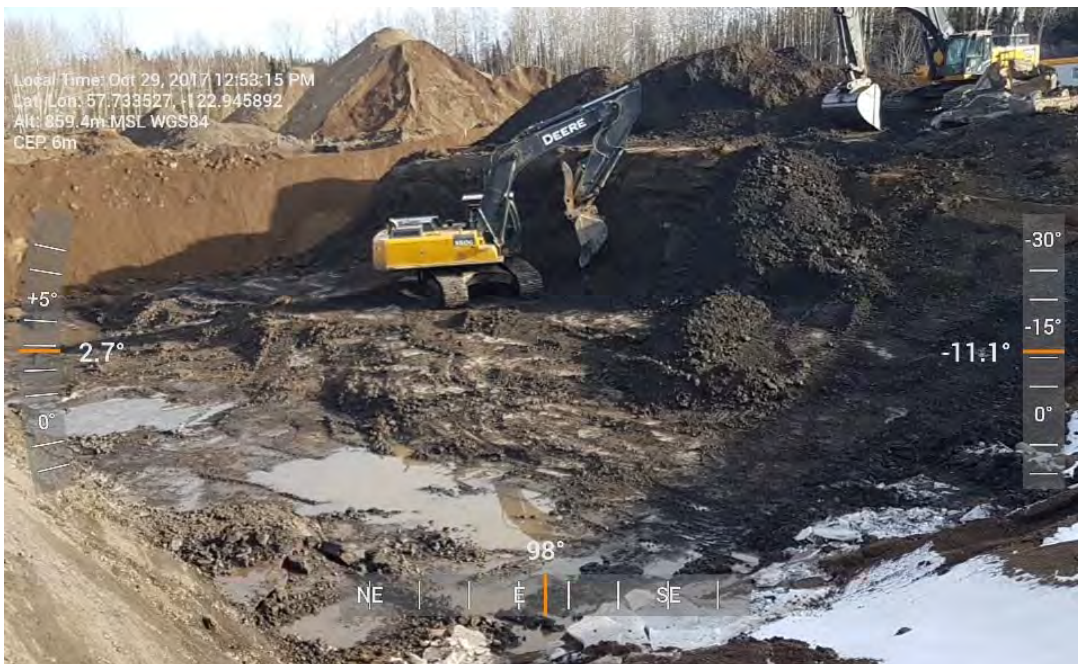
Photo 28: Continued excavation of central portion of AEC 1B looking towards the east.
