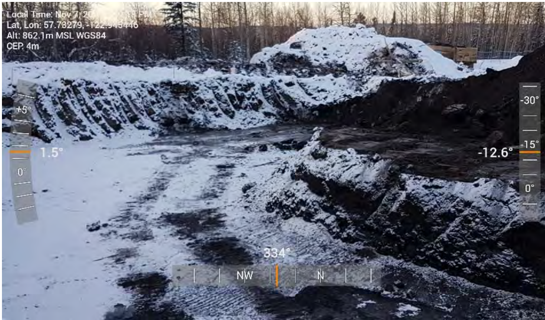
Photo 37: Continued excavation of central portion of AEC 1C looking towards the north-west.
