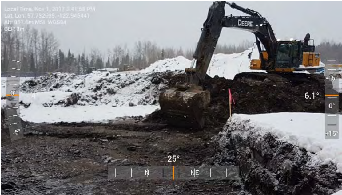
Photo 31: Excavation of inferred impacted material from the southern portion of AEC 1C looking towards the north-east.
