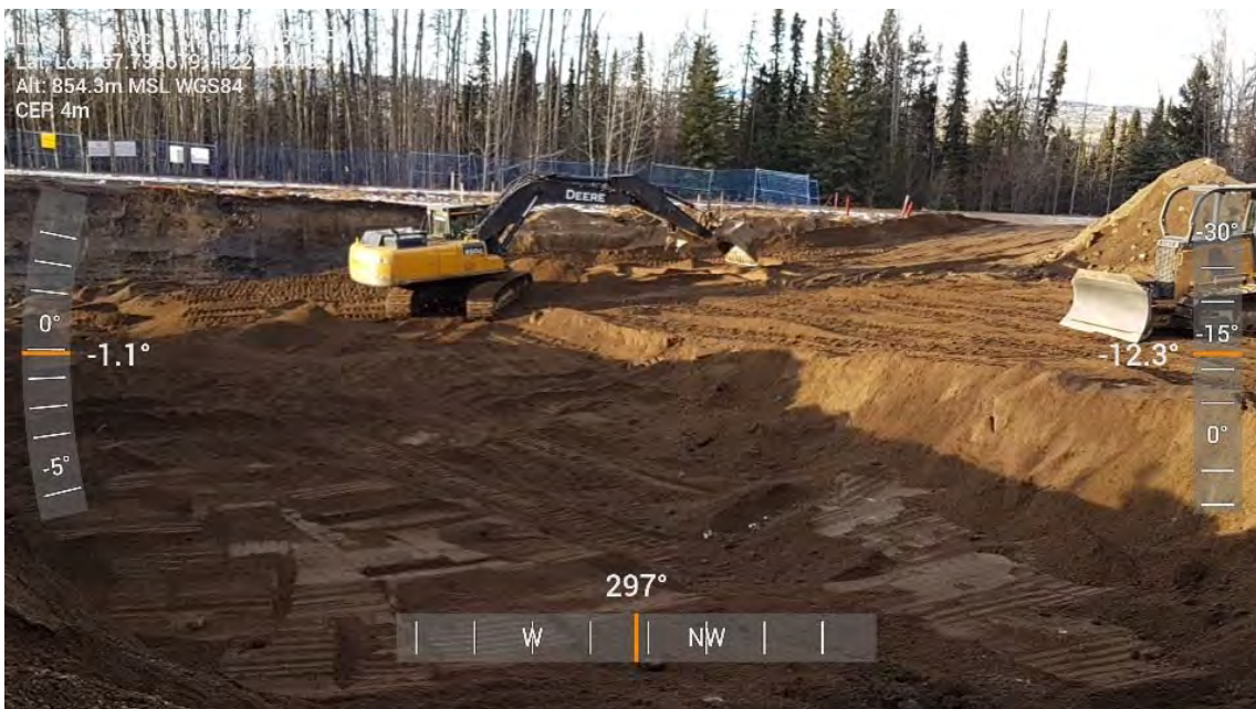
Photo 26: Continued backfilling of northern portion of AEC 1B looking towards the north-west.
