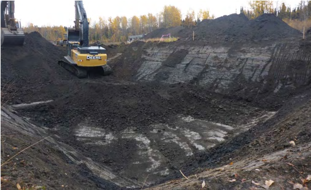
Photo 5: Excavation to 5 m bgs of inferred impacted material from southwestern corner of AEC 1B looking towards the north-east.
