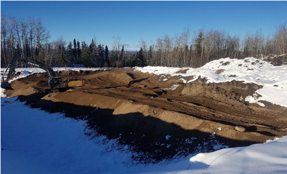
Photograph 2: Backfilling AEC 1b cell N2 to N5, O2 to O7 and P2 to P6 looking northwest
