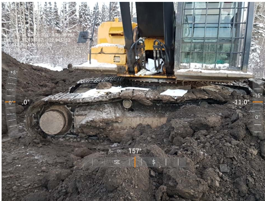
Photograph 2: Spill pads deployed to collect leaking hydraulic oil from the 350G LC excavator, looking south
