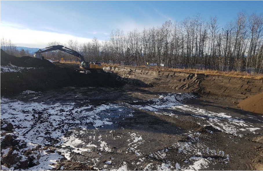
Photograph 1: AEC 1B including cells M2 to M7, N2 to N4, O2 to O4, P2 to P4, looking southwest
