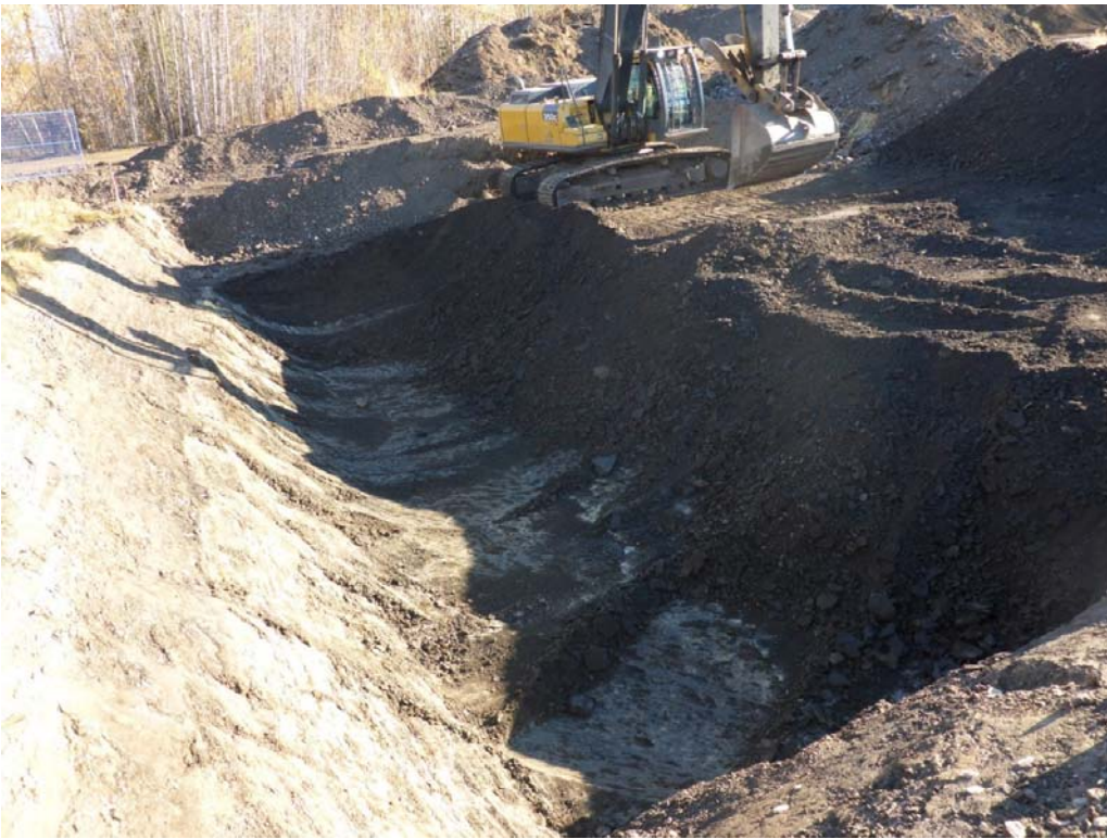
Photograph 3: Excavation in AEC 1b to approximately 3 mbsin cells N2, O2 and P2, looking east.
