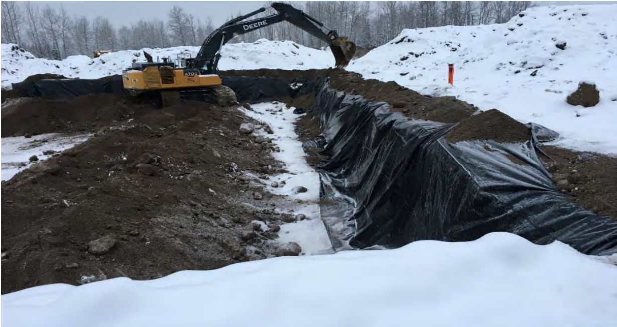
Photo 45: Installation of poly liner along north-east edge of AEC 1C looking towards the west.
