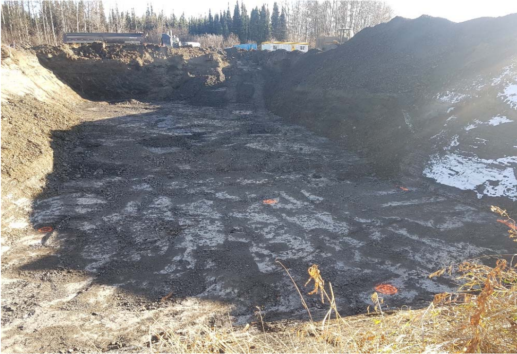
Photograph 1: AEC 1b including cells N2 to N5, O2 to O6 and P2 to P6 looking southeast
