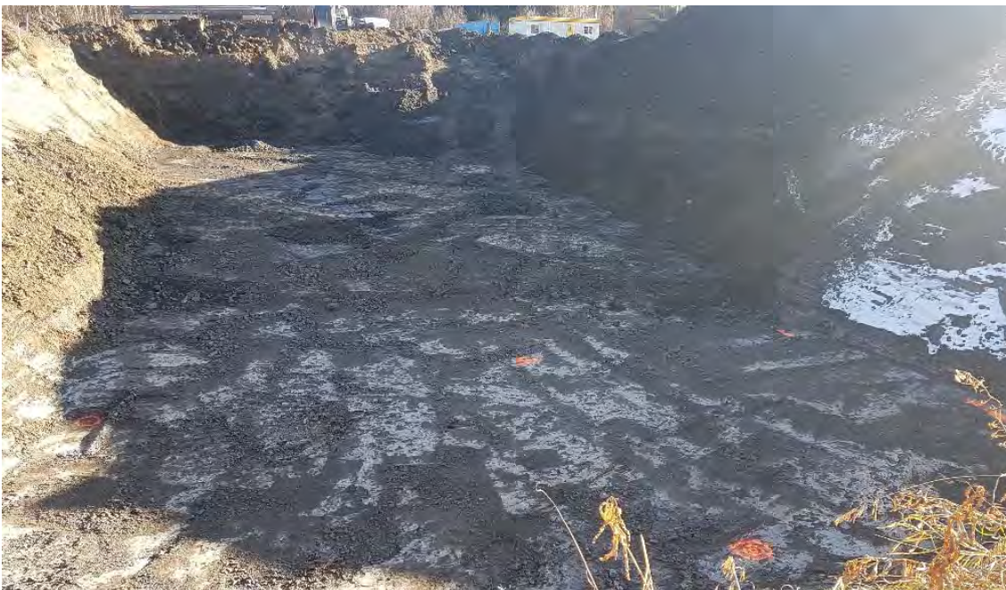
Photo 14: Continued excavation of inferred impacted material from eastern portion of AEC 1B looking towards the east.
