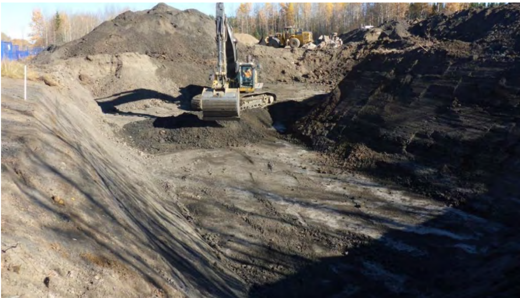
Photo 6: Continued excavation of inferred impacted material from southwestern portion of AEC 1B looking towards the north-east
