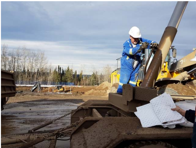
Photograph 2: Spill response to hydraulic fluid leak.
