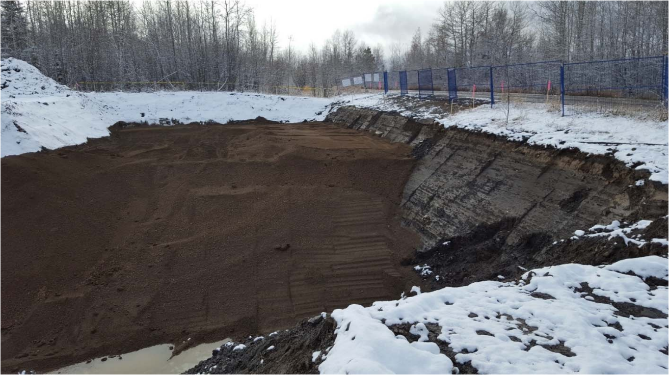
Photograph 1: AEC 1b including the backfilling of cells F2, F3, G2, G3, H2, H3, H4, I2, I3, I4, looking southwest.
