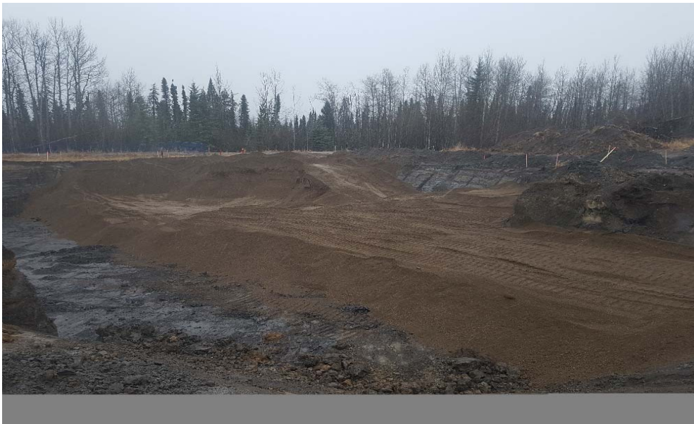
Photograph 2: Backfilling AEC 1b cell N2 to N5, O2 to O7 and P2 to P6 looking northwest
