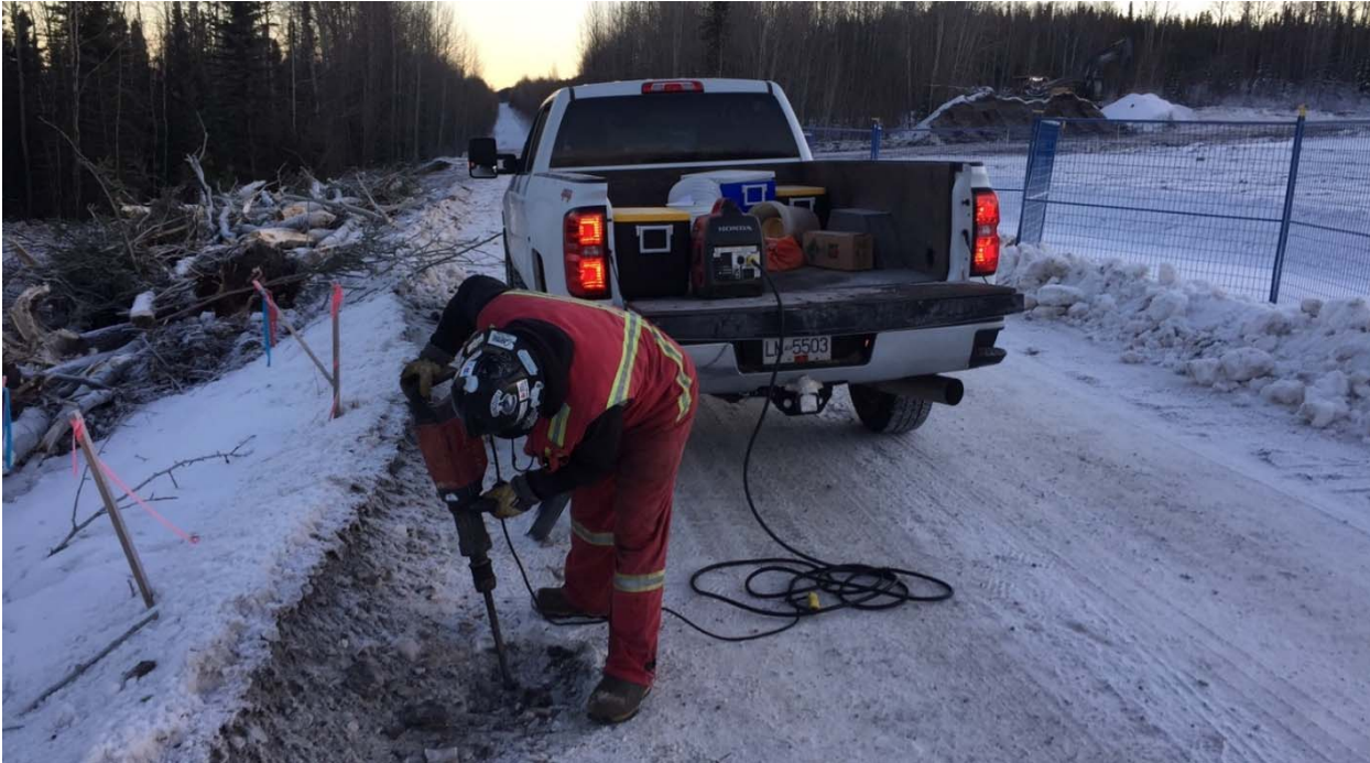
Photograph 9: Use of impact hammer to assess monitoring wells K19-MW17-29S/D along the former alignment. Looking north. 16 January 2018.
