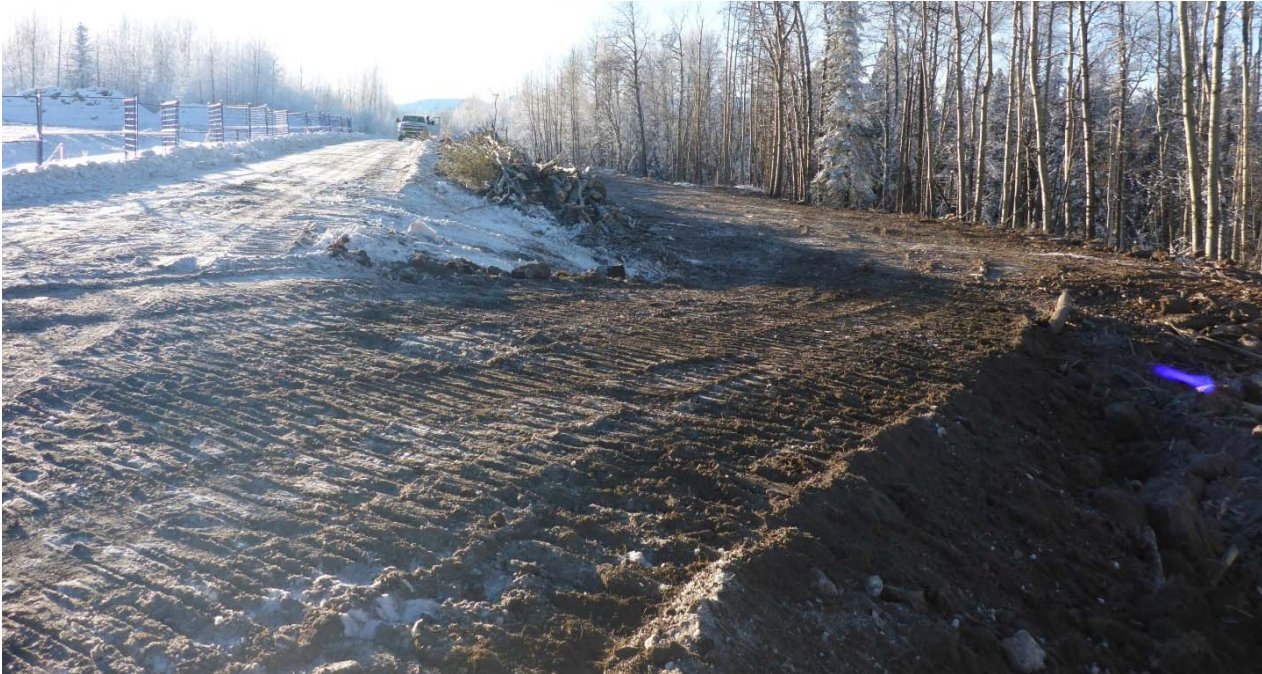
Photograph 3: Completed access road to the area west of the former alignment in AEC 1b, looking west. 12 January 2018.
