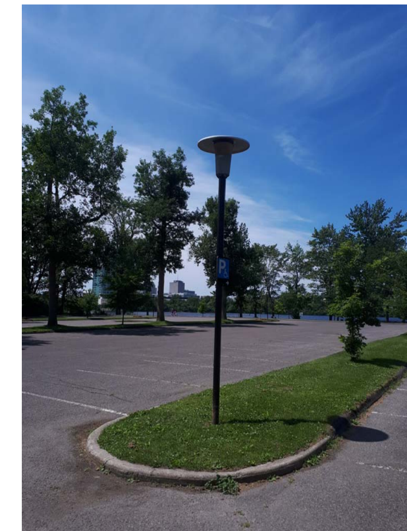
EXISTING LIGHT FIXTURE
