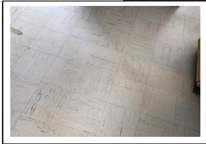
Photograph 1: Asbestos containing vinyl floor tiles and mastic in rooms EW6, EW15 and EW16 – Building 50
