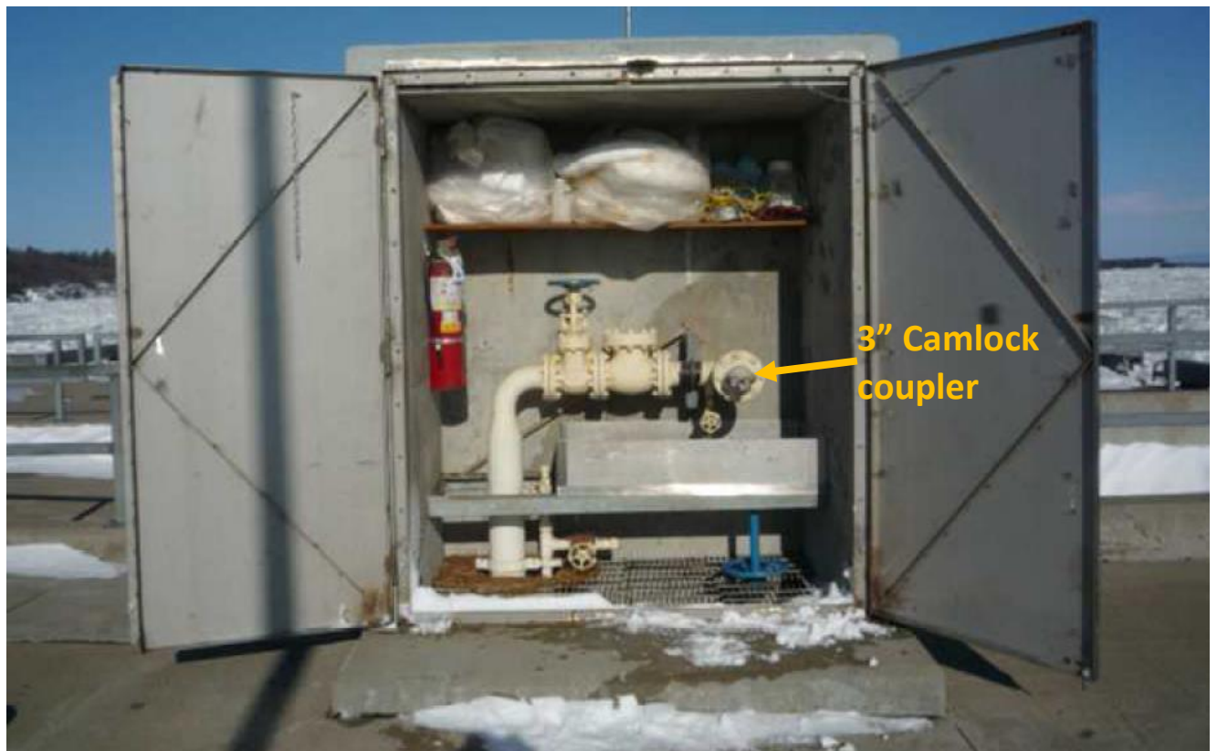
Connection point on the dock for the transfer of diesel fuel
