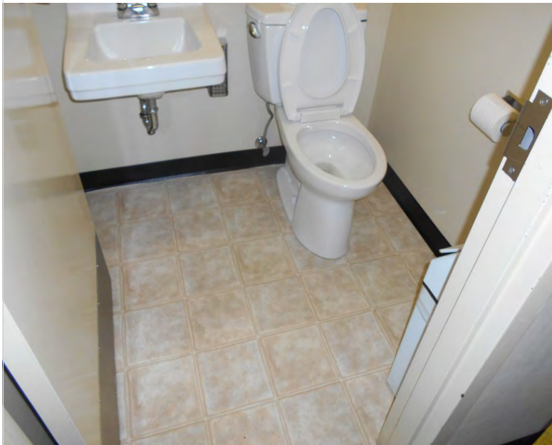
Washrooms 91270-99-989-000001 3 - Satisfactory condition-reliable N Mechanically washroom are in good working order no issues MEDIUM
