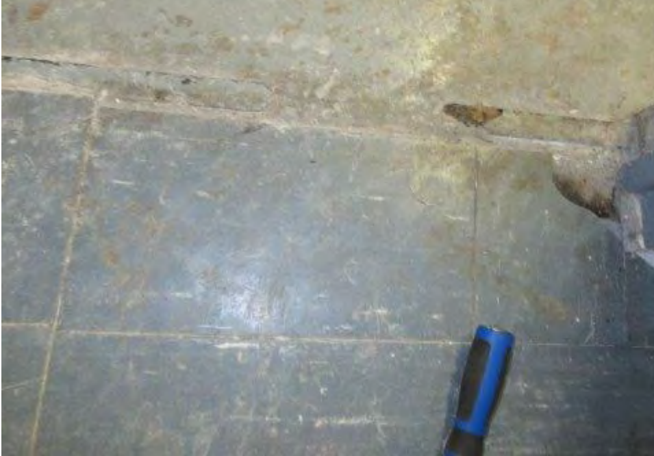
Photograph 3 Entrance to 126A Asbestos-containing grey vinyl door strip and underlying mastic (sample B3A)
