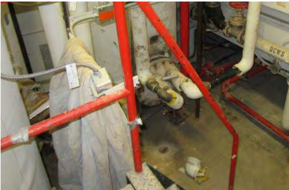
Photograph 4: Room 126A Non-asbestos fiberglass insulation applied to pipes and elbows. White wall paint (sample BL1). Red railing paint (BL5). Gasket (sample B1). Asbestos-containing refractory brick and gaskets may be present in hot water tank.
