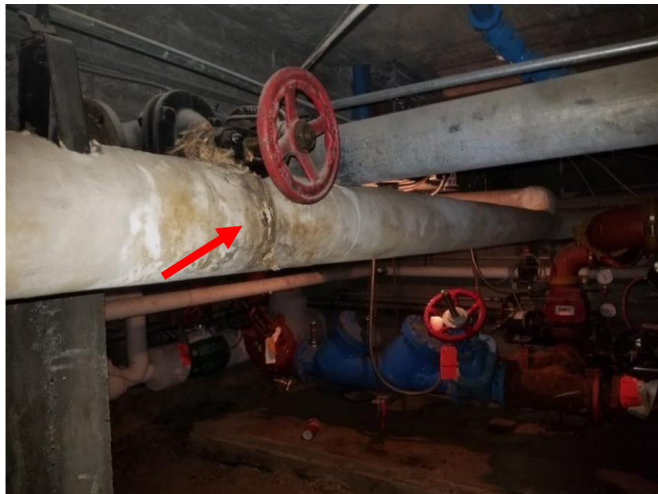
Photo 2. Basement, crawlspace, east-central, <1 square metre fair condition fitting.
