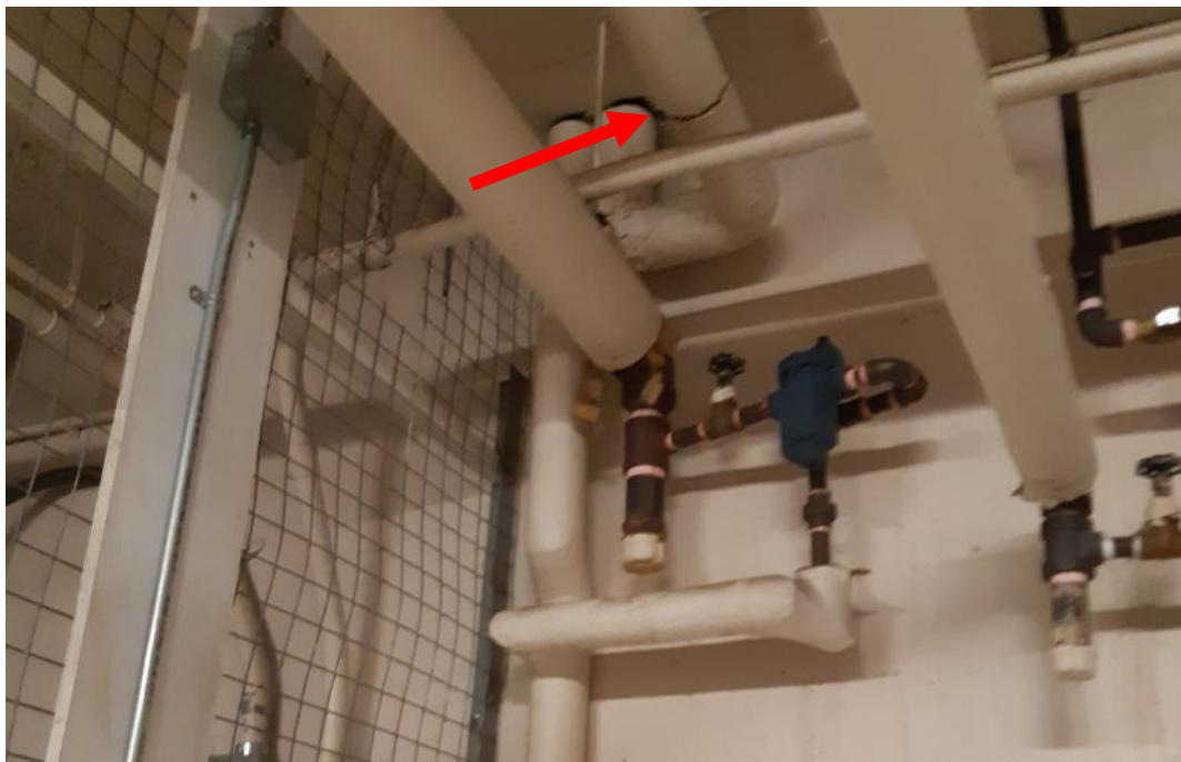
Photo 6. Basement, lab 15, north-west corner of room next to gated area, <1 linear metre fair condition Aircell.
