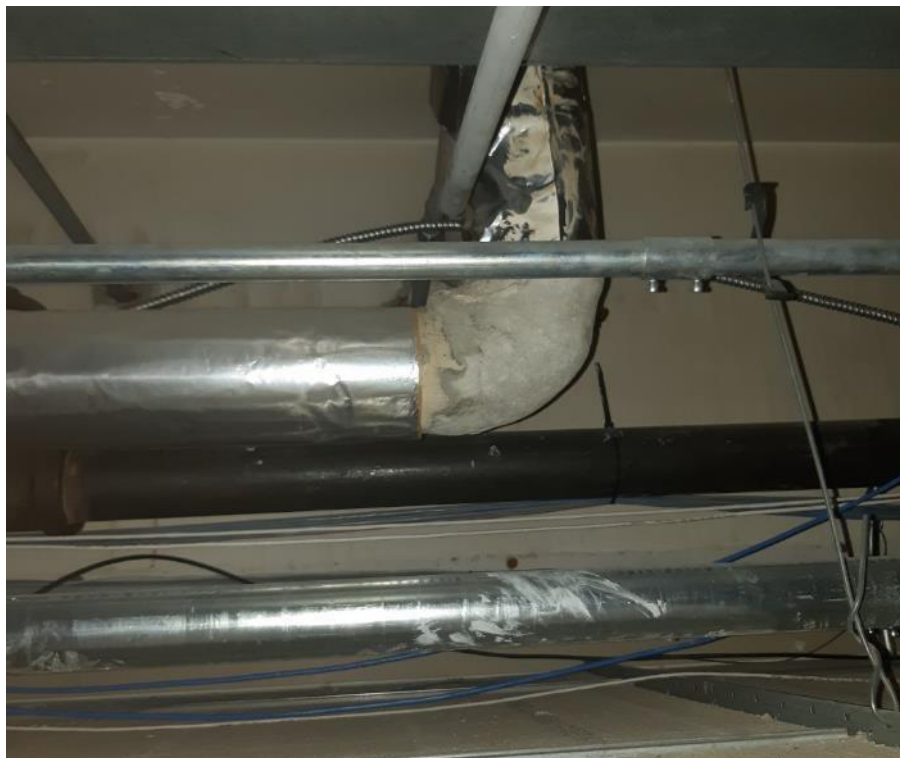
Photo 4. Basement, main hallway, in front of fire hose across from room 102, 1 fair condition pipe fitting.
