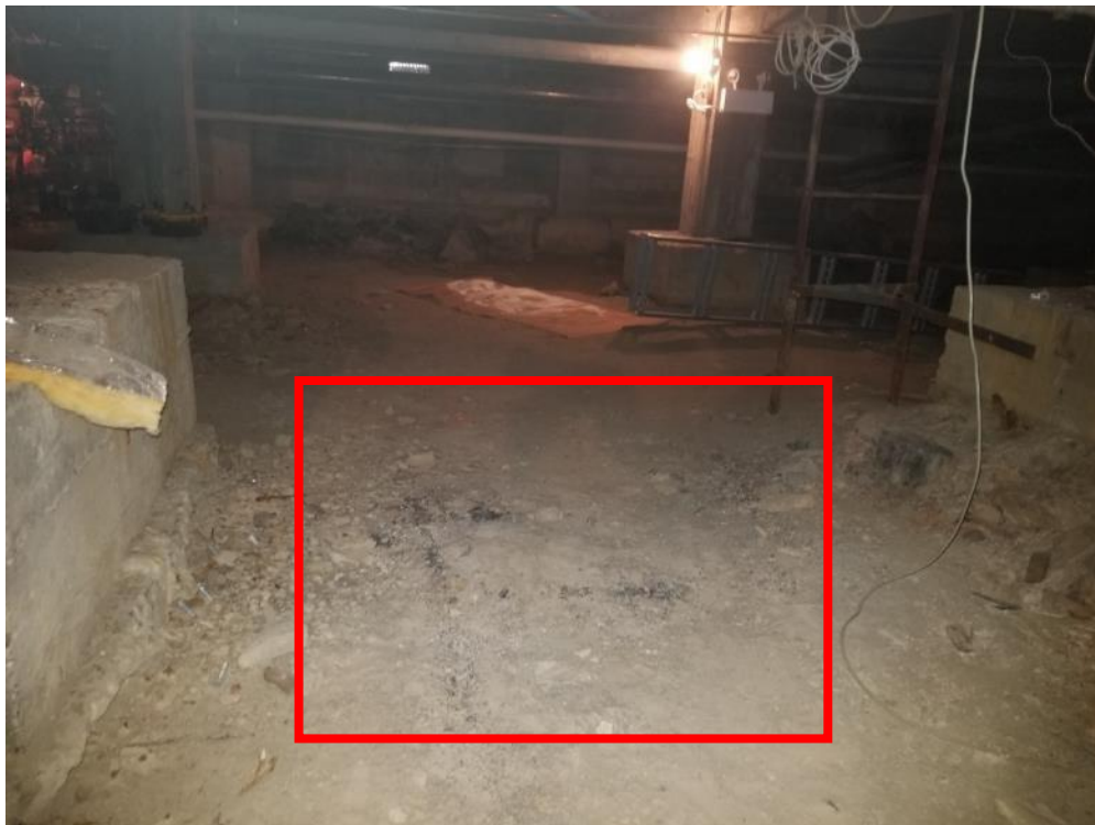
Photo 4. Basement, crawlspace, central behind ladder, 1 square metre Aircell debris on floor.
