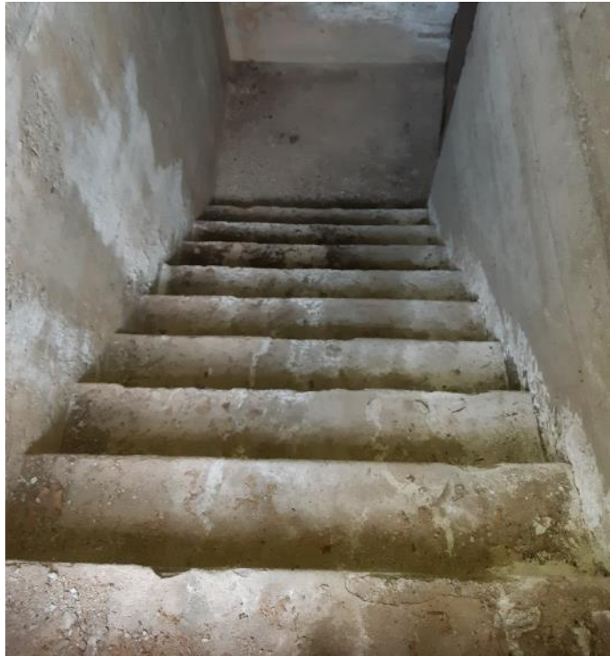
Photo 1. Basement, floor near entrance, 4 square metres debris on stairs.
