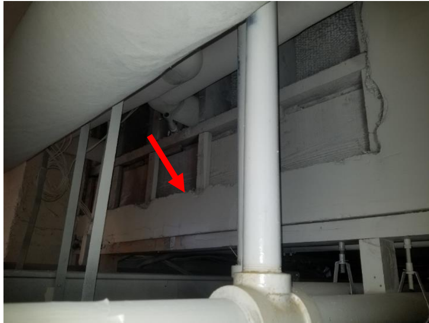
Photo 1. Basement, file secure room, south wall, 2 square metres poor condition ceiling plaster.
