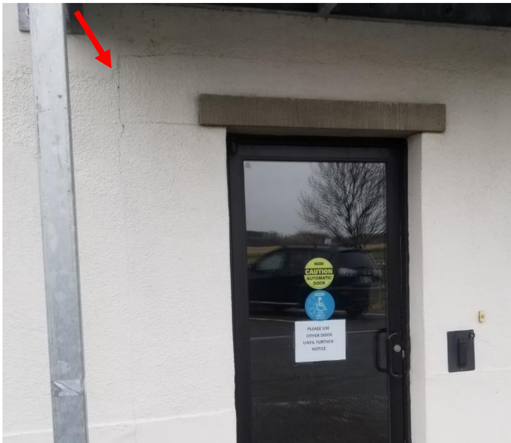
Photo 1. Exterior, west façade next to door, 1 metre fair condition texture coat on wall.
