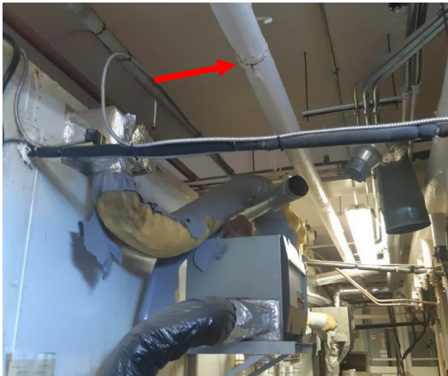
Photo 3. Basement, lab 15, along pipe above dehumidifier on north wall, <1 linear metre fair condition Aircell.
