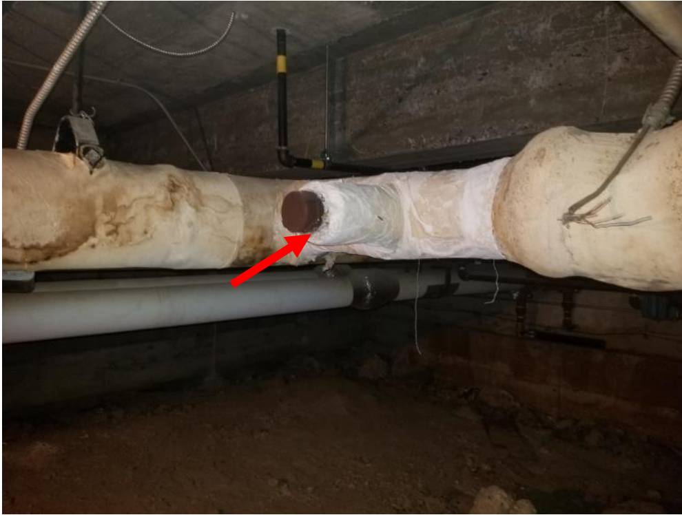
Photo 5. Basement, crawlspace, north-east corner, <1 linear metre poor condition fitting.
