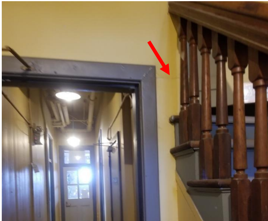
Photo 1. Ground floor, corridor/vestibule, <1 square metre fair condition drywall joint compound to the right of the door next to stairwell.
