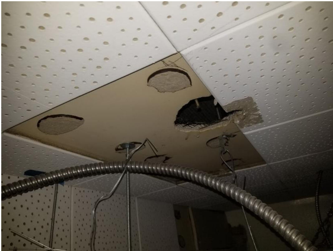
Photo 4. Second floor, room 201A, south side, <1 square metre (1 tile) in poor condition.
