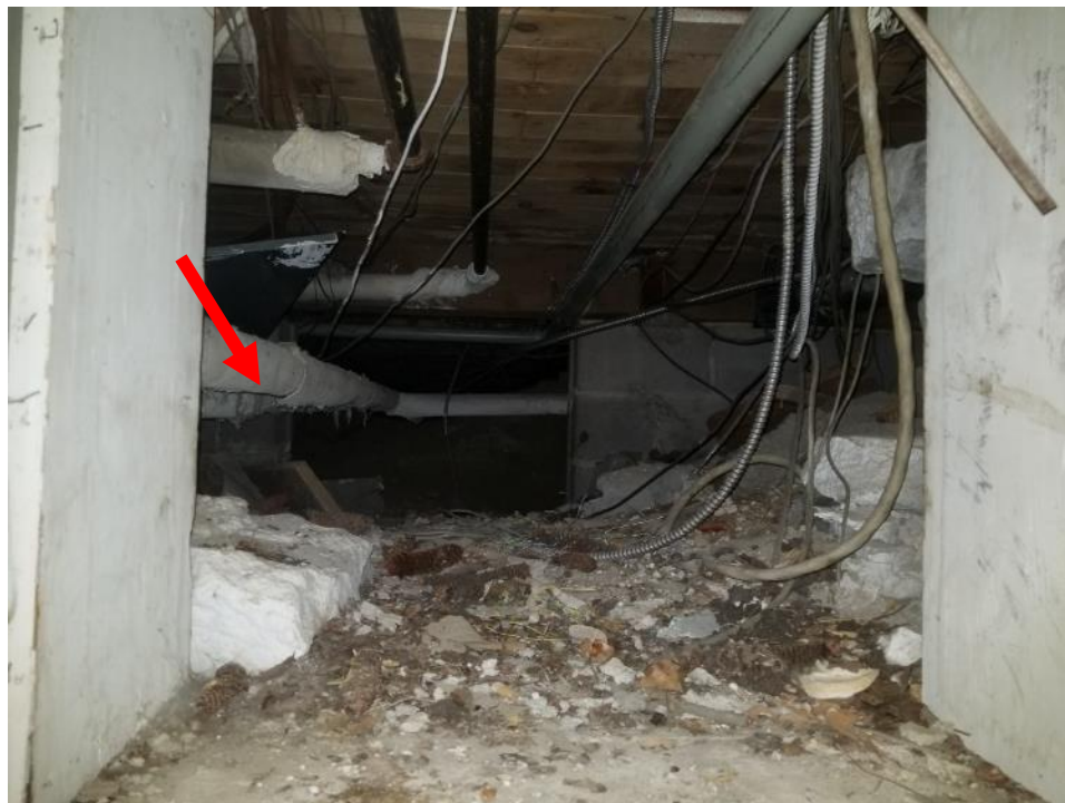
Photo 1. Basement, storage room between chimney and furnace rooms, behind panel on back wall in crawlspace, 20 linear metres poor condition Aircell.
