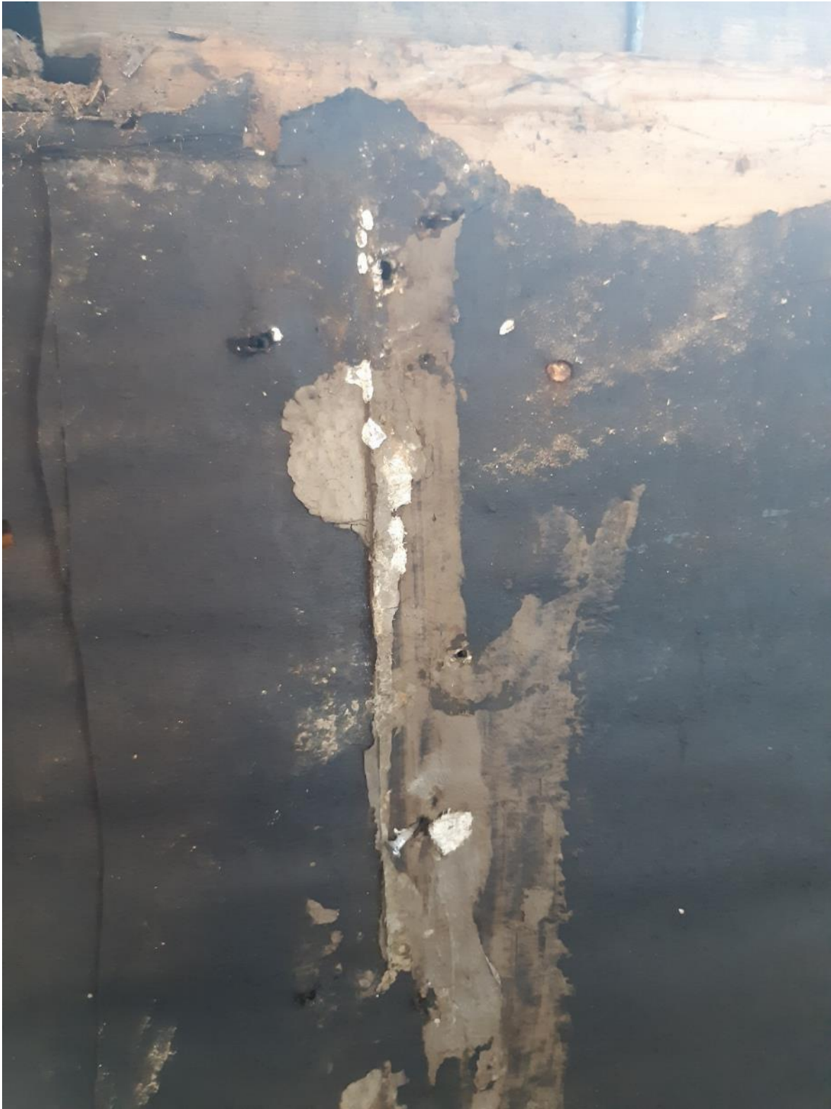
Photo 1. Ground floor, room adjacent entryway, 40 square metres of transite debris on walls.
