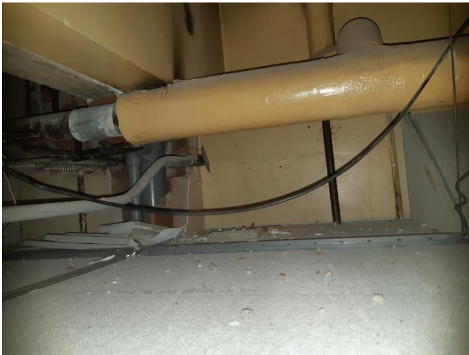
Photo 6. Basement, lab 101, above second window from east along south wall, 2 square metres debris on ceiling tile.
