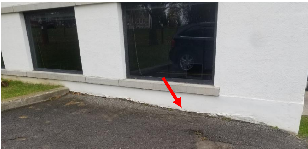
Photo 2. Exterior, north façade, 6 linear metres poor condition texture coat on wall.
