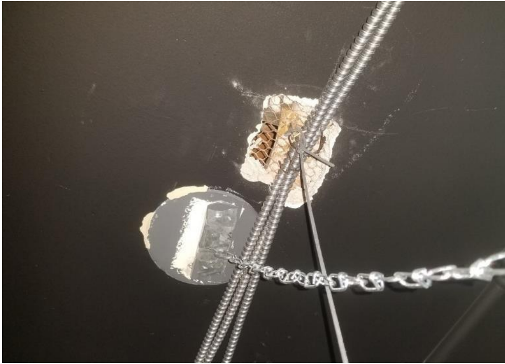
Photo 1. Basement, B-4, <1 square metre poor condition ceiling plaster at hangers throughout.
