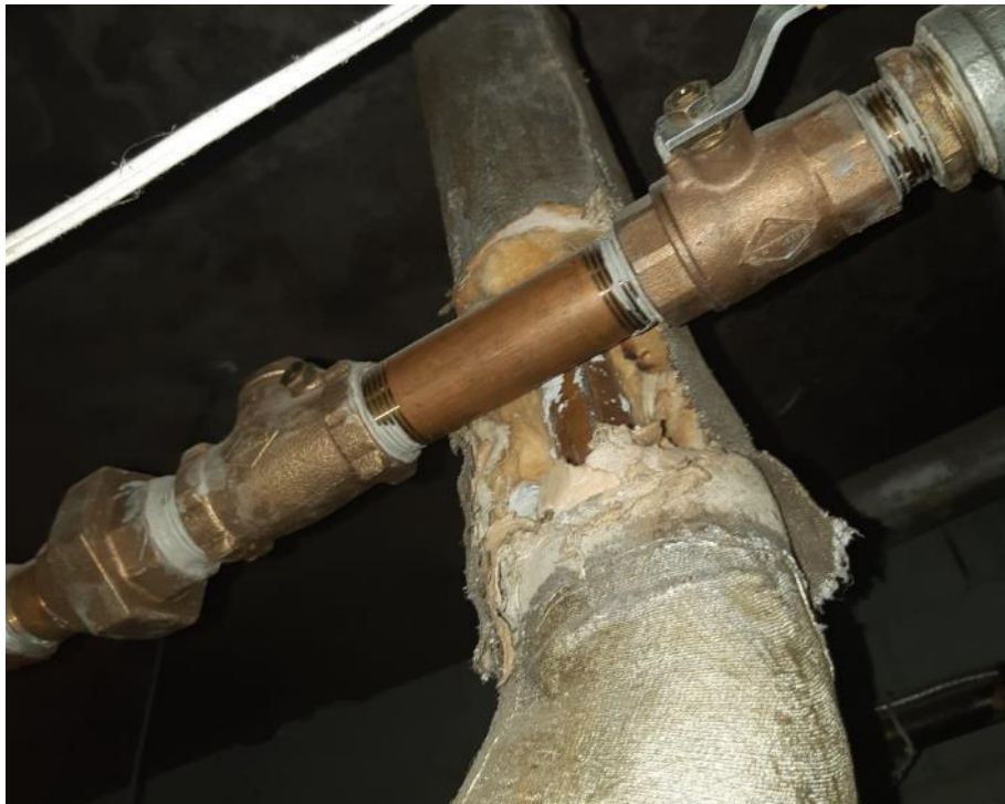
Photo 2. Basement, hallway to elevator, 1 poor condition fitting.
