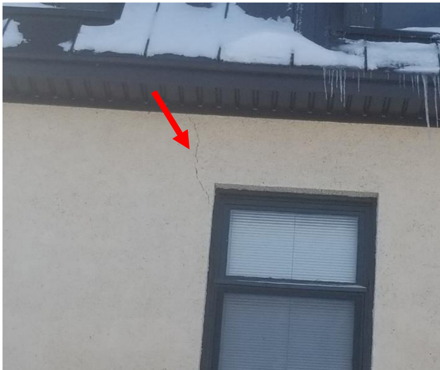
Photo 2. Exterior, north wall above fifth window from west, 1 linear metre fair condition stucco wall.
