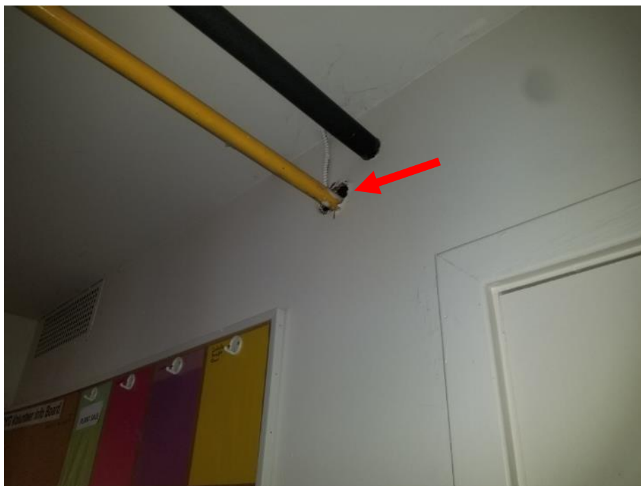
Photo 2. Ground floor, hall, east wall at yellow pipe penetration, <1 square metre poor condition drywall joint compound.
