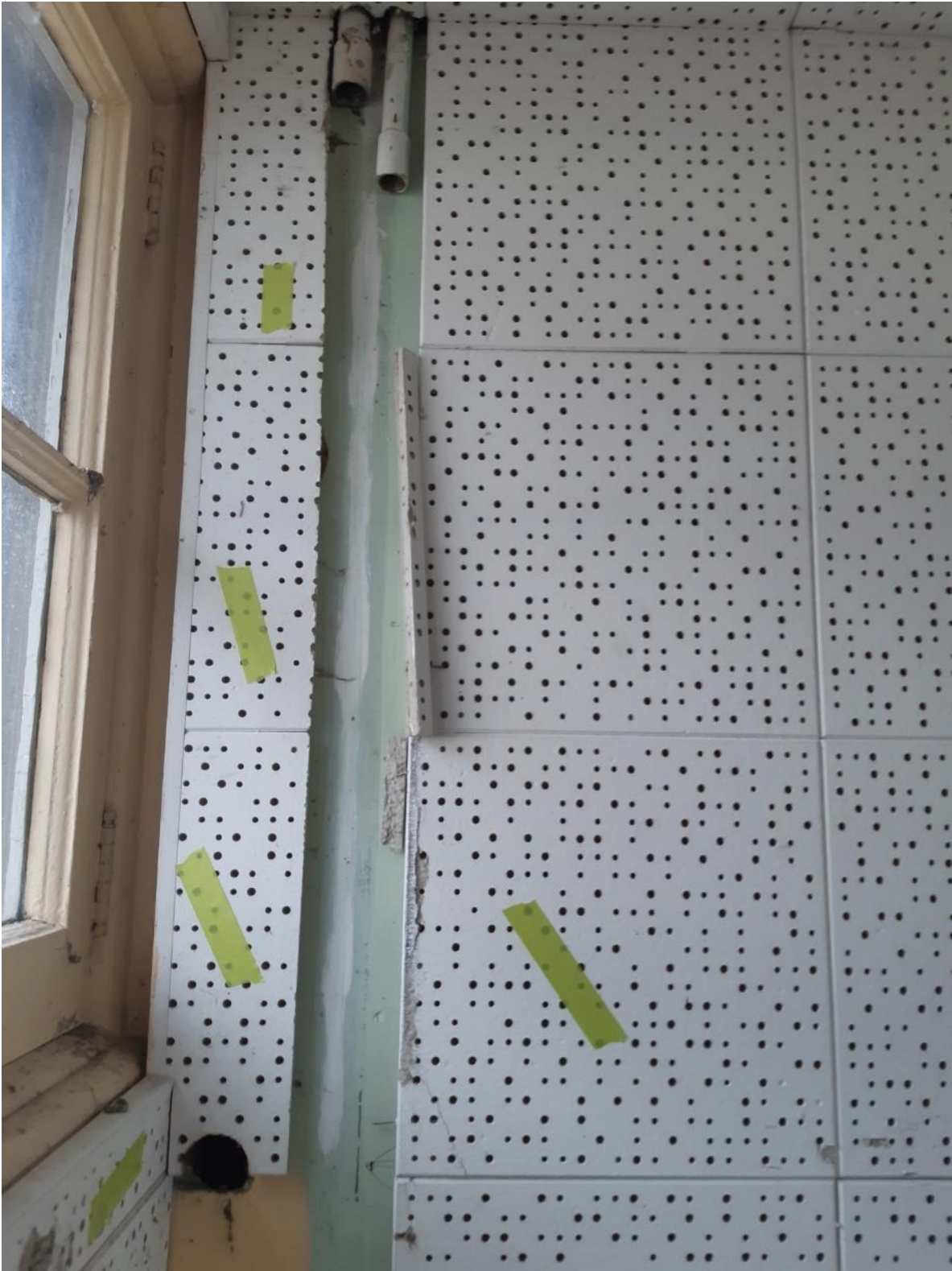
Photo 1. Ground floor, office space, poor condition 1'x1' grey acoustic tile on walls throughout.
