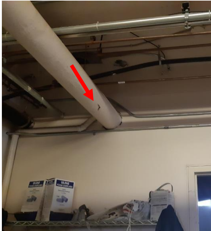
Photo 2. Basement, lab 12, on north wall to the west of room 14, <1 square metre fair condition Aircell.
