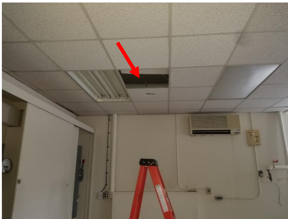
Photo 2. Ground floor, main area, south-west corner of room, <1 linear metre of poor condition Aircell.
