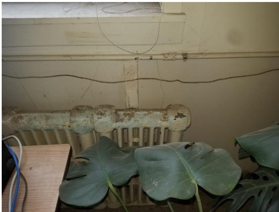
Photo 2. Ground floor, office 103, under north window, 1 square metre fair condition drywall joint compound wall.
