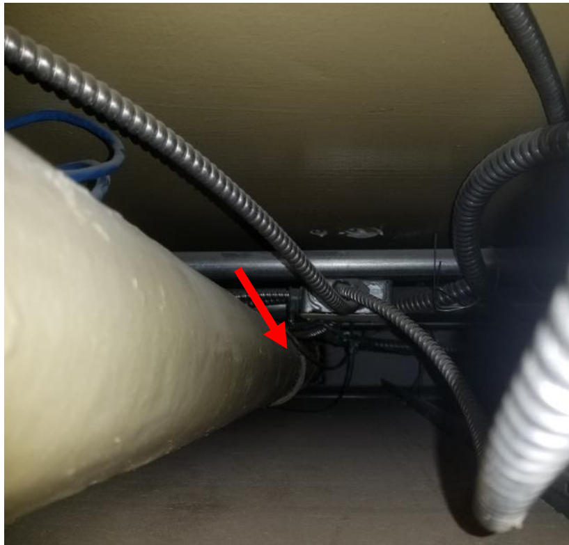
Photo 1. Basement, women's washroom, center of room, <1 linear metre poor condition thermal pipe insulation.
