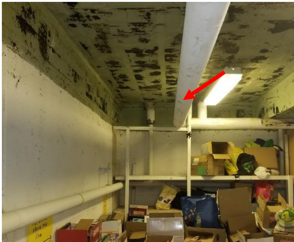
Photo 1. Basement, craft drying room, <1 linear metre fair condition Aircell on pipe running east to west in center of room.
