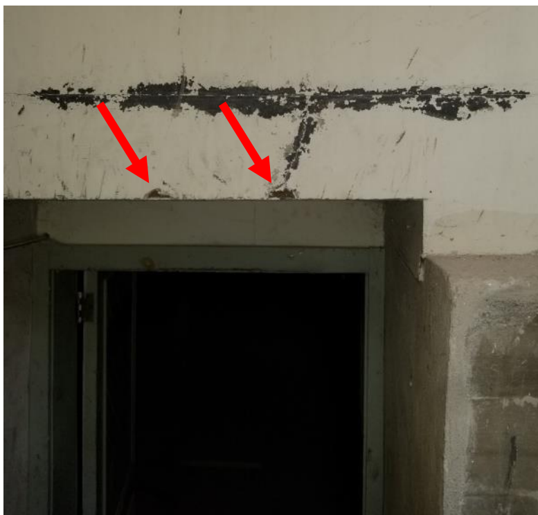
Photo 2. Basement to ground, stairwell, <1 square metre poor condition Transite wall.
