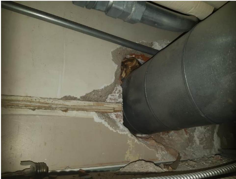
Photo 5. Basement, main hallway, 80 square metres poor condition wall plaster at pipe/duct wall penetrations.
