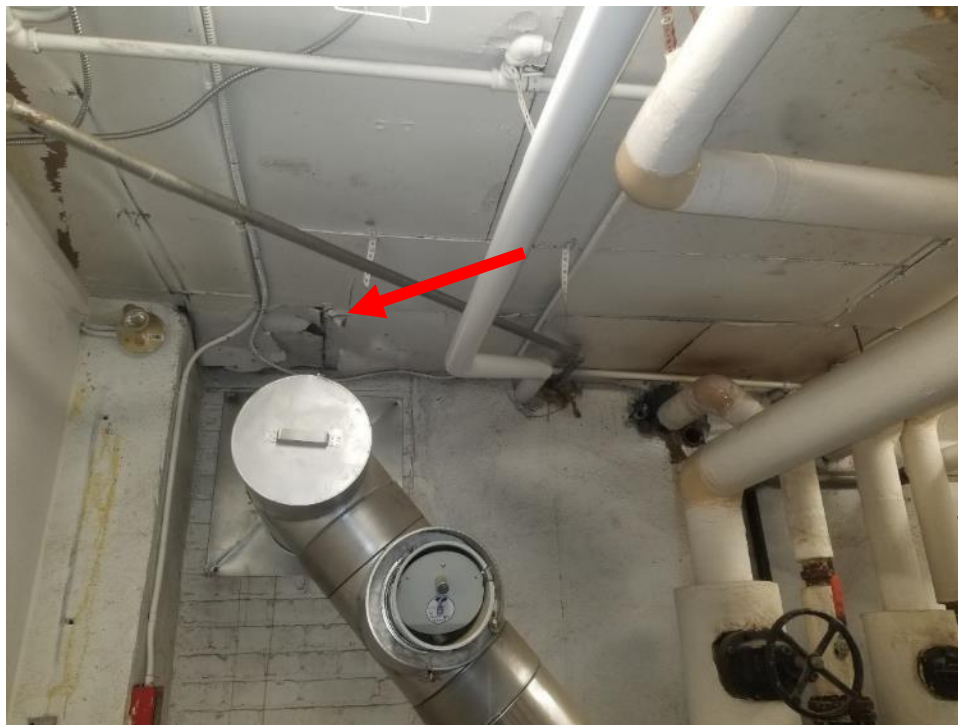
Photo 1. Basement, boiler room, west wall, 3 square metres poor condition Transite on ceiling.
