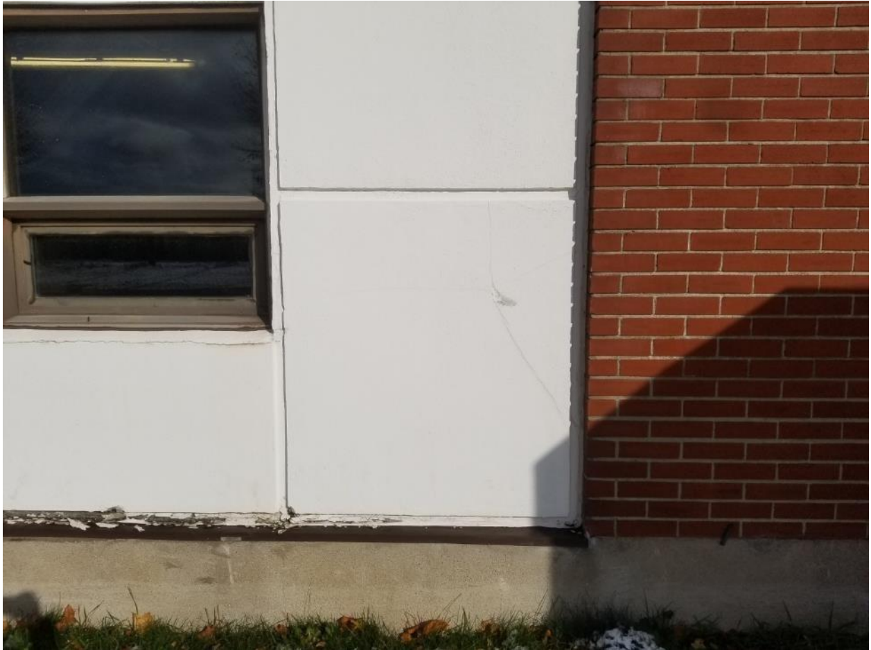
Photo 3. Exterior, south façade, east of first window, 1 square metre fair condition finish coat on wall.
