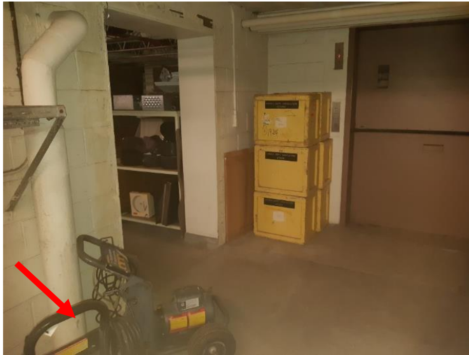
Photo 1. Second floor, mezzanine, north of freight elevator on east wall, <1 linear metre poor condition pipe insulation.
