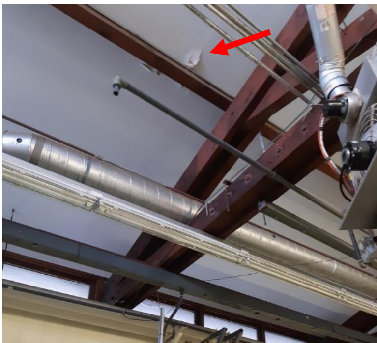
Photo 2. Ground floor, room 1, above growth unit #17, 1 square metre poor condition drywall joint compound.
