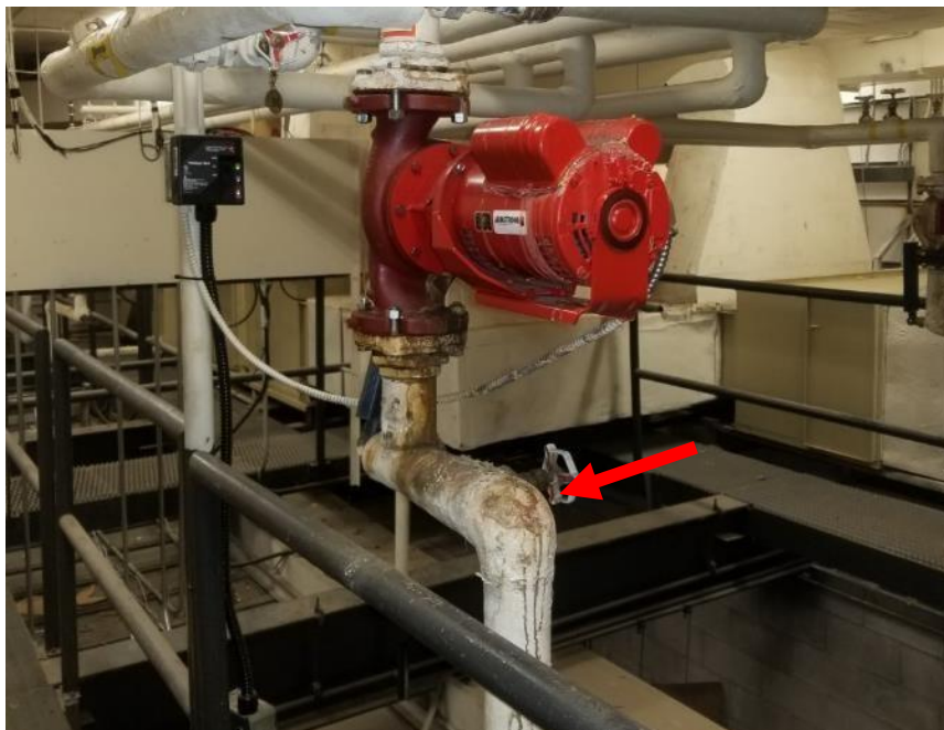
Photo 1. Mezzanine above boiler room, under red Armstrong machine, north-east side of room, 1 poor condition fitting.
