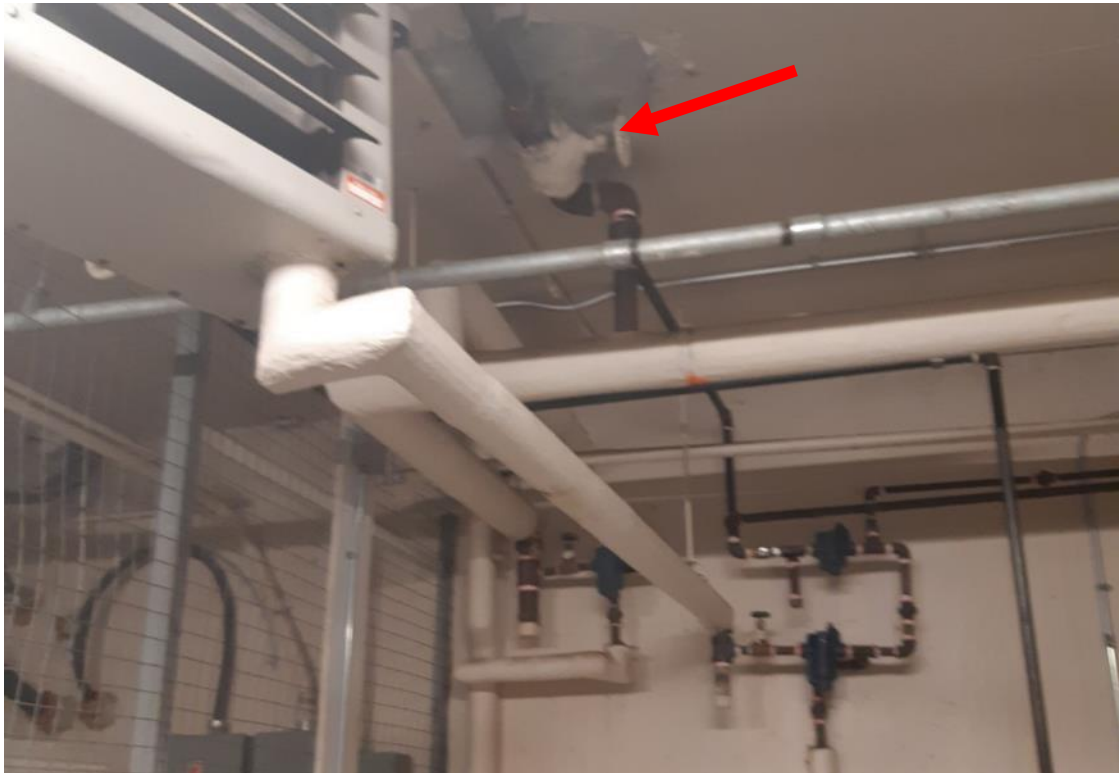
Photo 7. Basement, lab 15, north-west corner, 1 poor condition fitting.
