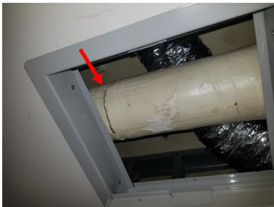
Photo 2. Basement, men's washroom, in ceiling hatch, <1 linear metre fair condition thermal pipe insulation.
