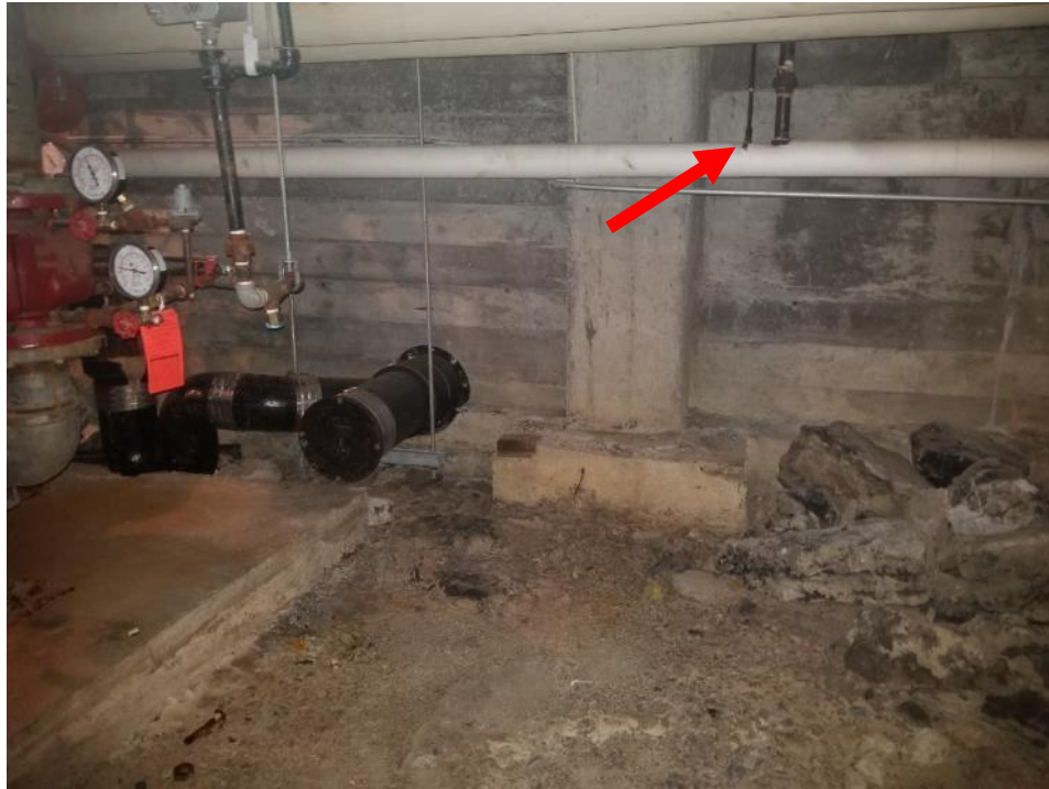
Photo 1. Basement, crawlspace, <1 square metre poor condition Aircell at hanger.
