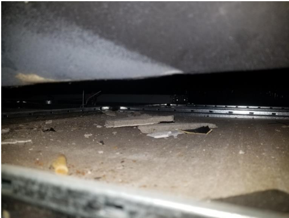
Photo 2. Basement, B-4, 200 square metres ceiling plaster debris throughout.
