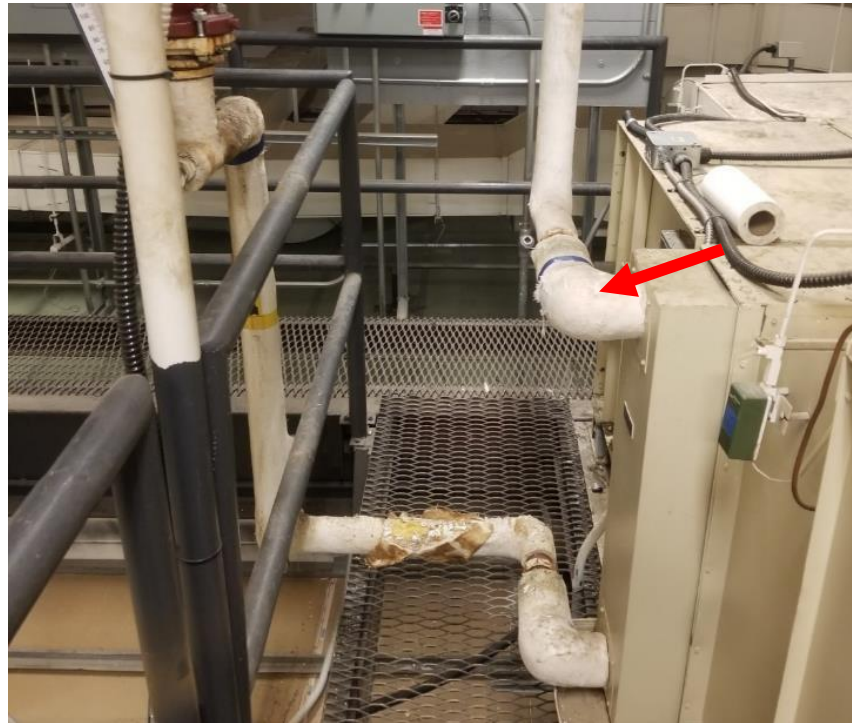
Photo 3. Mezzanine above boiler room, on AHU #3, north-east corner of room, 1 poor condition fitting.
