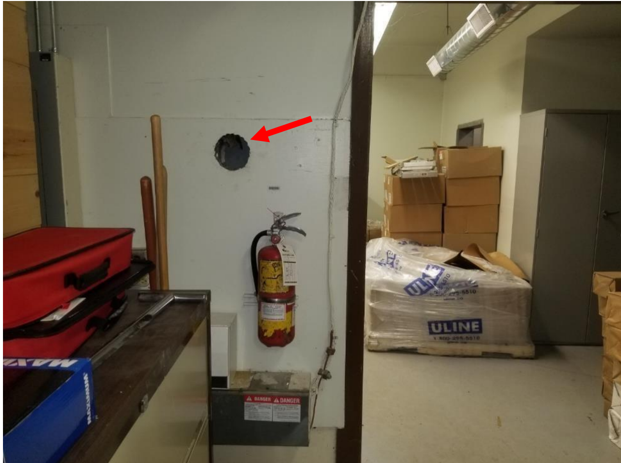
Photo 1. Ground floor, main room, north wall, <1 square metre fair condition Transite wall.
