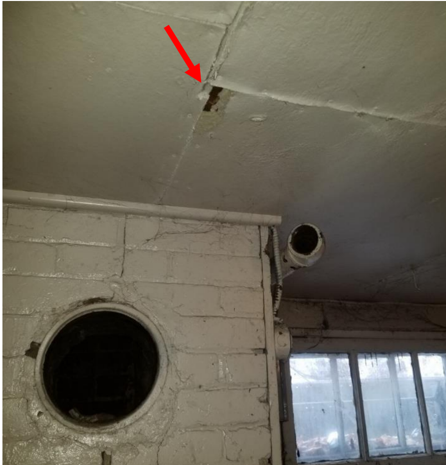
Photo 1. Basement, B-4, <1 square metre poor condition Transite on ceiling.
