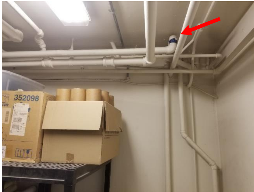
Photo 1. Basement, storage area, south-east corner, 1 poor condition fitting.
