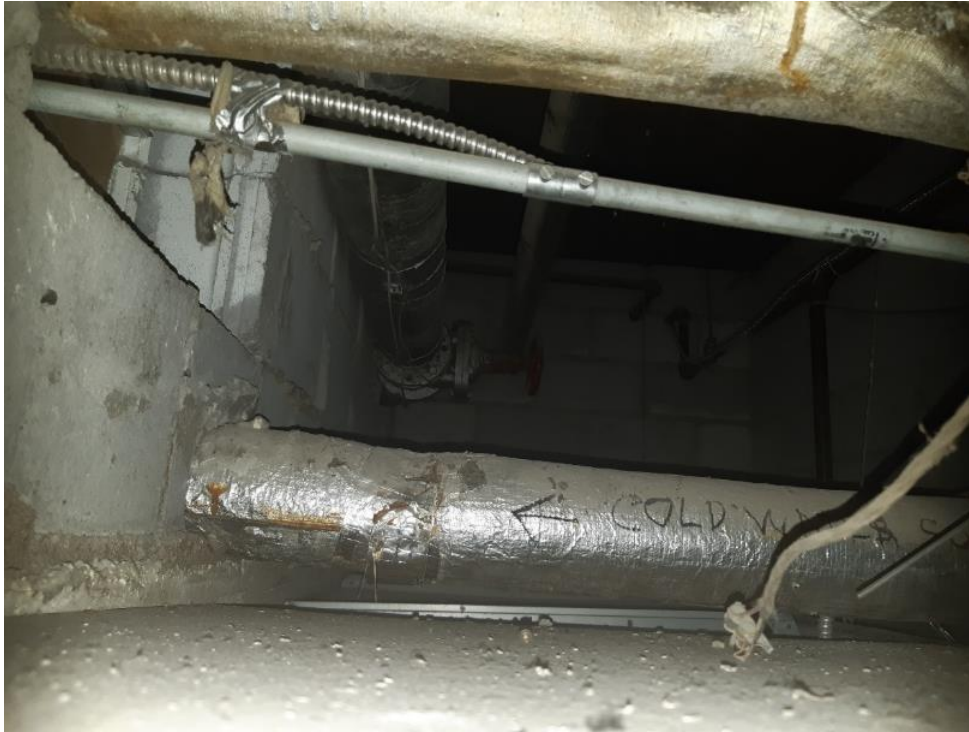
Photo 3. Basement, hallway to elevator, 4 square metres of Magblock debris on ceiling tiles.
