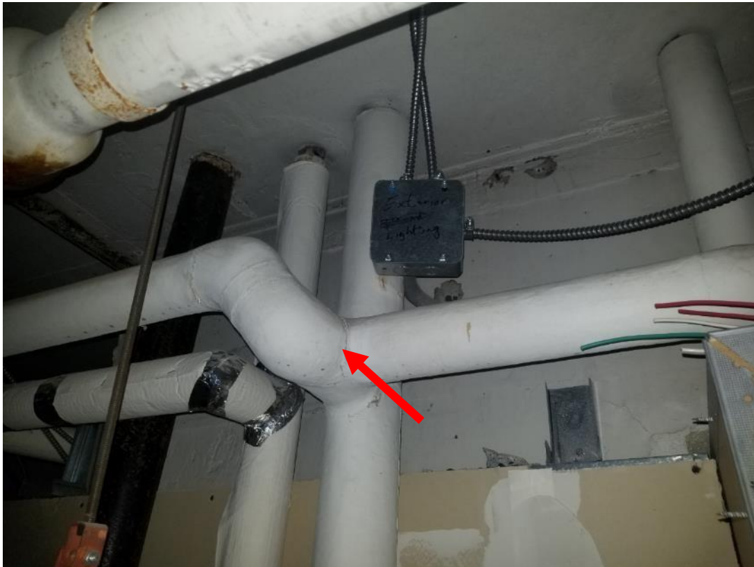
Photo 9. Basement, lab B-12, west of first window from west, 1 fair condition fitting.
