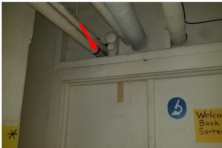
Photo 2. Basement, central, bottom of stairs next to door to B-1, <1 linear metre fair condition Aircell.
