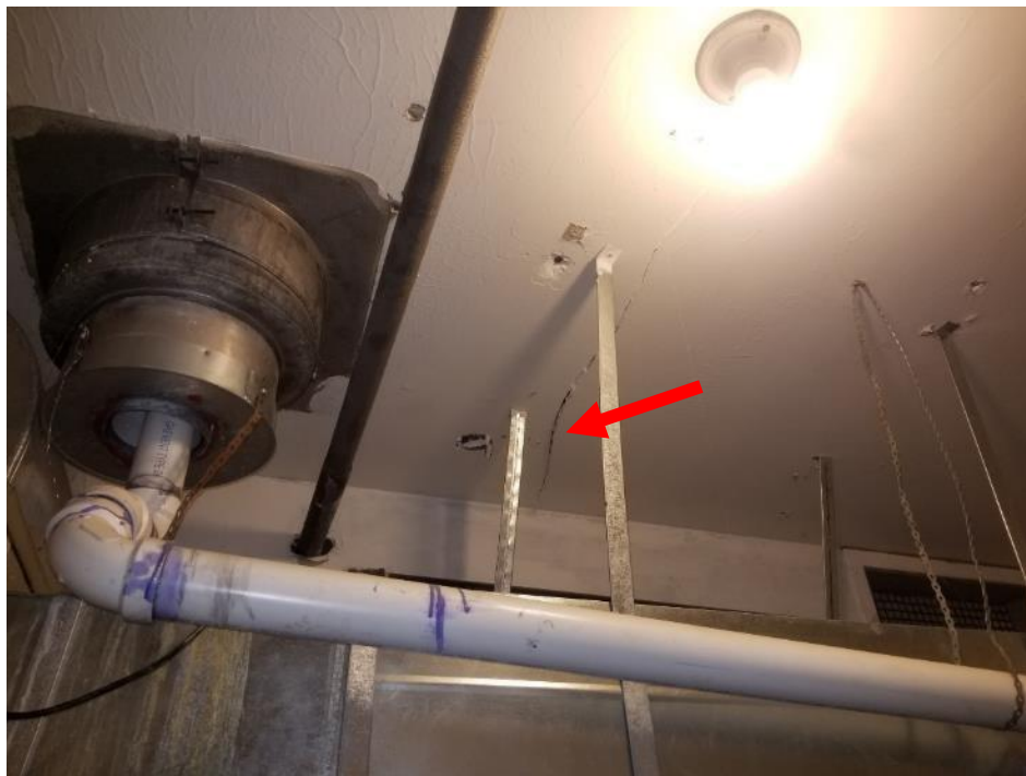
Photo 1. Ground floor, mechanical room ceiling, above duct, 1 square metre poor condition drywall joint compound.
