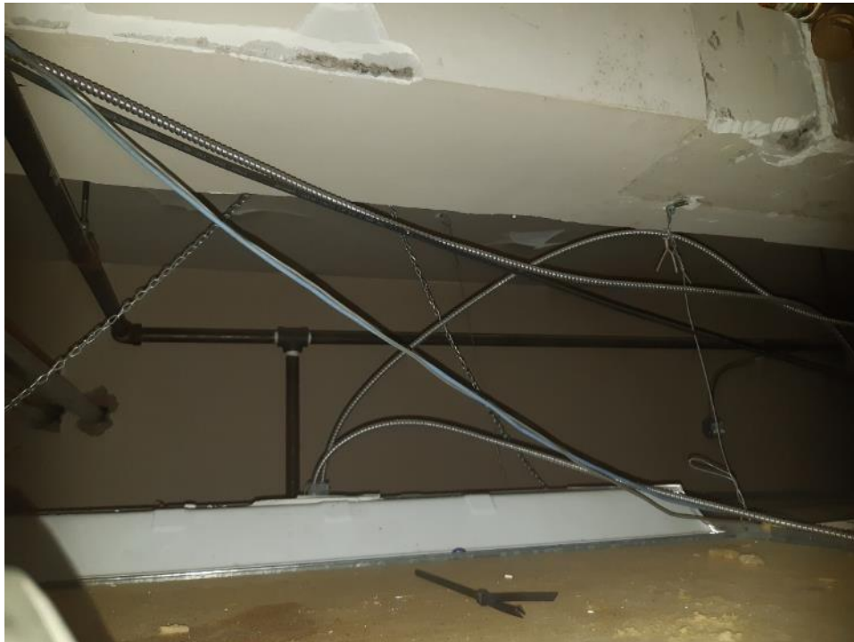
Photo 7. Basement, storage room 110, west of door, 2 square metres poor condition ceiling plaster and 4 square metres debris on ceiling tile.
