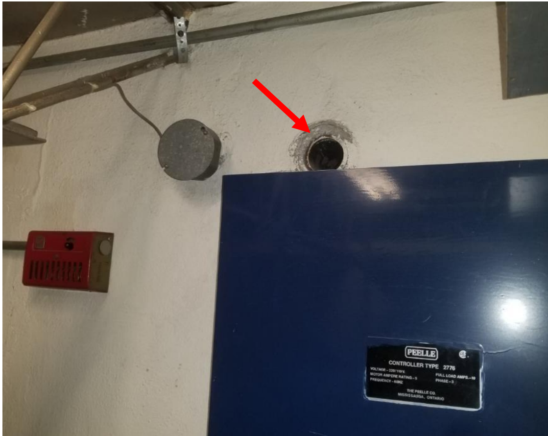
Photo 3. Second floor, west elevator control room, west wall, <1 square metre poor condition remnant pipe insulation.
