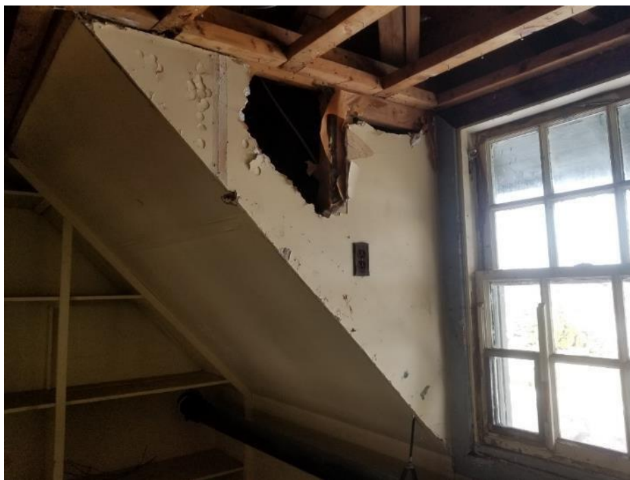
Photo 2. Third floor, storage room, 2 square metres poor condition drywall joint compound wall.
