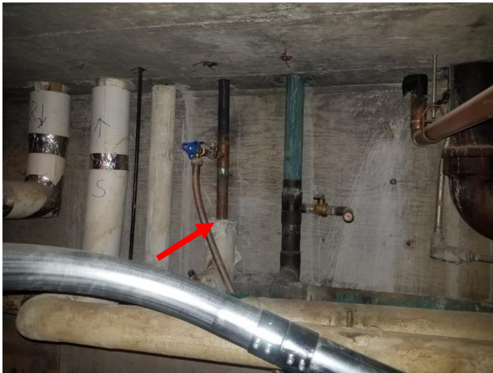
Photo 6. Basement, crawlspace, north-east corner, <1 linear metre poor condition Aircell.
