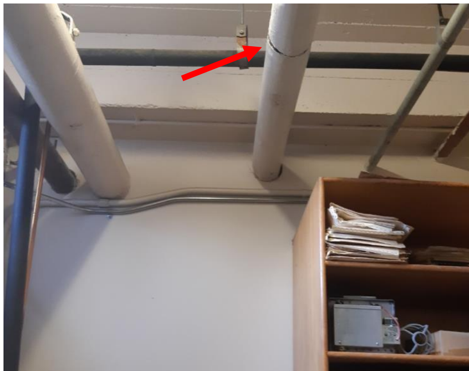
Photo 4. Basement, lab 15, along pipe above dehumidifier on north wall, <1 linear metre fair condition Aircell.
