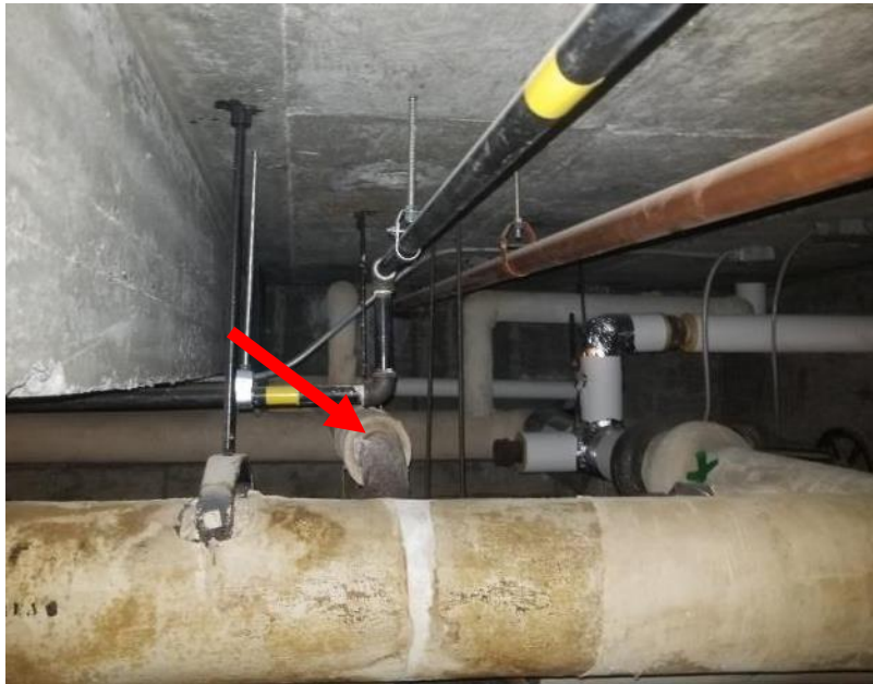
Photo 7. Basement, crawlspace, north-east corner, <1 square metre Aircell debris on cast iron pipe.
