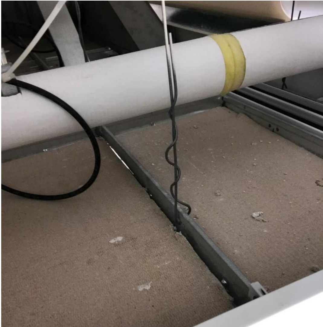
Photo 1. Ground floor, location 18 office, on south side of window, <1 square metre ceiling plaster debris on ceiling tiles.
