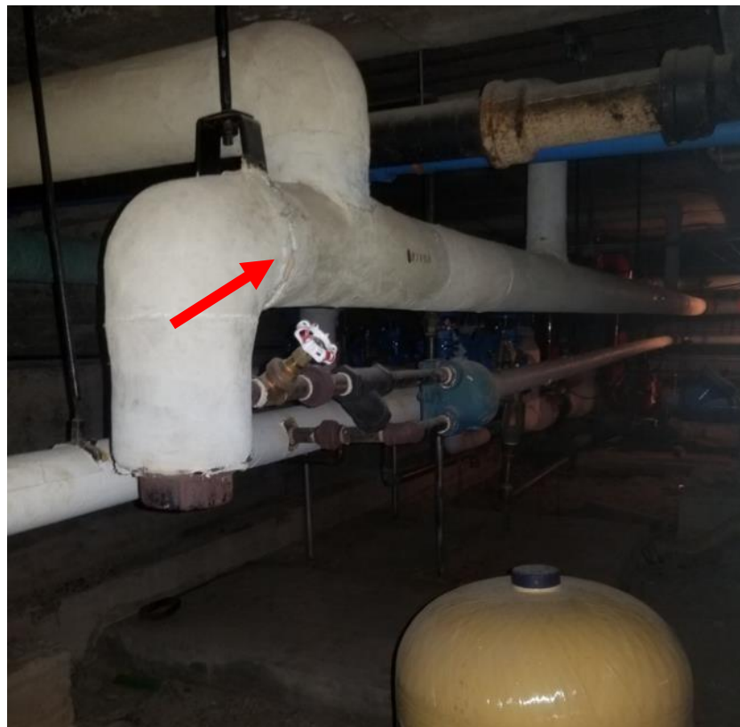
Photo 8. Basement, crawlspace, along east wall above yellow water tank, 1 poor condition fitting.
