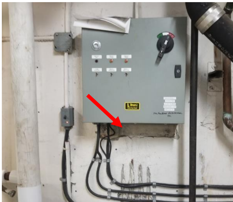
Photo 2. Basement, B-6, around emergency panel A on west wall, 1 square metre poor condition wall textured plaster.
