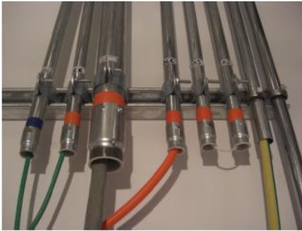
COLOR TAPED ELECTRICAL CONDUITS - BLUE FOR SECURITY
