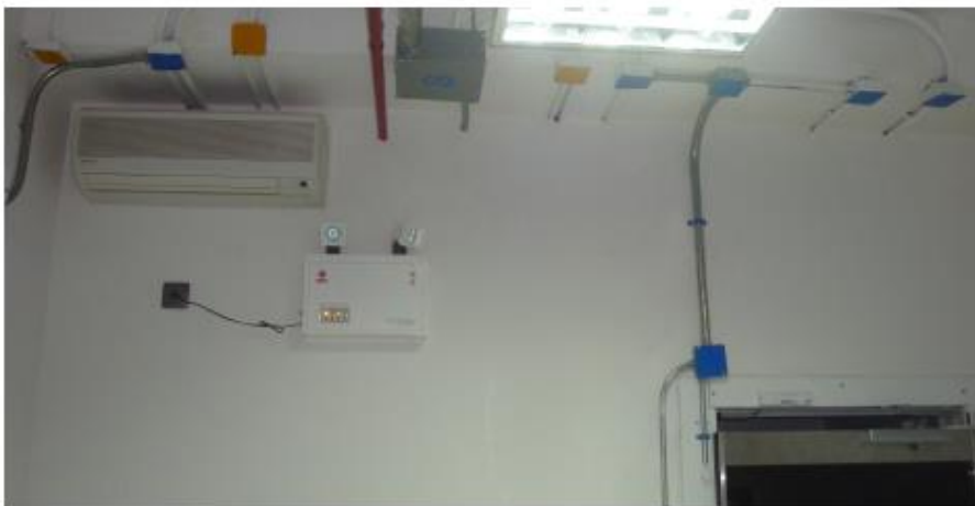
SPRAY PAINTED JUNCTION BOXES - BLUE FOR SECURITY
