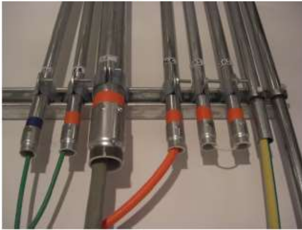
COLOR TAPED ELECTRICAL CONDUITS - BLUE FOR SECURITY
