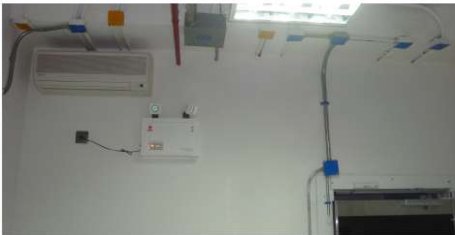
SPRAY PAINTED JUNCTION BOXES - BLUE FOR SECURITY
