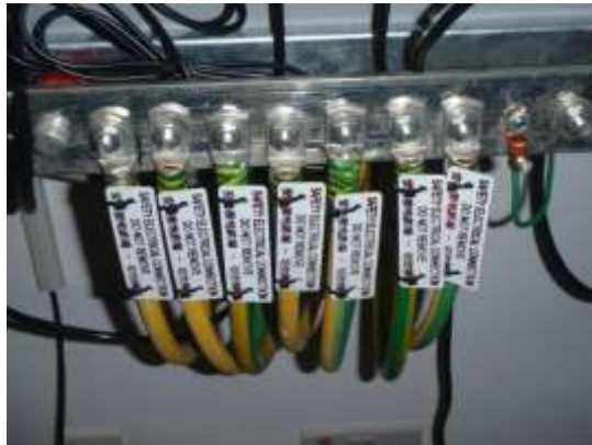
2/0 AWG main grounding conductor, terminal grounding bar and #10 AWG grounding conductor to equipment
