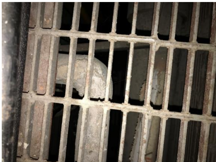
Photo 34: Pipe chase 2001-Stairwell, Poor Condition Pipe Fitting located below floor grate
