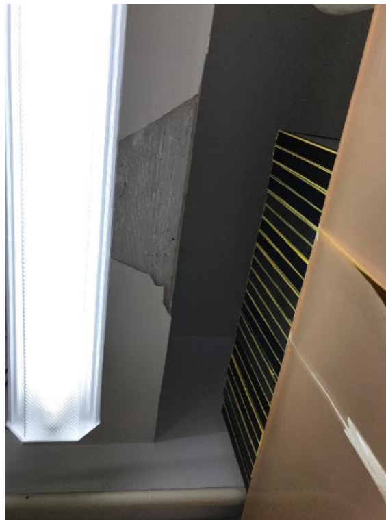
Photo 61: Room 3135, Poor Condition Ceiling Plaster on I-beam
