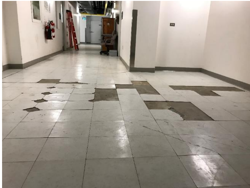
Photo 12: Corridor B85-B90 Poor Condition Vinyl Floor Tile
