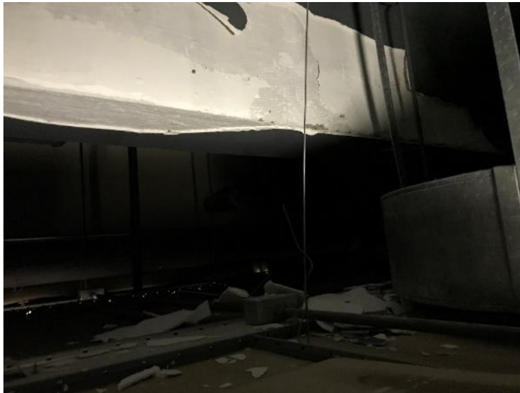
Photo 8: Room B71 and B71A Poor Condition Plaster and Debris located above and on Ceiling tiles
