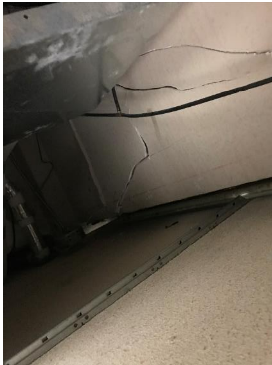
Photo 52: Room 2109, Poor Condition Wall and Ceiling Plaster located above ceiling tiles
