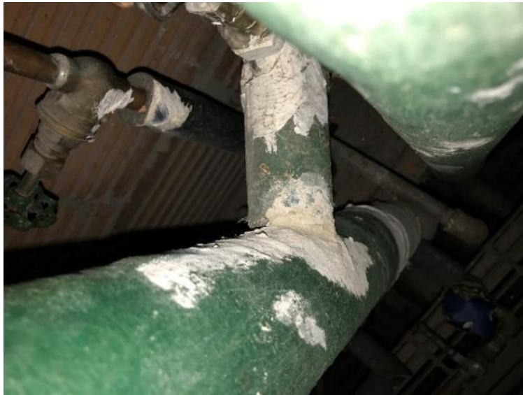
Photo 14: Pipe chase 1007-1009 Poor Condition Pipe Fitting and Aircell Pipe Insulation
