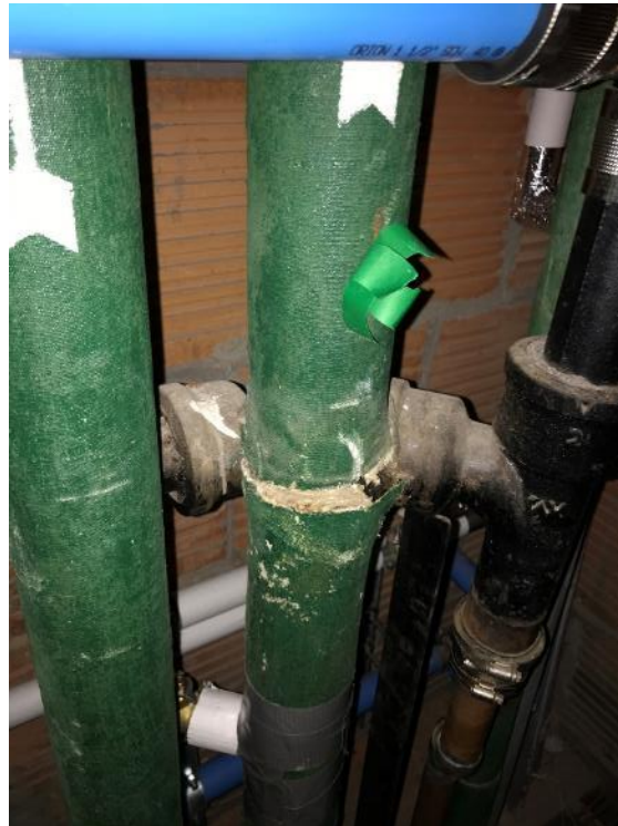
Photo 45: Pipe chase 2044-2046, Poor Condition Aircell Pipe Insulation
