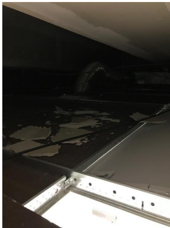
Photo 55: Room 2130, Poor Condition Ceiling Plaster and Plaster Debris located on and above ceiling tiles
