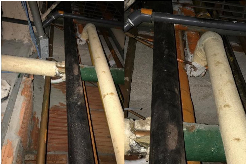
Photo 43 & 44: Pipe chase 2043-2045, Poor Condition Pipe Fittings and Aircell Pipe Insulation
