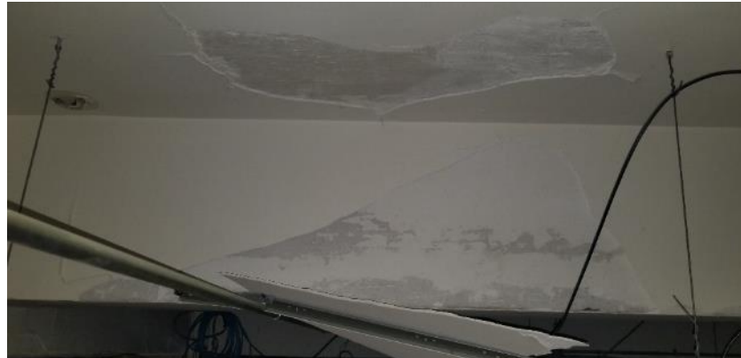
Photo 79: Room 4097, Poor Condition Ceiling Plaster and Ceiling Plaster Debris located above and on ceiling tiles
