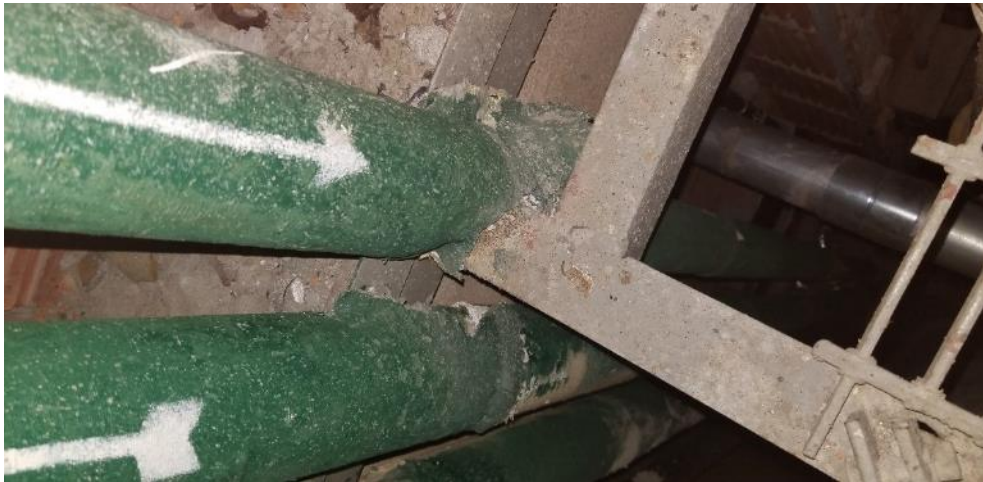
Photo 70: Pipe chase 4035-4037, Poor Condition Aircell Pipe Insulation and Debris located on floor grate
