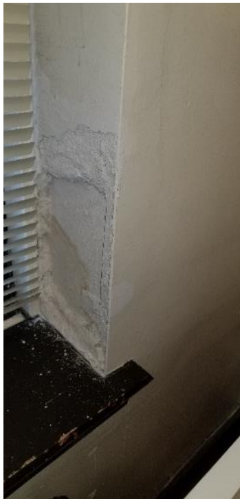
Photo 59: Room 3119, Poor Condition Wall Plaster and Debris located on Windowsill
