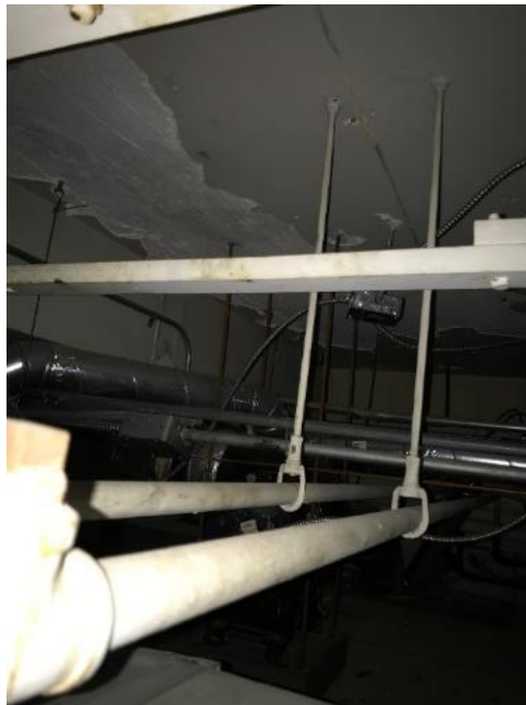
Photo 1: Room B-48, above ceiling tiles, Poor Condition Plaster and Debris
