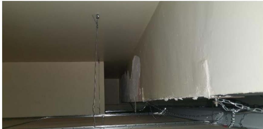
Photo 80: Room 4102, Poor Condition Ceiling Plaster and Plaster Debris located above Ceiling Tiles
