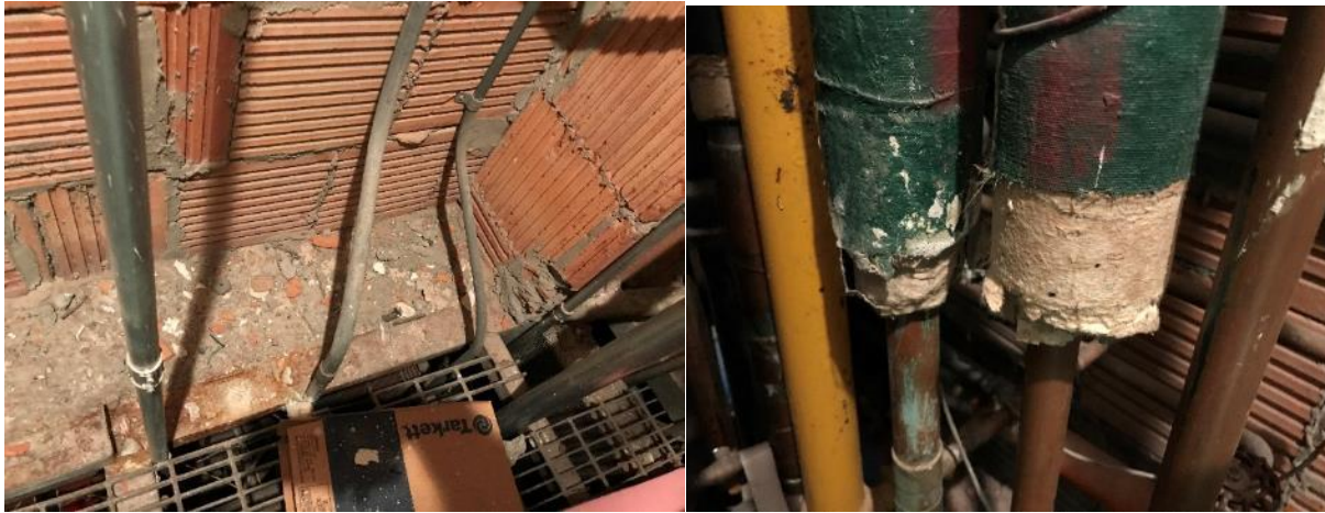
Photo 41 & 42: Pipe chase 2028-2030, Poor Condition Pipe Fittings with Poor Condition Aircell Pipe Insulation and Debris
