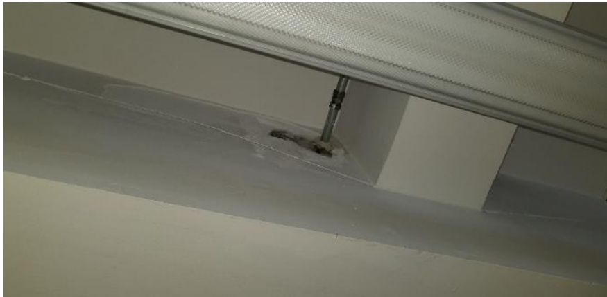
Photo 60: Room 3121-311A, Poor Condition Wall Plaster located on ceiling
