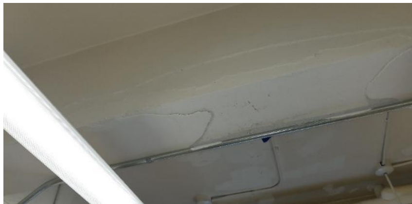
Photo 63: Room 3135E, Poor Condition Ceiling Plaster
