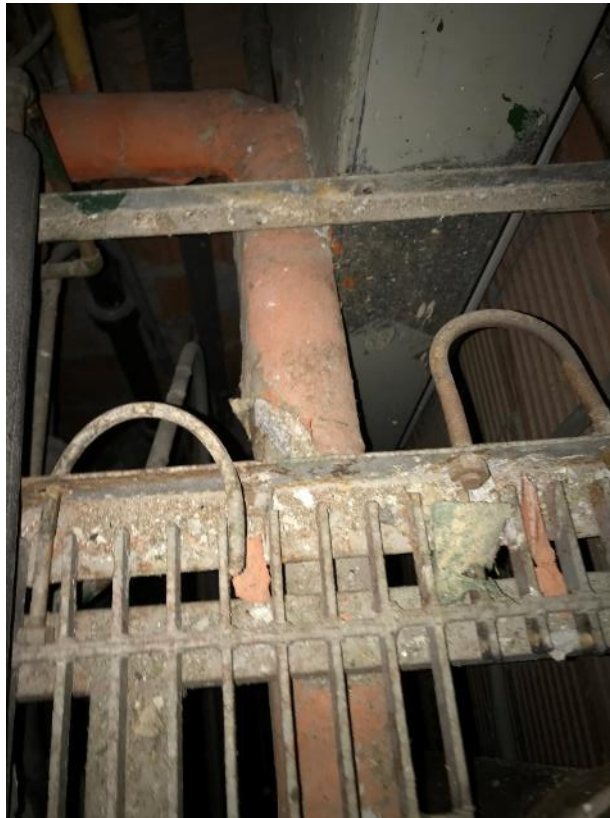
Photo 35: Pipe chase 2012-2014, Poor Condition Pipe Fitting and Aircell Pipe Insulation
