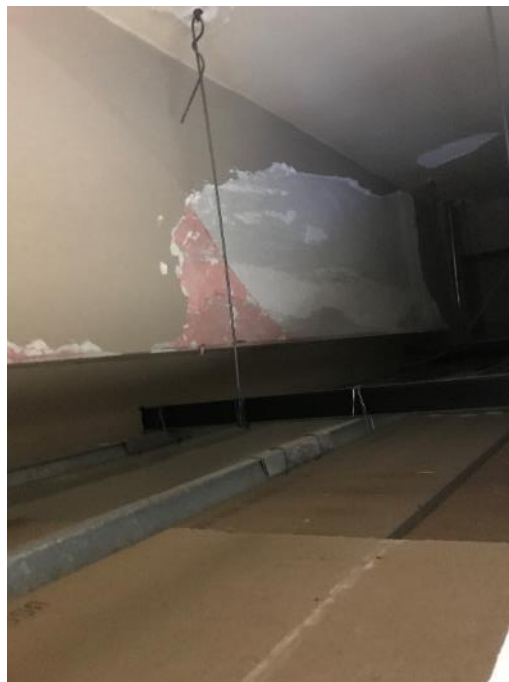
Photo 53: Room 2117, Poor Condition Ceiling Plaster and Plaster Debris located on and above ceiling tiles
