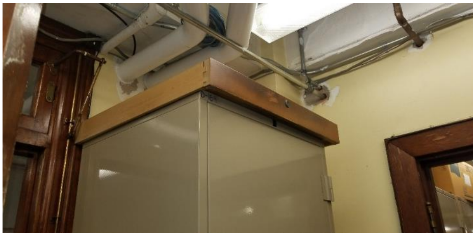
Photo 57: Common room of rooms 3109-3113, Poor Condition Poor Ceiling and Wall Plaster
