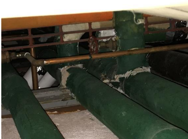
Photo 36: Pipe chase 2018-2020, Poor Condition Pipe Fittings
