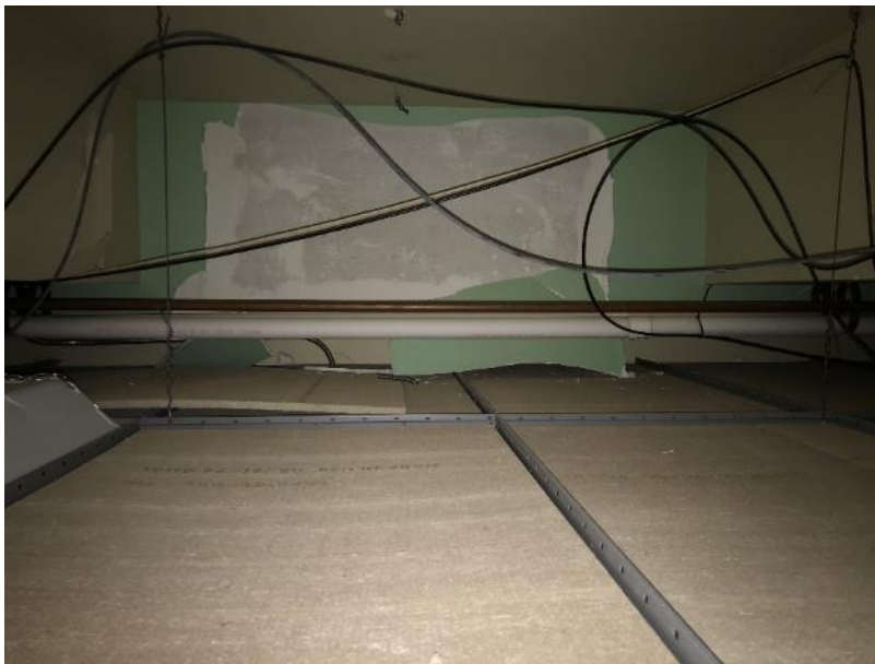
Photo 32: Room 1121A, Poor Condition Ceiling Plaster and Plaster Debris located on and above Ceiling Tiles
