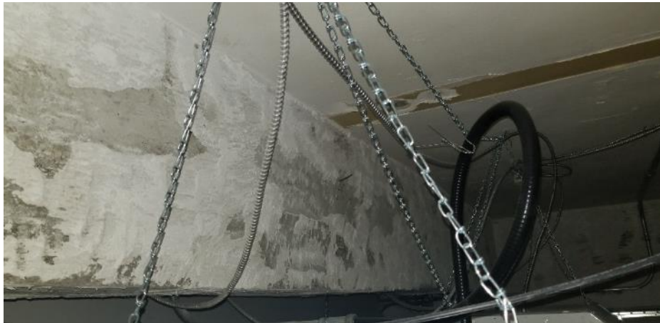
Photo 64: Room 3135G, Poor Condition Ceiling Plaster and Debris located above Ceiling Tiles
