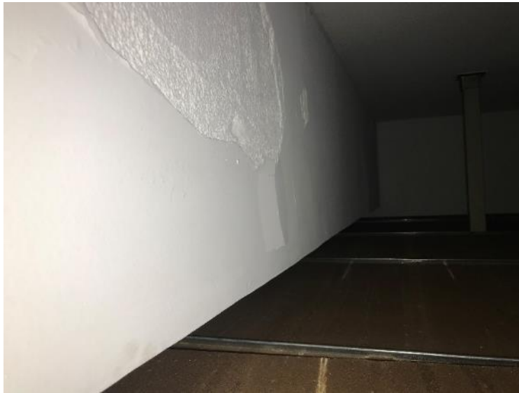
Photo 76: Room 4090, Poor Condition Ceiling Plaster and Debris located above and on ceiling tiles
