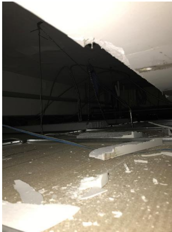
Photo 47: Room 2057, Poor Condition Ceiling Plaster and Plaster Debris located on and above Ceiling tiles
