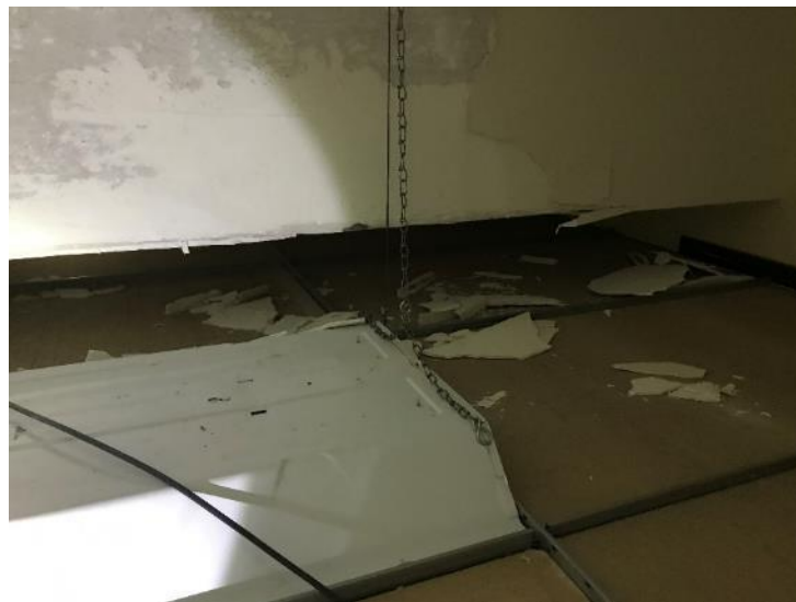
Photo 77: Room 4091, Poor Condition Ceiling Plaster and Plaster Debris located on and above ceiling tiles and on light fixtures
