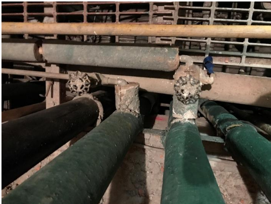
Photo 15: Pipe chase 1020-1022 Poor Condition Pipe Fittings and Debris
