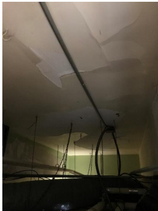
Photo 21: Room 1061A, Poor Condition Ceiling Plaster and Plaster Debris
