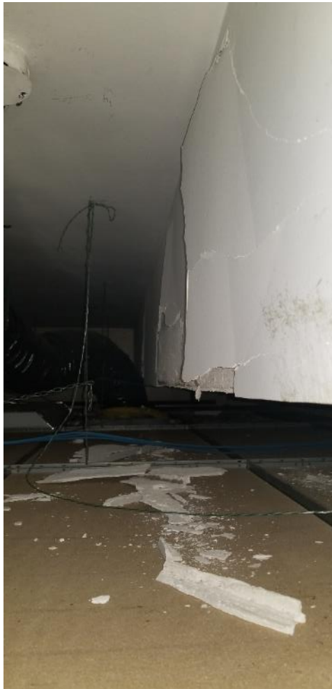
Photo 82: Room 4109, Poor Condition Ceiling Plaster and Plaster Debris located on and above ceiling tiles and light fixtures
