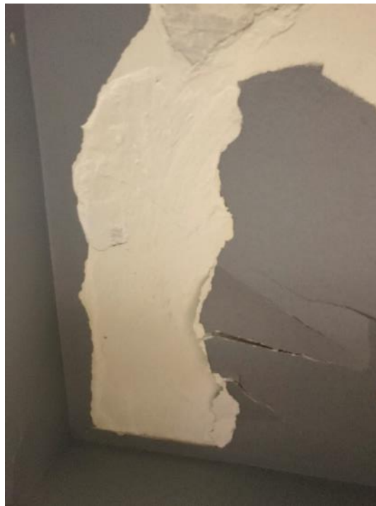
Photo 48: Room 2067, Poor Condition Ceiling Plaster and Plaster Debris located on and above Ceiling Tiles
