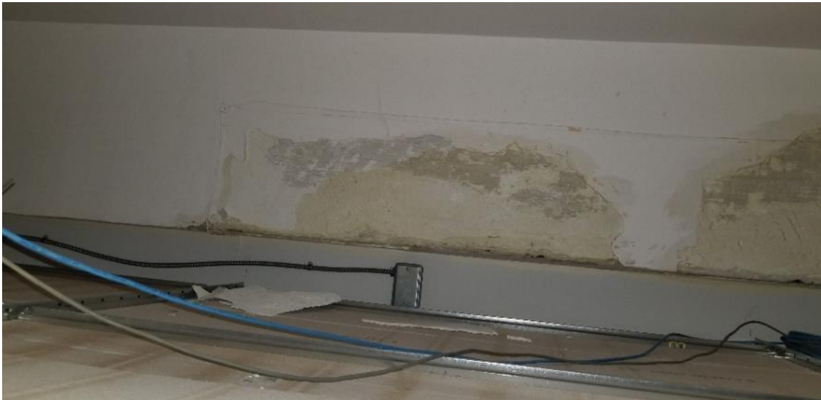
Photo 56: Room 3098, Poor Condition Ceiling Plaster and Plaster Debris located above ceiling tiles
