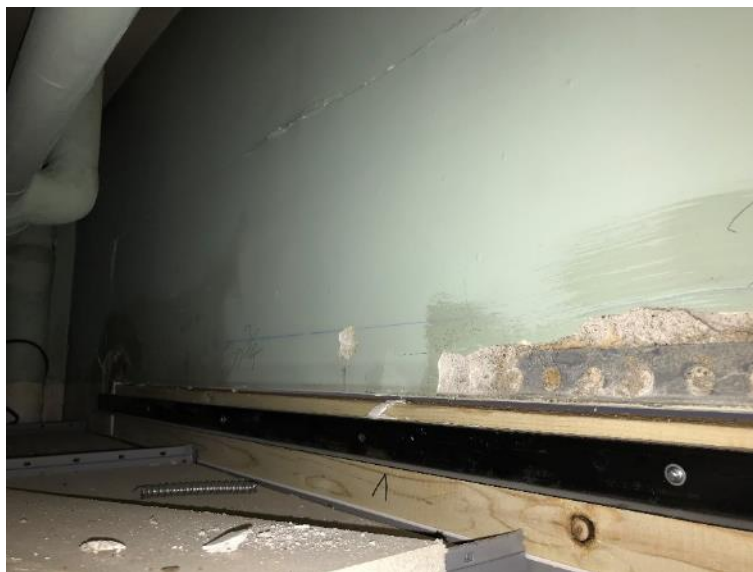
Photo 28: Room 1103A, Poor Condition Ceiling Plaster and Plaster Debris located on Ceiling Tiles
