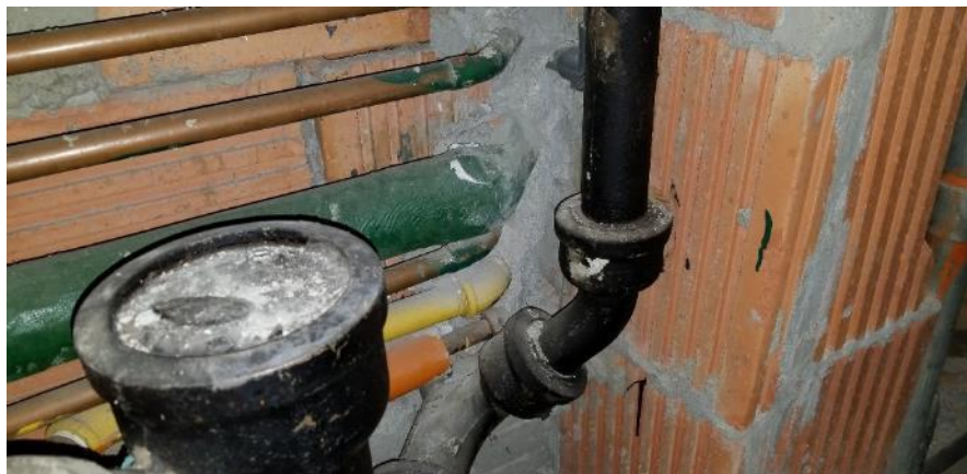
Photo 69: Pipe chase 4003-4005, Poor Condition Aircell Pipe Insulation and Debris
