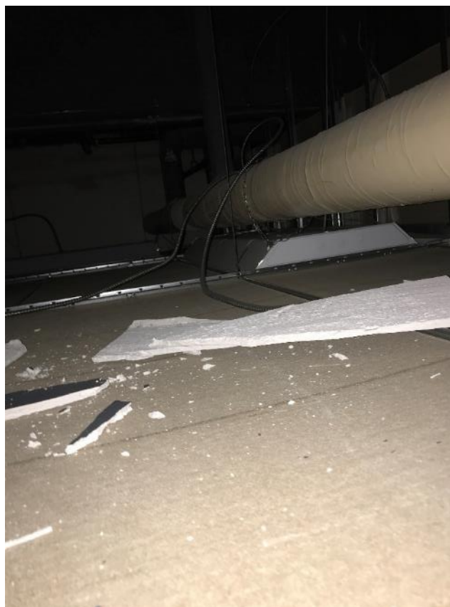
Photo 9: Room B84 Poor Condition Plaster and Debris located on Ceiling Tiles
