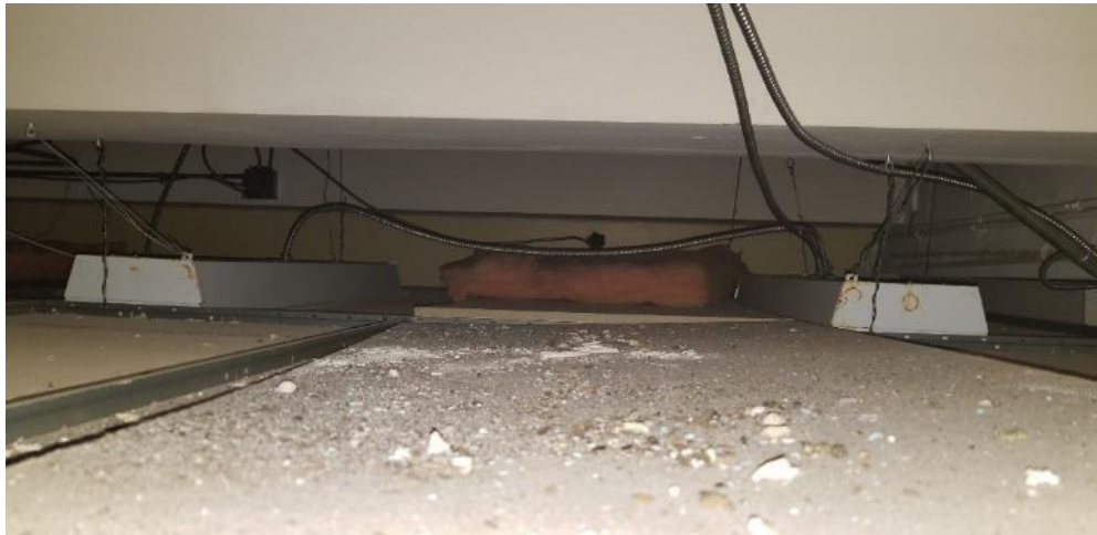
Photo 84: Room 4115, Poor Condition Ceiling Plaster and Plaster Debris located on and above ceiling tiles and light fixtures
