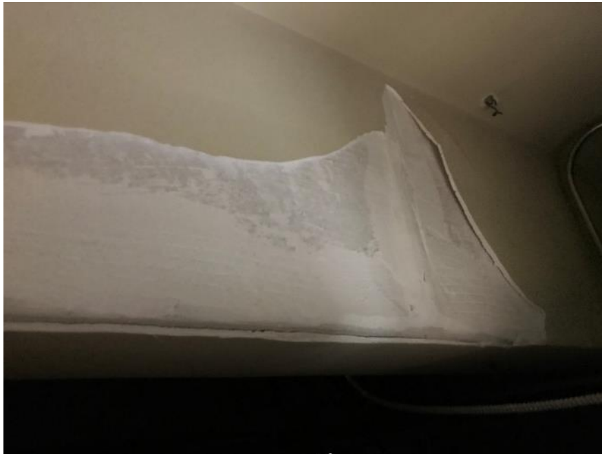
Photo 31: Room 1120, Poor Condition Ceiling Plaster located above Ceiling Plaster
