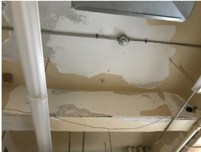
Photo 22: Room 1065A, Poor Condition Ceiling Plaster
