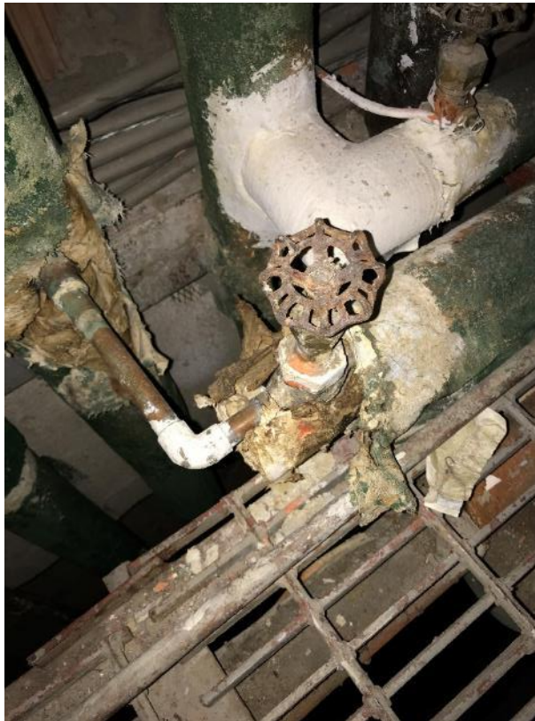
Photo 39: Pipe chase 2022-2024, Poor Condition Pipe Fittings and Aircell Pipe Insulation located at floor grate
