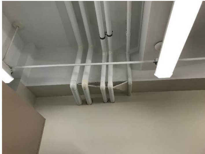
Photo 27: Room 1103, Poor Condition Ceiling Plaster and Plaster Debris
