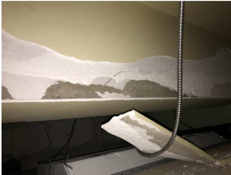
Photo 29: Room 1105, Poor Condition Ceiling Plaster and Plaster Debris located on Ceiling Tiles and Light fixtures.
