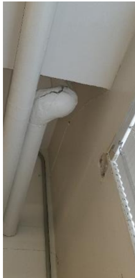
Photo 58: Room 3115-3117, Poor Condition Pipe Fitting and Ceiling Plaster
