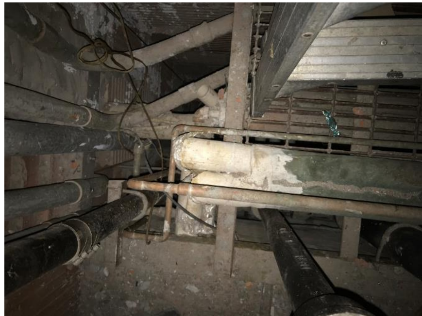
Photo 40: Pipe chase 2026-2028, Poor Condition Pipe Fitting and Aircell Pipe Insulation with Debris
