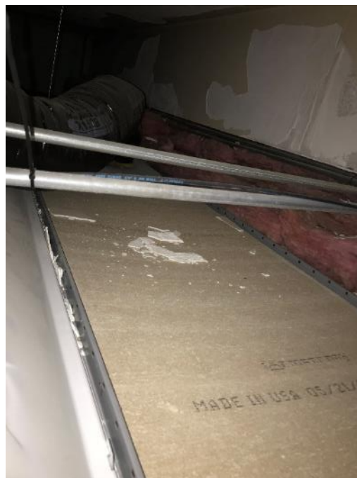
Photo 26: Room 1081, Poor Condition Ceiling Plaster and Plaster Debris Located on Ceiling Tiles
