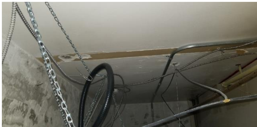
Photo 65: Room 3135H, Poor Condition Ceiling Plaster and Debris located above Ceiling Tiles
