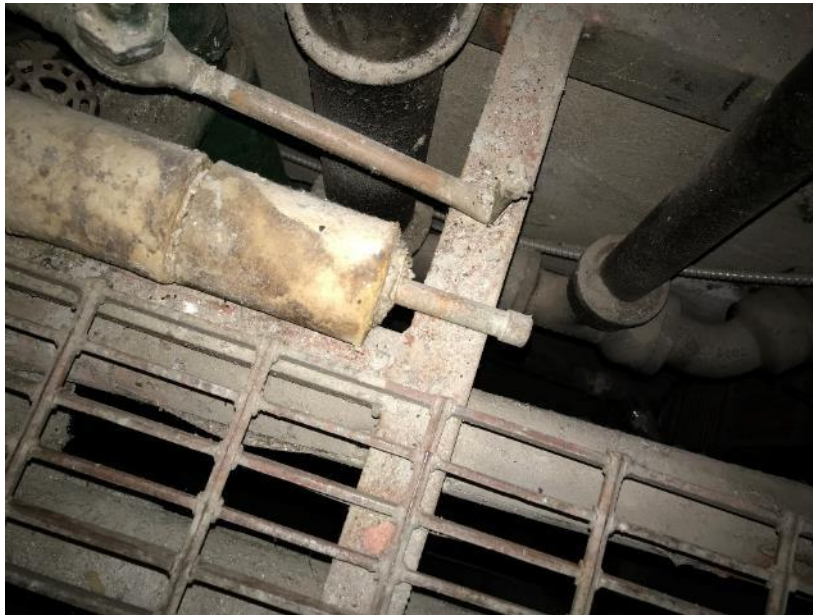
Photo 37: Pipe chase 2020-2022, Poor Condition Pipe Fitting located at floor grate
