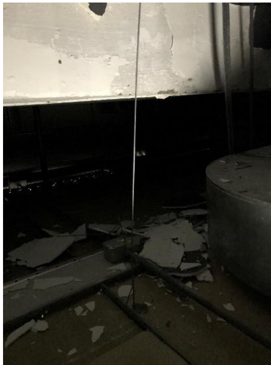
Photo 7: Room B71 and B71A Poor Condition Plaster and Debris located above and on Ceiling tiles
