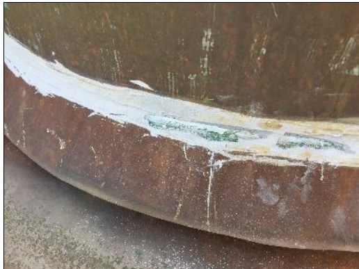
Non-PCB light grey caulking.
