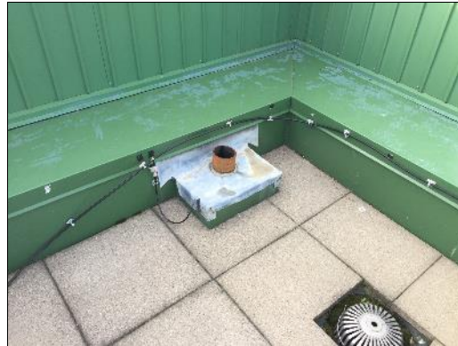
Lead-based green paint on the roof.
