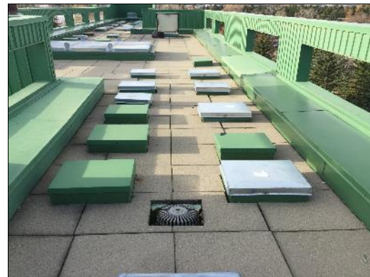
Presumed lead-containing roof drain.
