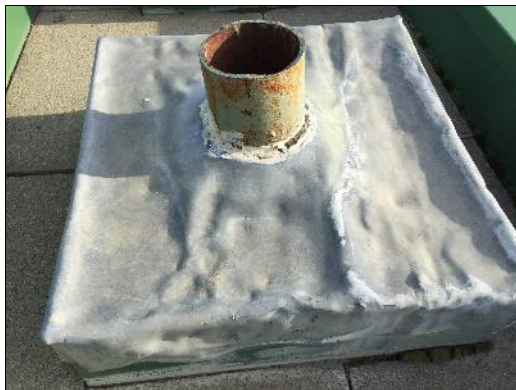
Example of lead sheeting found on the roof.
