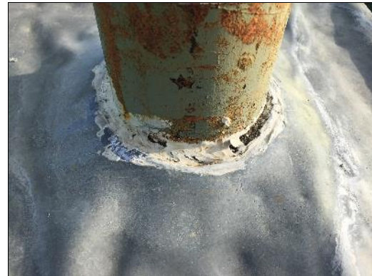
Non-PCB white caulking.
