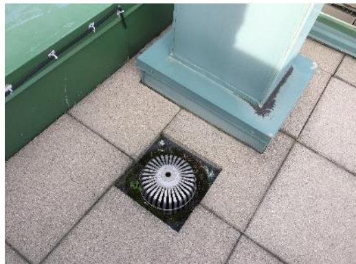
View of the concrete slabs on the roof and a roof drain.
