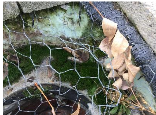
Close-up view of the roof drain shows non-asbestos Styrofoam insulation and plastic sheeting.
