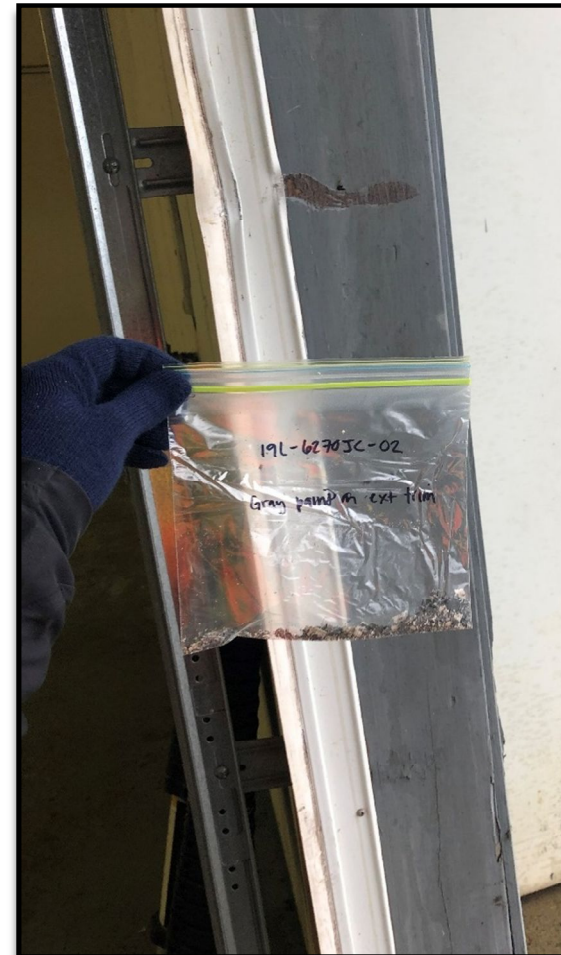
Grey paint sample 19L-6270JC-02 applied to the exterior wood trim with lead concentration: <0.0058 wt% (<58 ppm).
