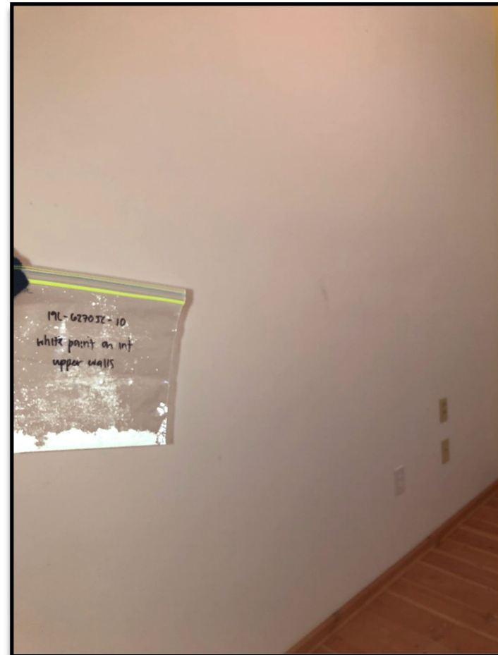
White paint sample 19L-6270JC-10 applied to the upper residence interior drywall walls with lead concentration: 0.0086\text{ wt\%} (86 ppm).
