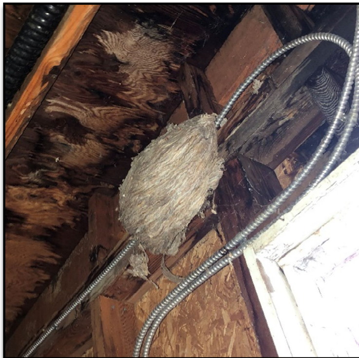
A wasp nest was observed on the interior wood framing above the doorway of the electrical room.
