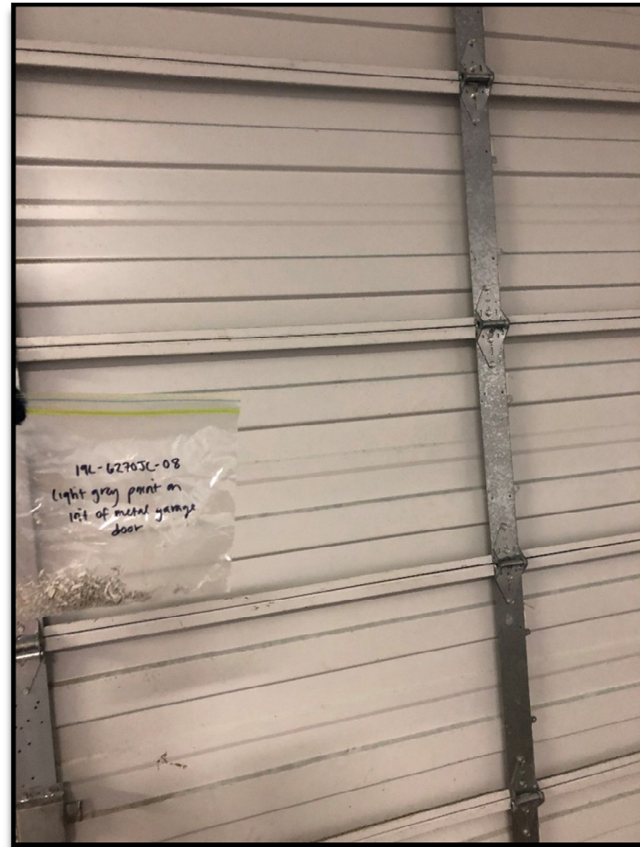
Light grey paint sample 19L-6270JC-08 applied to the interior of the roll-up metal door with lead concentration: <0.0084 wt% (<84 ppm).
