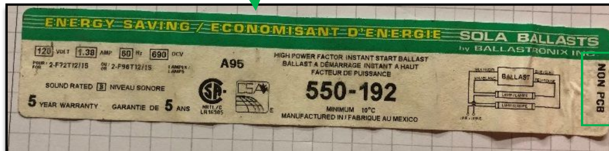
Fluorescent fixture lamp ballasts as inspected within the warehouse were found to be labeled “NON PCB”.
