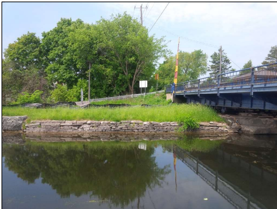
Photo 6: Overgrown grass and scrub vegetation presently downstream (south) on western bank of Warsaw Bridge. Photo taken south of bridge on eastern bank, facing west. Photo taken by Environmental Officer, Sarah Bunting May 30th, 2018.
