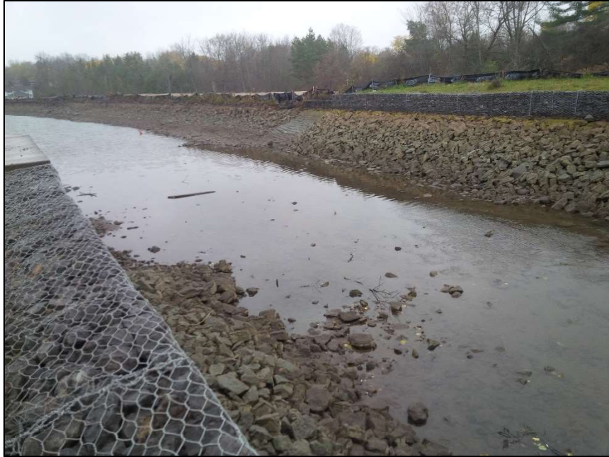
Photo 15: Typical winter/non-navigation season's water levels of Warsaw Bridge. Photo taken downstream (south) of Warsaw Bridge, facing south. Photo taken by Environmental Officer, Sarah Bunting November 5th, 2018.
