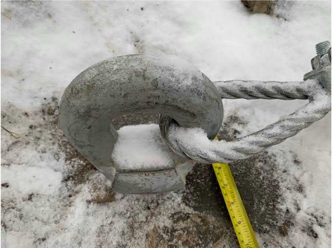
Photograph 9: Close view of a cable loop connection to an anchor eye nut.
