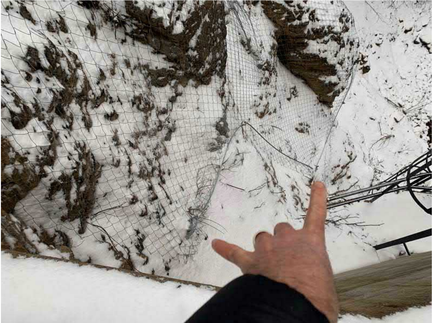
Photograph 8: View down from top of valve platform at bottom of mesh. Fingers point to locations of rock anchors with anchor plates and nuts that are used to pin the bottom of the mesh to the slope.
