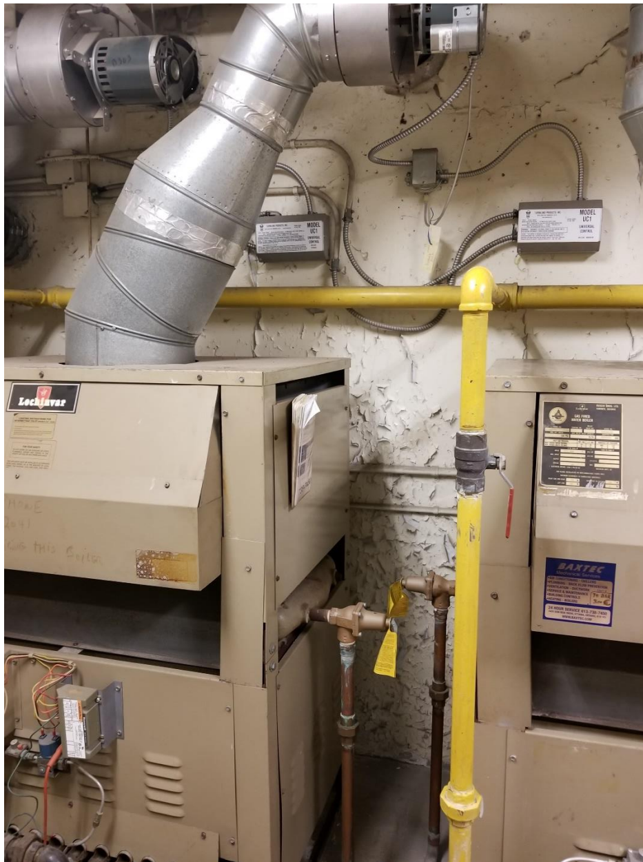
Photo 2: Beige paint applied to walls of the boiler room, contains 1,320 ppm lead (DST Sample LP-02).
