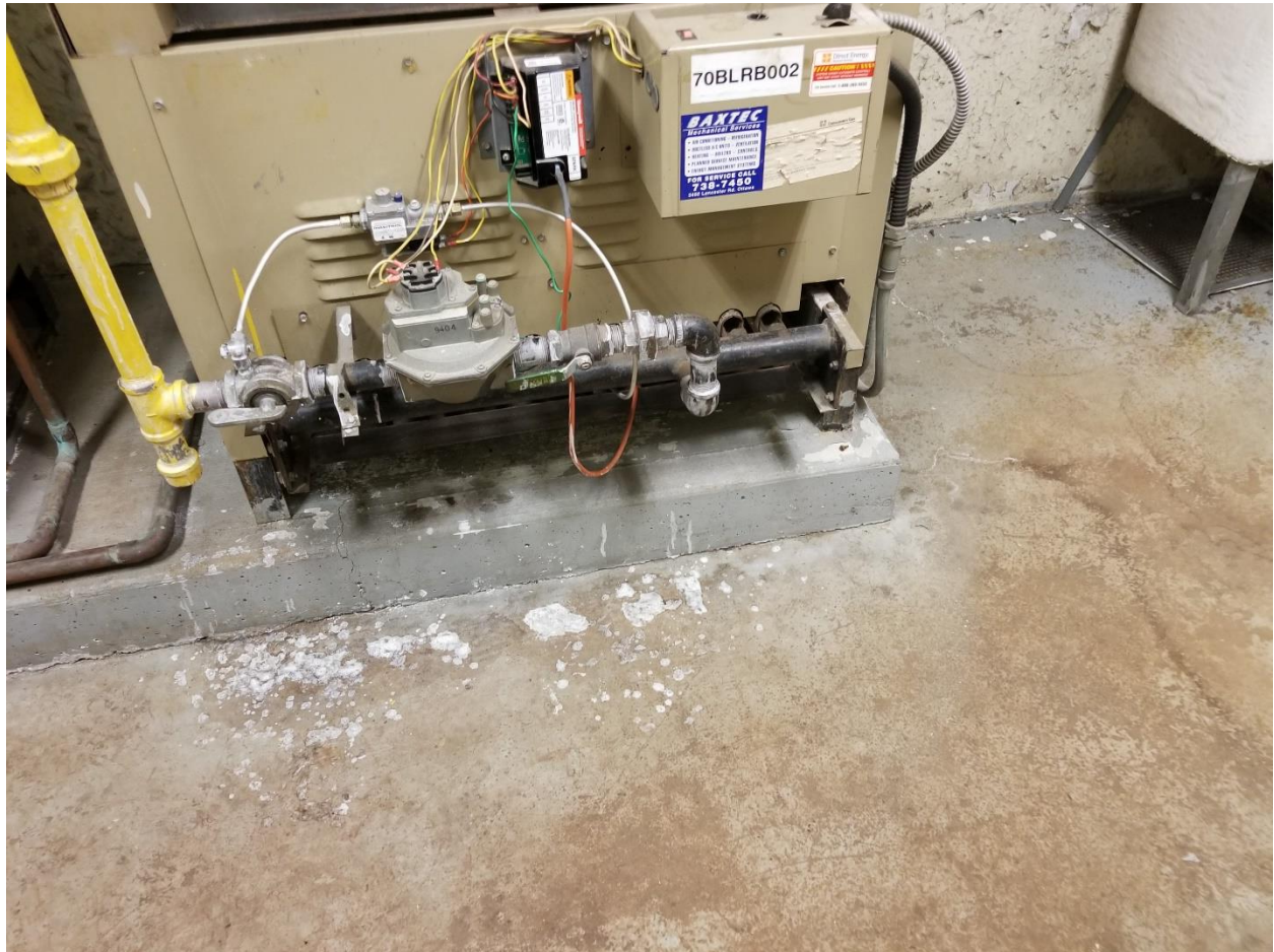
Photo 1: Grey paint applied to the floor of the boiler room, contains 949 ppm lead (DST Sample LP-01).
