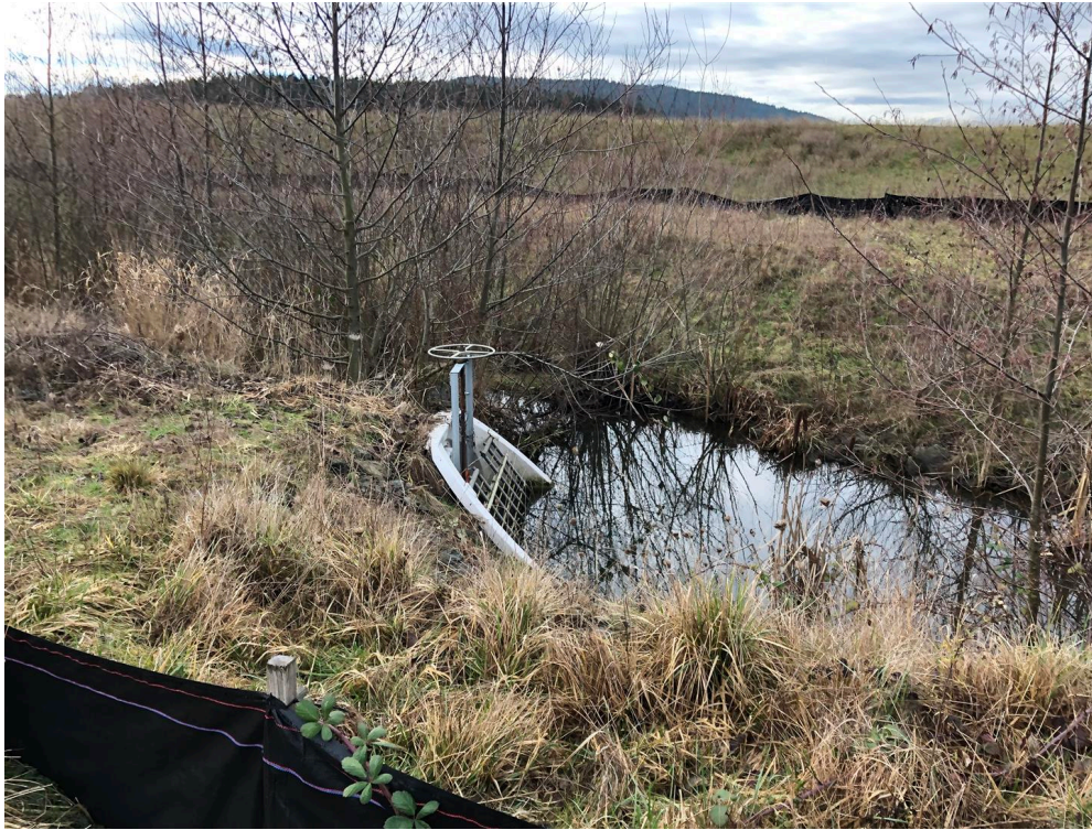
Photo 1: Flow controller at upstream end of Reach 1A, looking south.
