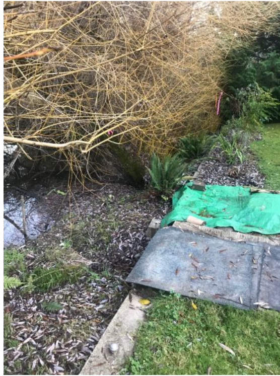
Photo 7: Concrete retaining wall at property line along south boundary of lower KEL,SET (Reay) Creek Pond, looking east.
