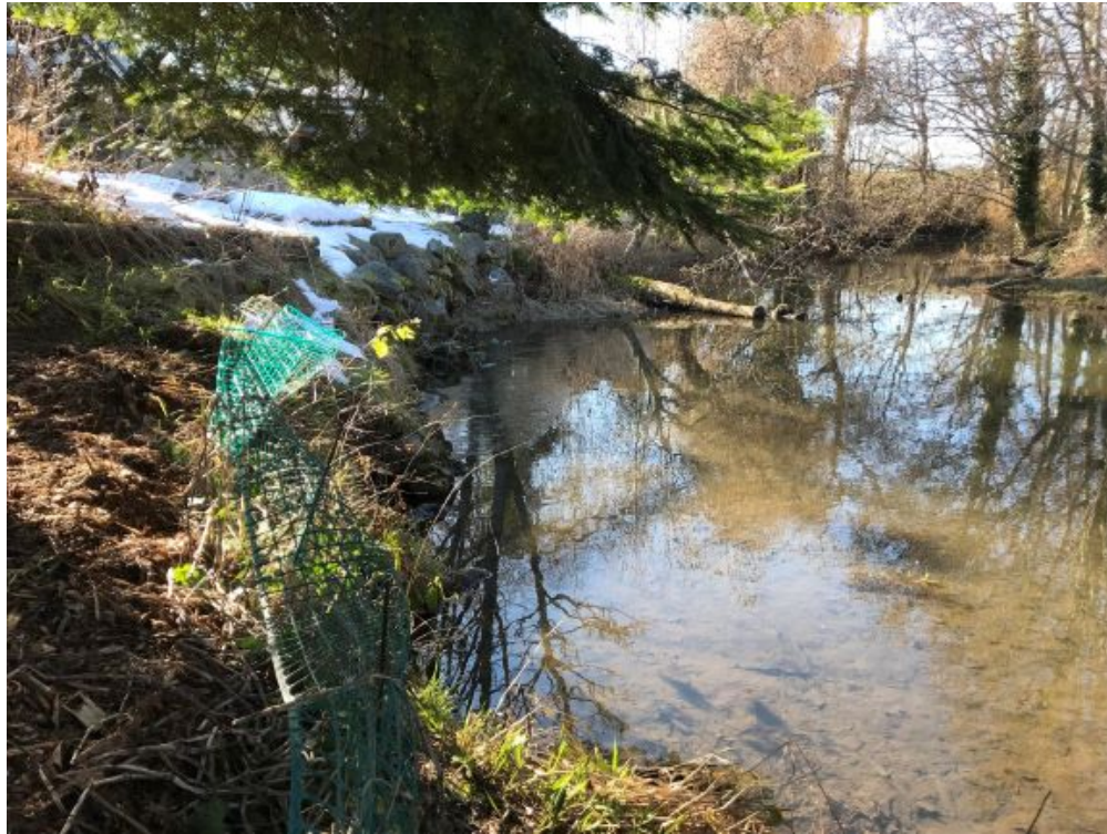
Photo 27: Shallow water depths and accumulated sediment near upstream end of pond along south bank, looking northwest.
