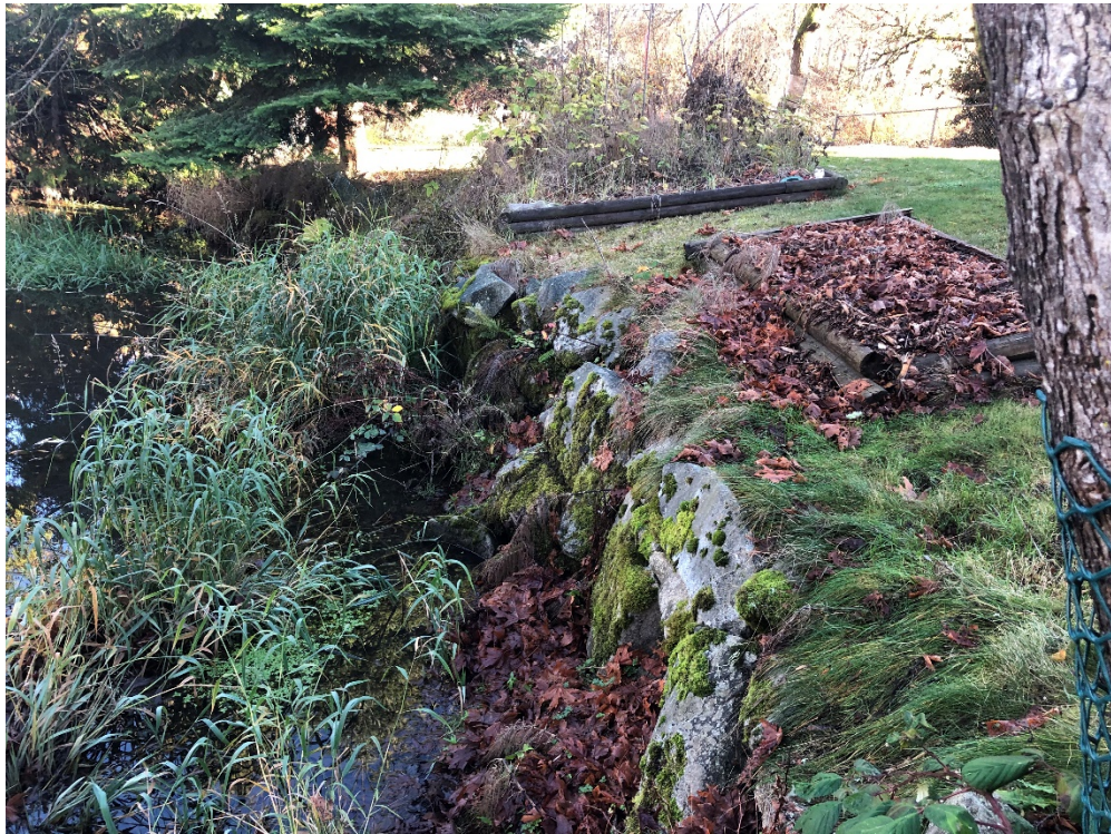
Photo 20: Rock wall along the southwest perimeter of KÉL,SET (Reay) Creek Pond at the edge of residential properties, looking southeast. Structures extend beyond property line in select areas.
