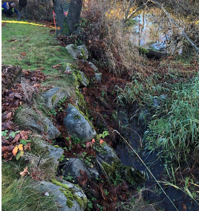
Photo 21: Rock wall along the southwest perimeter of KÉL,SET (Reay) Creek Pond at the edge of residential properties, looking northwest. Structures extend beyond property line in select areas.
