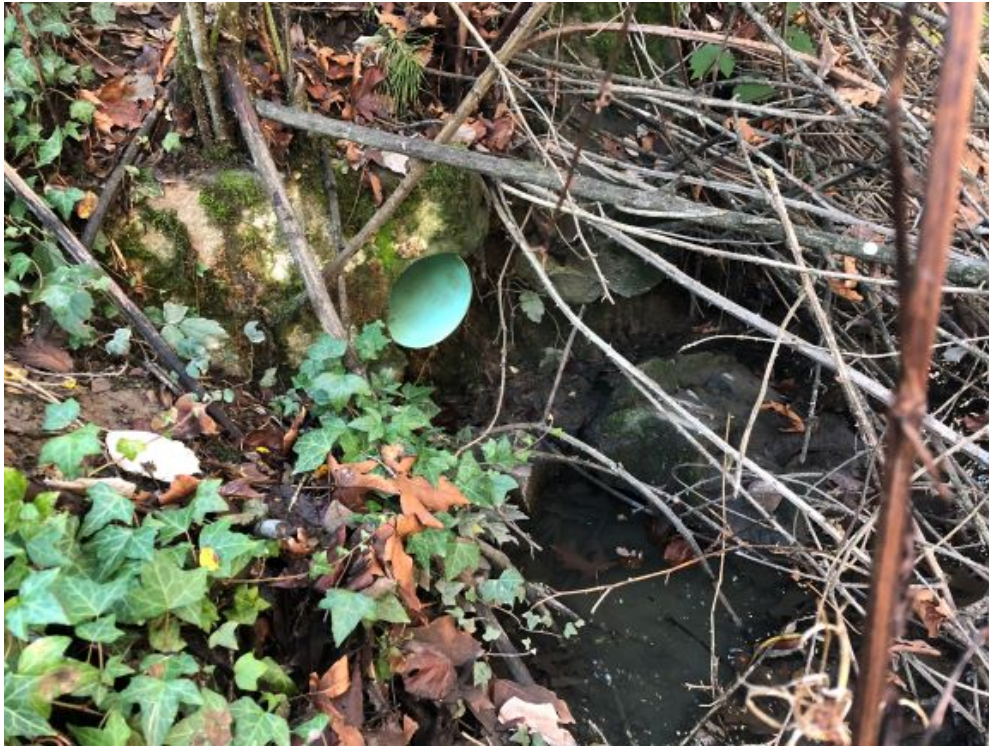
Photo 19: Local property storm drainage outlet along south side of KÉL,SET (Reay) Creek Pond at the edge of residential properties.
