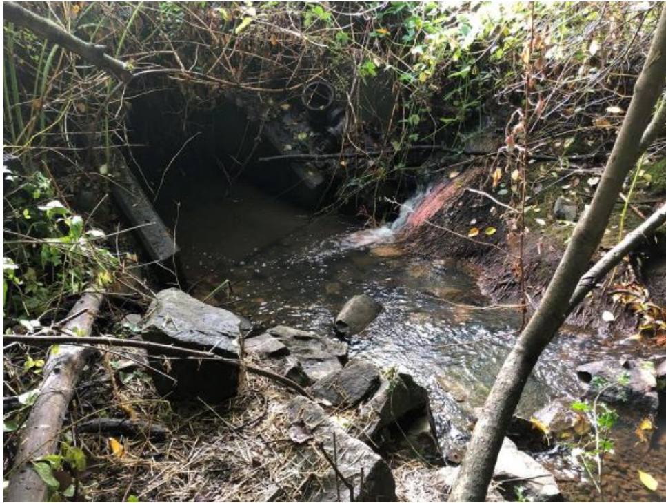
Photo 37: Culvert entrance of KEL,SET (Reay) Creek upstream of Canora Road, looking south.
