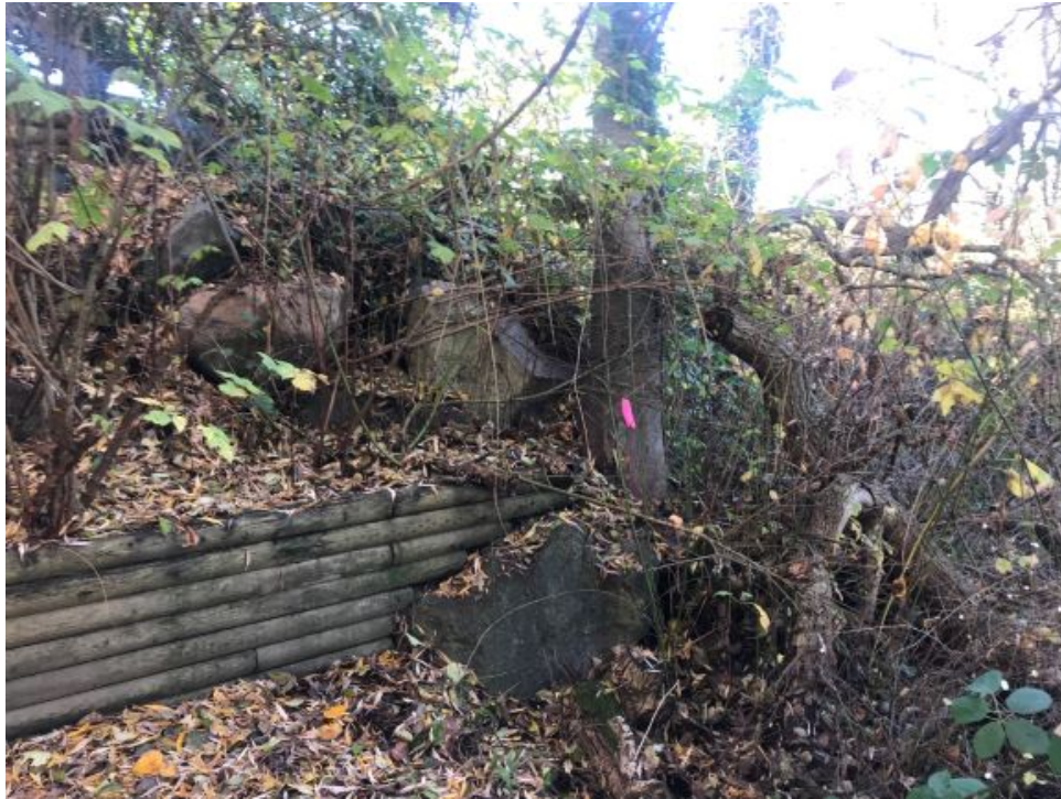
Photo 25: Wooden retaining wall on private property adjacent to upper section of pond along south bank, looking west.
