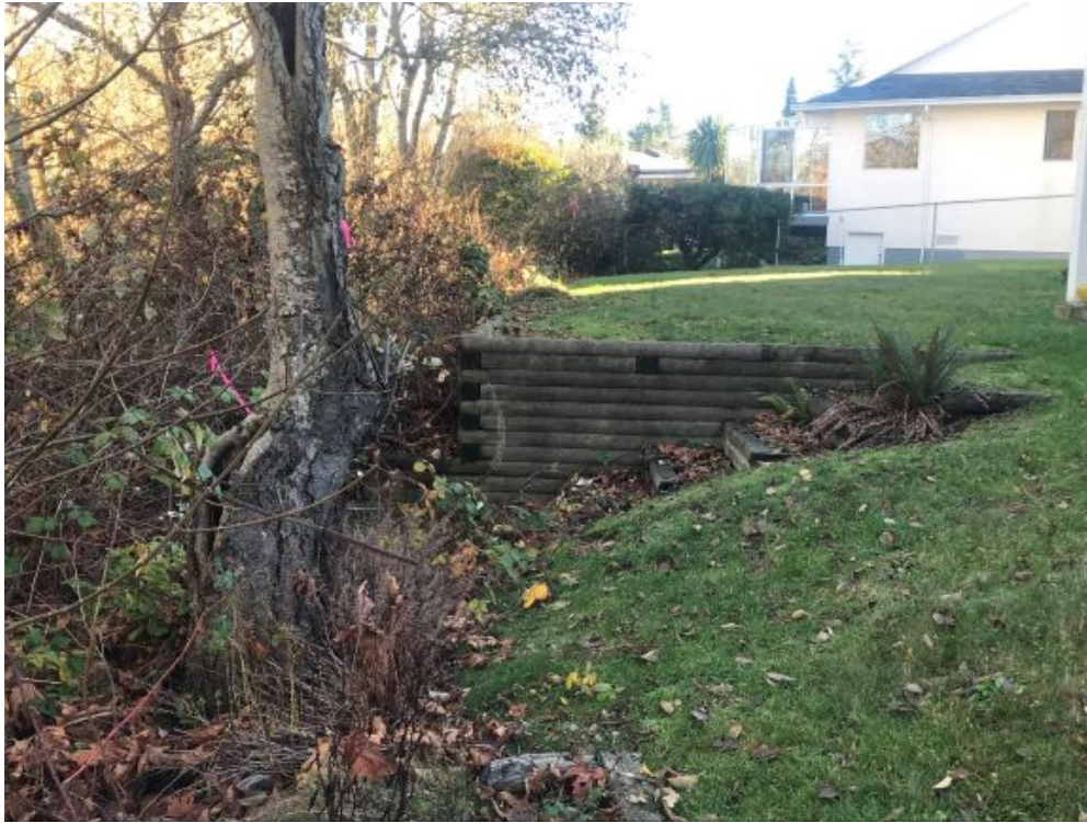
Photo 17: Wooden retaining wall and trees along south side of KÉL,SET (Reay) Creek Pond at the edge of residential properties, looking southeast.
